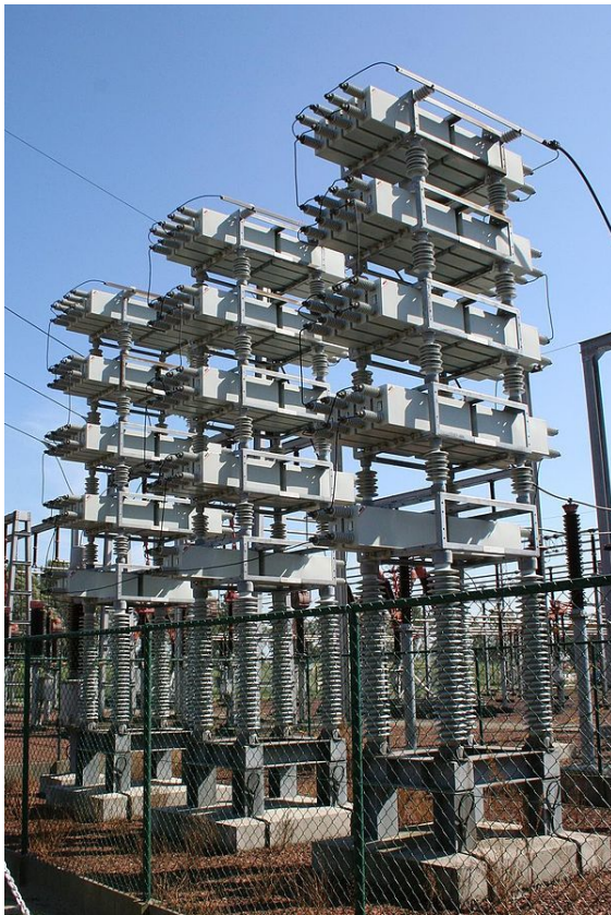
A high-voltage capacitor bank used for power factor correction on a power transmission system
