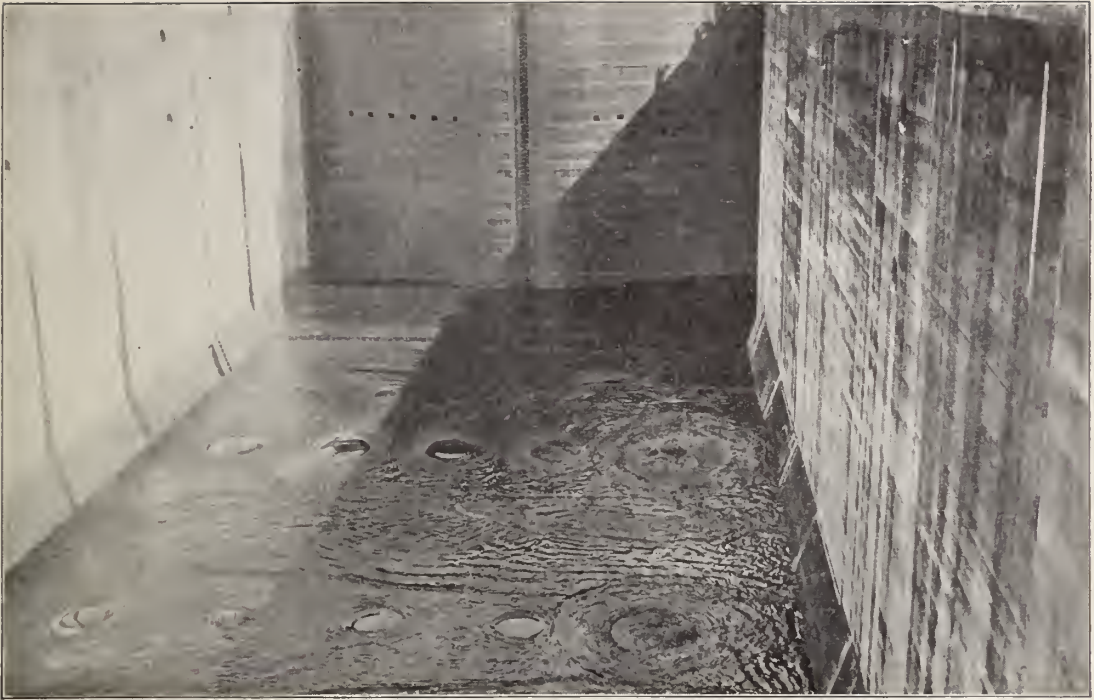
Turning water into the lock chamber through culvert openings in the floor—partial flow.
