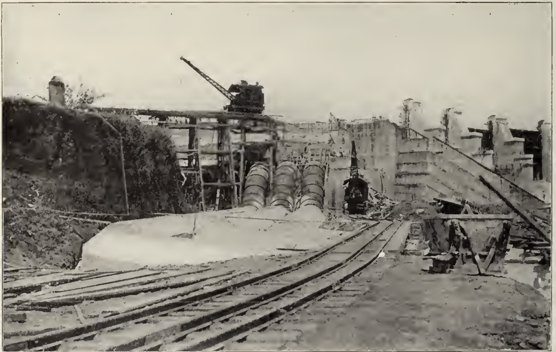
The penstocks at the new hydroelectric station at Gatun spillway, which, by furnishing the water to the turbines from Gatun Lake, will drive the machinery at all the locks.
