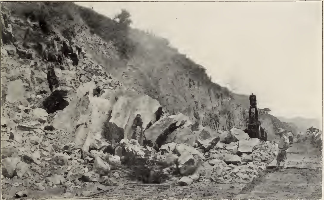
Steam shovel 218 buried under fall of rock, west side of Canal, near Las Cascadas. This shovel was working on the bottom of the canal when destroyed, May 31, 1912. Several steam shovels have been destroyed in this manner and a number of men injured and killed.
