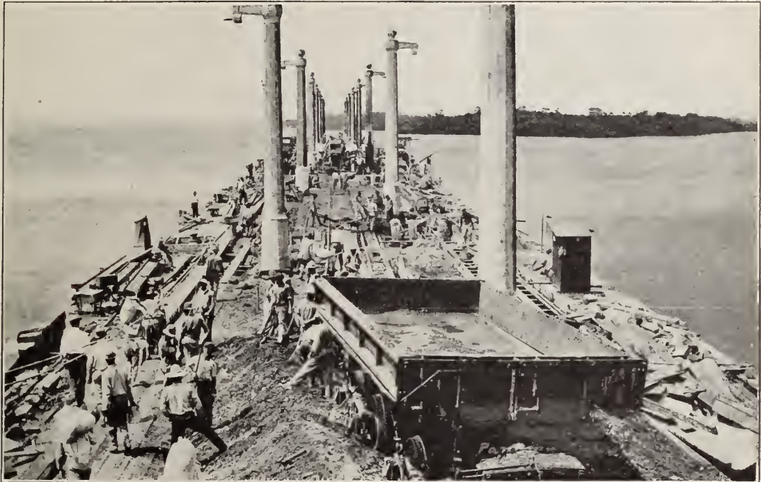
Sunday scene on south approach wall at Gatun Locks. In order to finish a piece of work within a given time, it was frequently necessary to work the men the full seven days.
