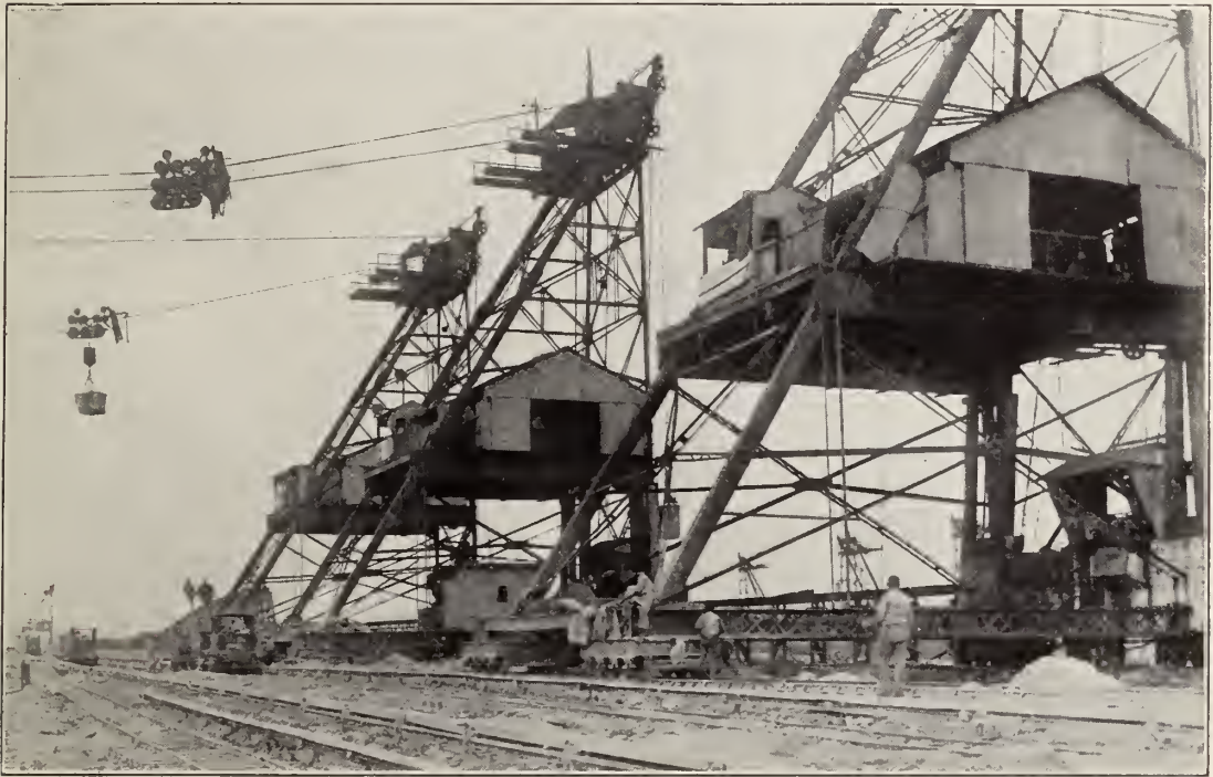
Eight of these cableways, four on each bank, were used to place the concrete in the lock walls. They consisted of steel towers, 85 feet high, operating on their own tracks, and supported cables, which carried the concrete buckets back and forth.
