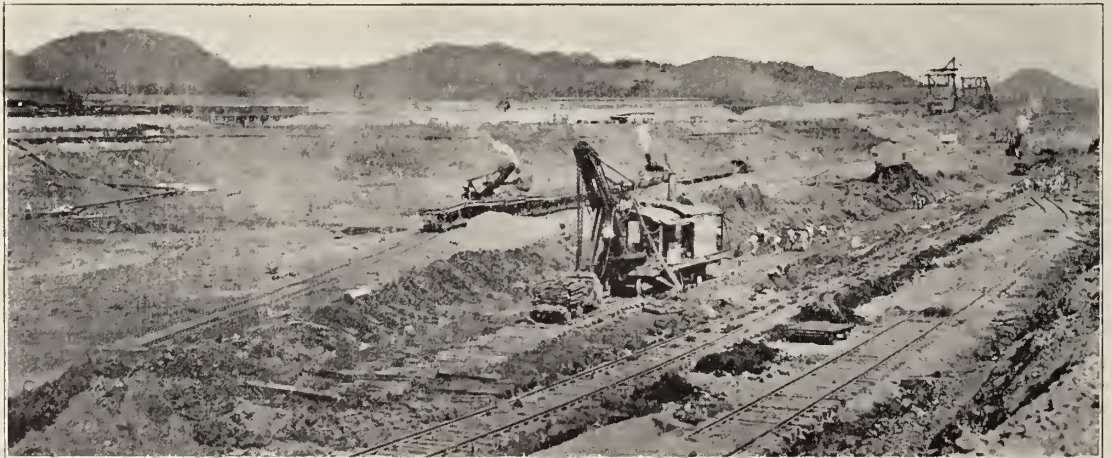
Excavating for lock site, Miraflores. Millions of cubic yards of material had to be excavated before the locks were built.
