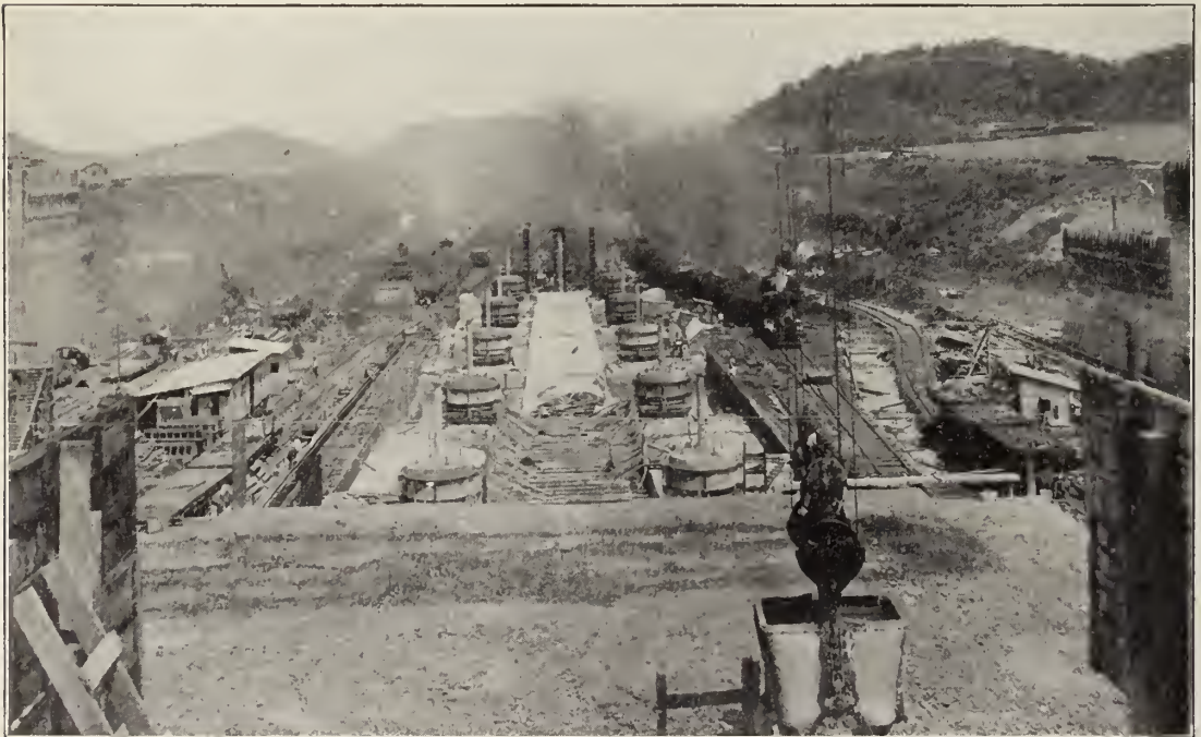
Installing the cylindrical valves for the control of the flow of water in and out of the locks. The water control system of the locks consists of rising stem or Stony gate valves, and cylindrical valves. The rising stem valves govern the flow of water in the side wall culverts, and the cylindrical valves govern the flow of water in the center wall culverts.
