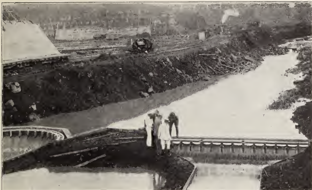
Experimental spillway at Gatun Dam. Like all other important features of the Canal work, experiments were made to ascertain the proper method of constructing the work.
