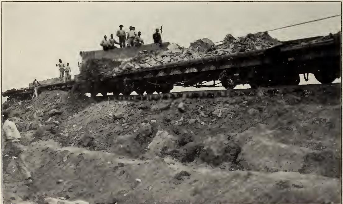
An unloading machine at work on a train of Lidgerwood flat cars. The unloader, actuated by steam from the locomotive, pulls the plow by a steel cable which coils around a drum. A man rides the plow, and signals the movements with a flag.
