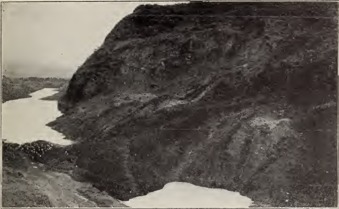
Close view of Cucaracha slide. The lagoon in the foreground was formed by another part of the slide blocking the Canal about where the picture ends. In the distance may be seen two points projecting into the Canal. These were the toes of the slides on the east and west banks at Culebra, which moved some distance after water was admitted to the Cut.
