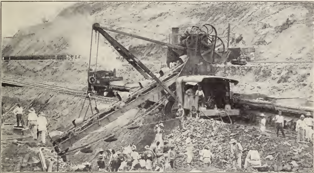
A French excavator opening a pioneer trench in the south end of the Cut. This was the best known method of excavating in that day.
