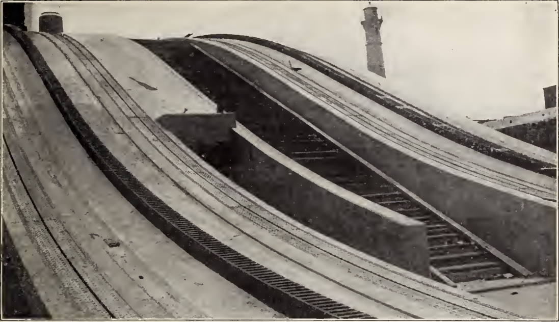
Section of lock wall showing the rack rail over which the towing locomotives travel.
