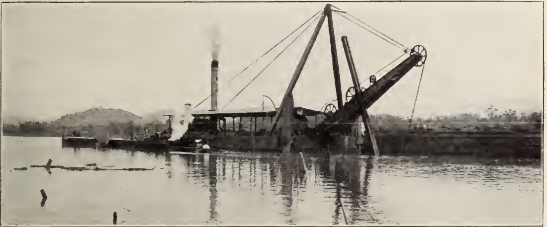
A dipper dredge at work in the Canal. The material is dumped into the barge along side the dredge, and when full the barge is towed out to sea and emptied.
