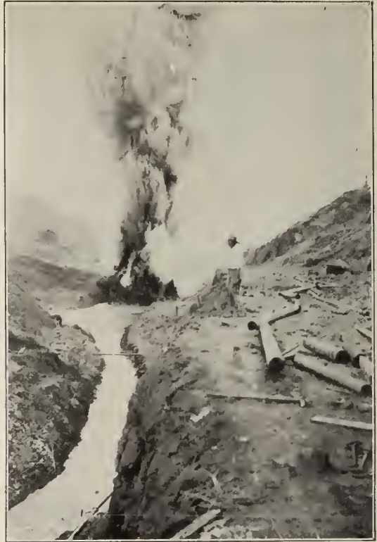
Shooting off a blast in connection with the work of cutting a ditch through Cucaracha slide for the passage of water.
