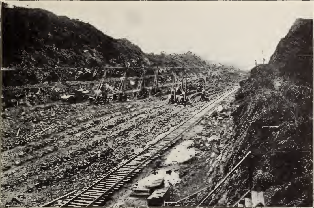
The Cut at Bas Obispo looking south June 30, 1910. The greater part of the excavating in this section had to be done through solid rock, and thousands of pounds of dynamite were used. It was in this section that the premature explosion occurred in 1908.
