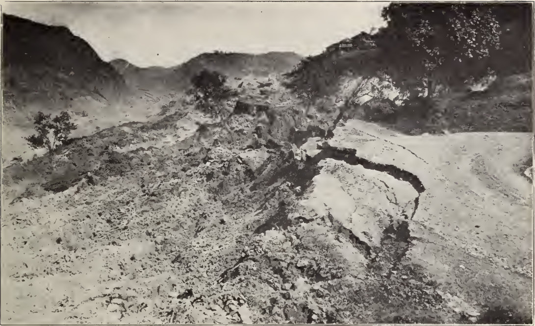
Many slides have developed during the latter part of the Canal work which have caused a great deal of damage and the excavation of much more material than was formerly estimated. This view shows a break on the west bank at Culebra which encroached on the village of Culebra to such an extent that it was necessary to move a large number of buildings, including the hotel and Y. M. C. A. Clubhouse.
