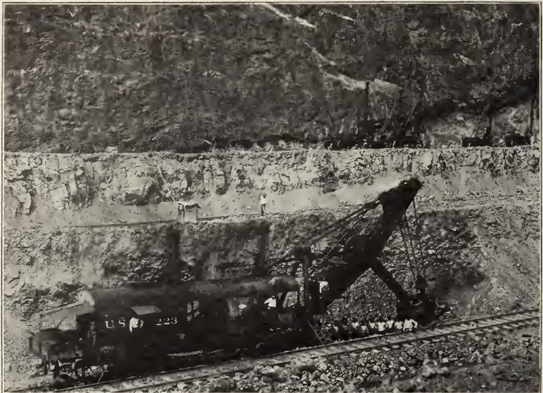
Ninety-five ton steam shovel at work in Culebra Cut. One hundred steam shovels have been used in the Canal work. Culebra Cut is a term officially applied to that part of the Canal between Bas Obispo on the north and Pedro Miguel on the south, a distance of about nine miles. The width of the Cut is 300 feet at the bottom.
