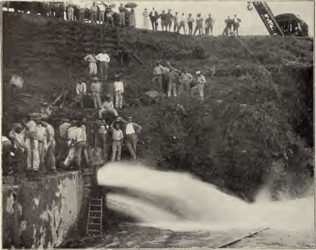
Letting water through Gamboa Dike into Culebra Cut. Two of the 24-inch pipes are shown in this picture. Six of these pipes were opened ten days before the Dike was blown up, allowing the Cut to become partly filled, so there would not be such a rush of water when the Dike was destroyed.
