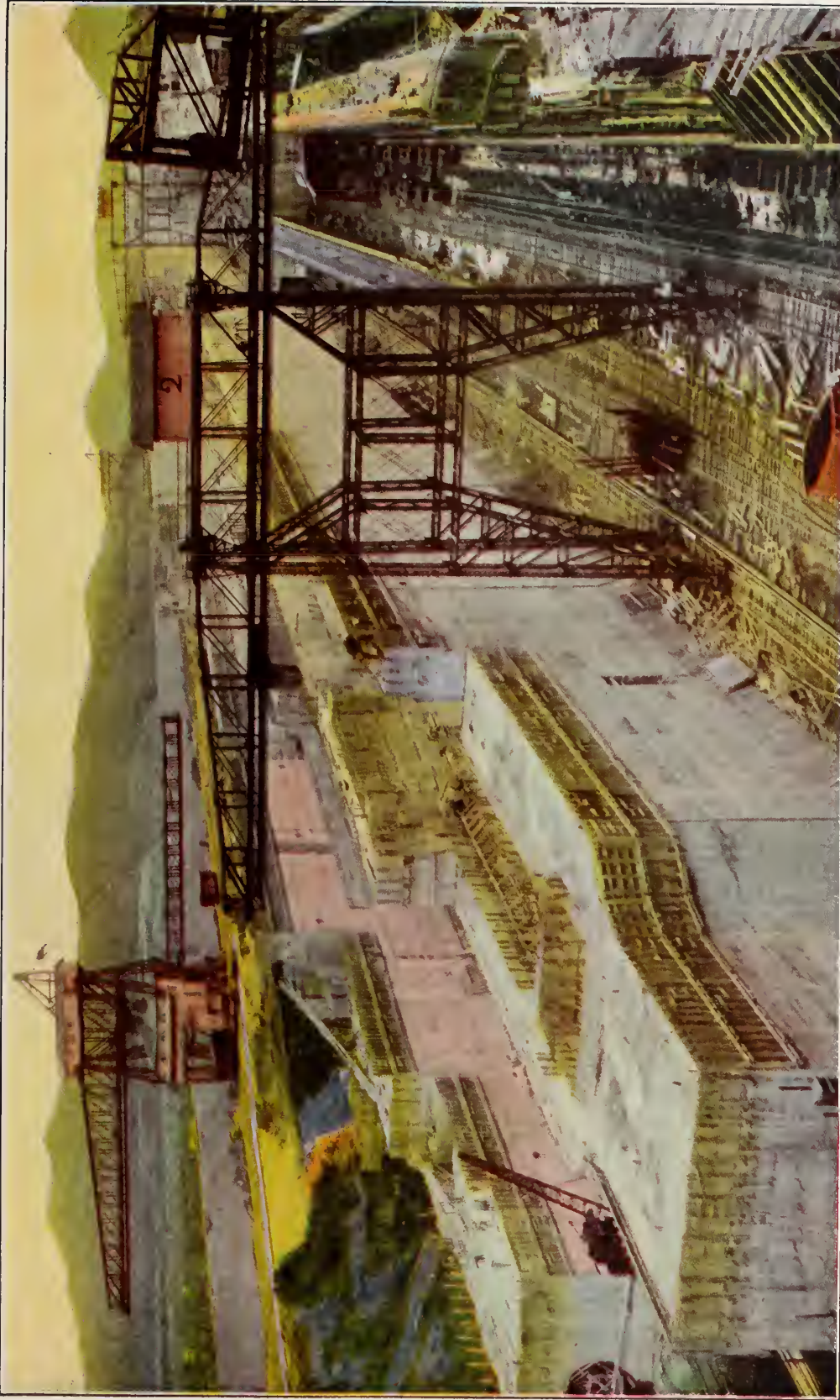
A comprehensive view of one of the great locks of the Canal under construction, where the largest concrete monoliths in the world have been built. One is almost bewildered by the tremendous machinery of the work—the enormous Berm and Chamber cranes with their almost uncanny air of intelligence towering over the scene with their interlaced-ironwork arms extended above the cement walls which they are constructing.
