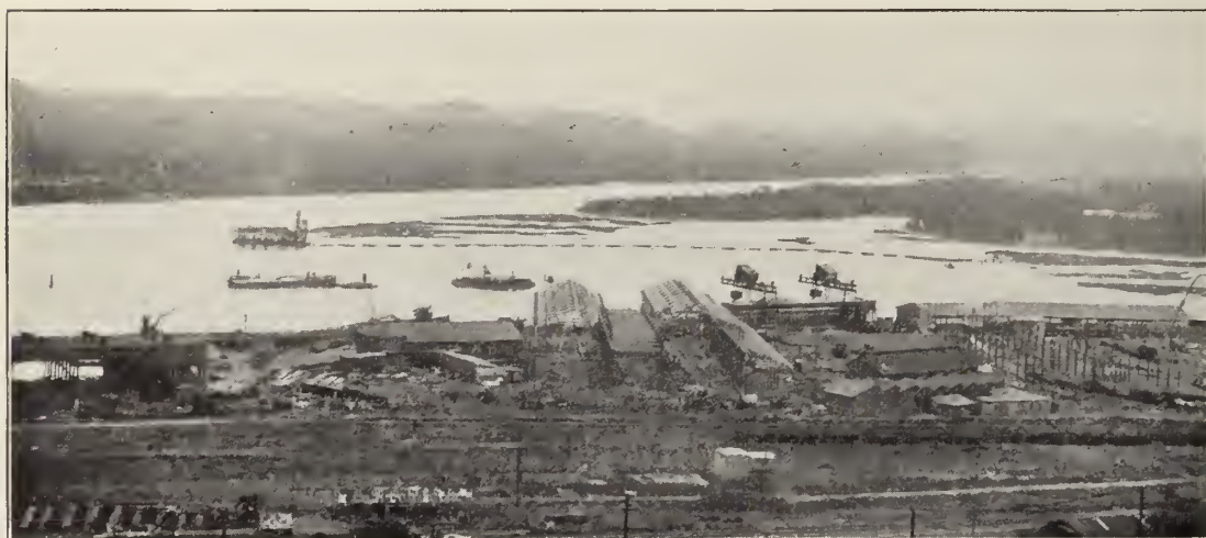
Excavation in the immediate foreground is for the new Balboa dry dock. Buildings under construction are the permanent shops. Beyond where the dredge is working will be the Balboa ship basin.
