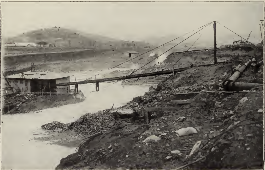
After the material has been loosened and washed into the sumps, centrifugal dredging pumps, shown here, force the material to the desired destination. Many acres have been reclaimed near Corozal by utilizing this excavated material.
