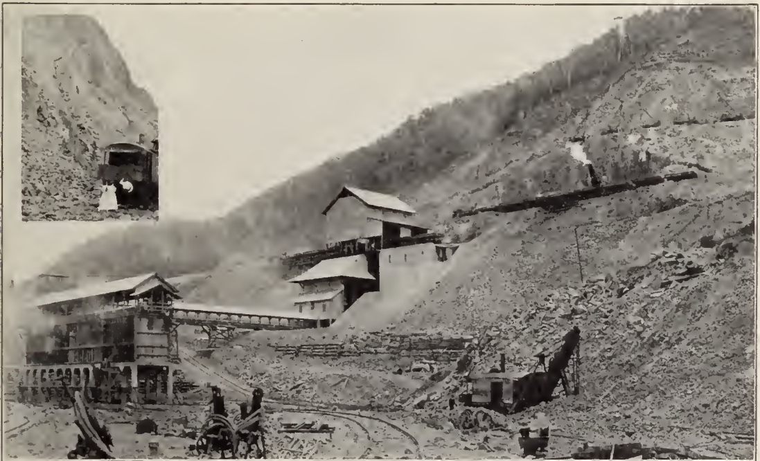
Ancon rock crusher plant and quarry, between Panama City and Balboa, where the crushed rock was obtained for the concrete used in the Pacific locks. The side of the hill has been literally eaten away to secure the large amount of rock required.
