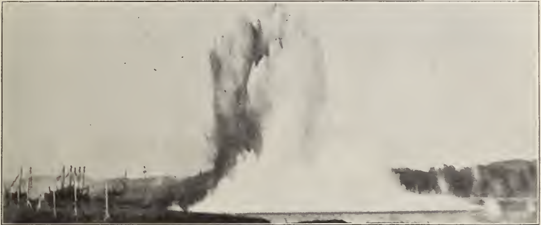
A subaqueous blast in progress in the Pacific entrance to the Canal. As high as 10,000 pounds of dynamite are shot off in a single blast of this kind.
