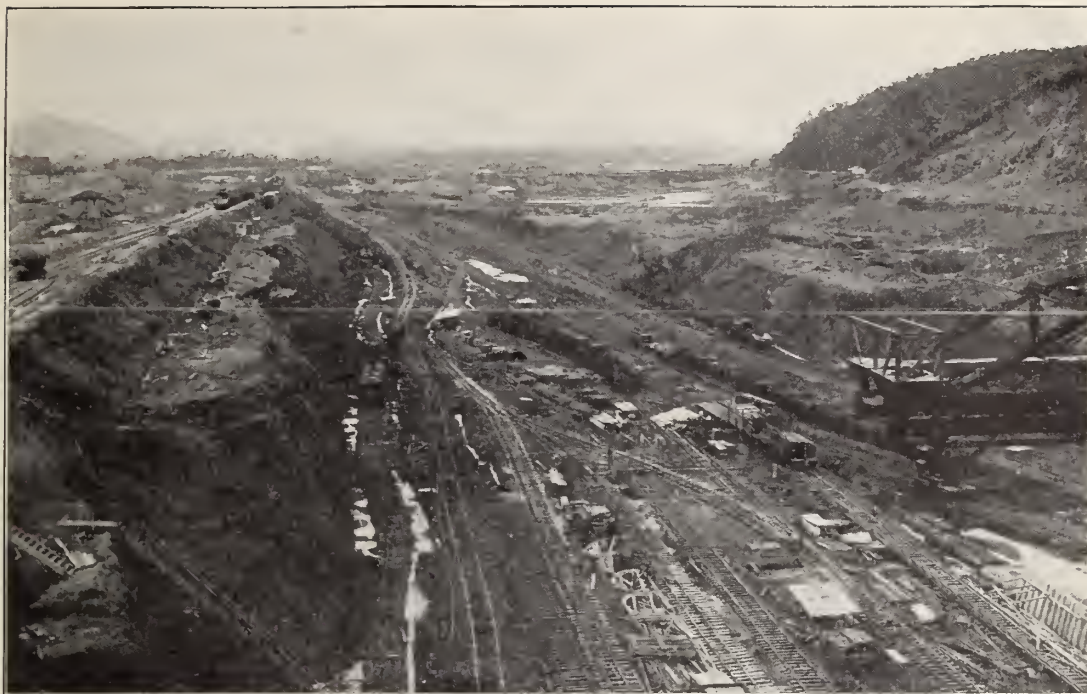
Excavating in the Canal from Miraflores Locks to the sea. This is the section of the Canal that was filled by the blowing up of the last dike at Miraflores, shown on the previous pages.
