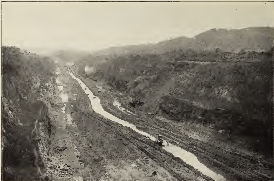
Completed section of Culebra Cut looking north from Cunette. Steam shovels are excavating in slide material. Bottom is to grade.
