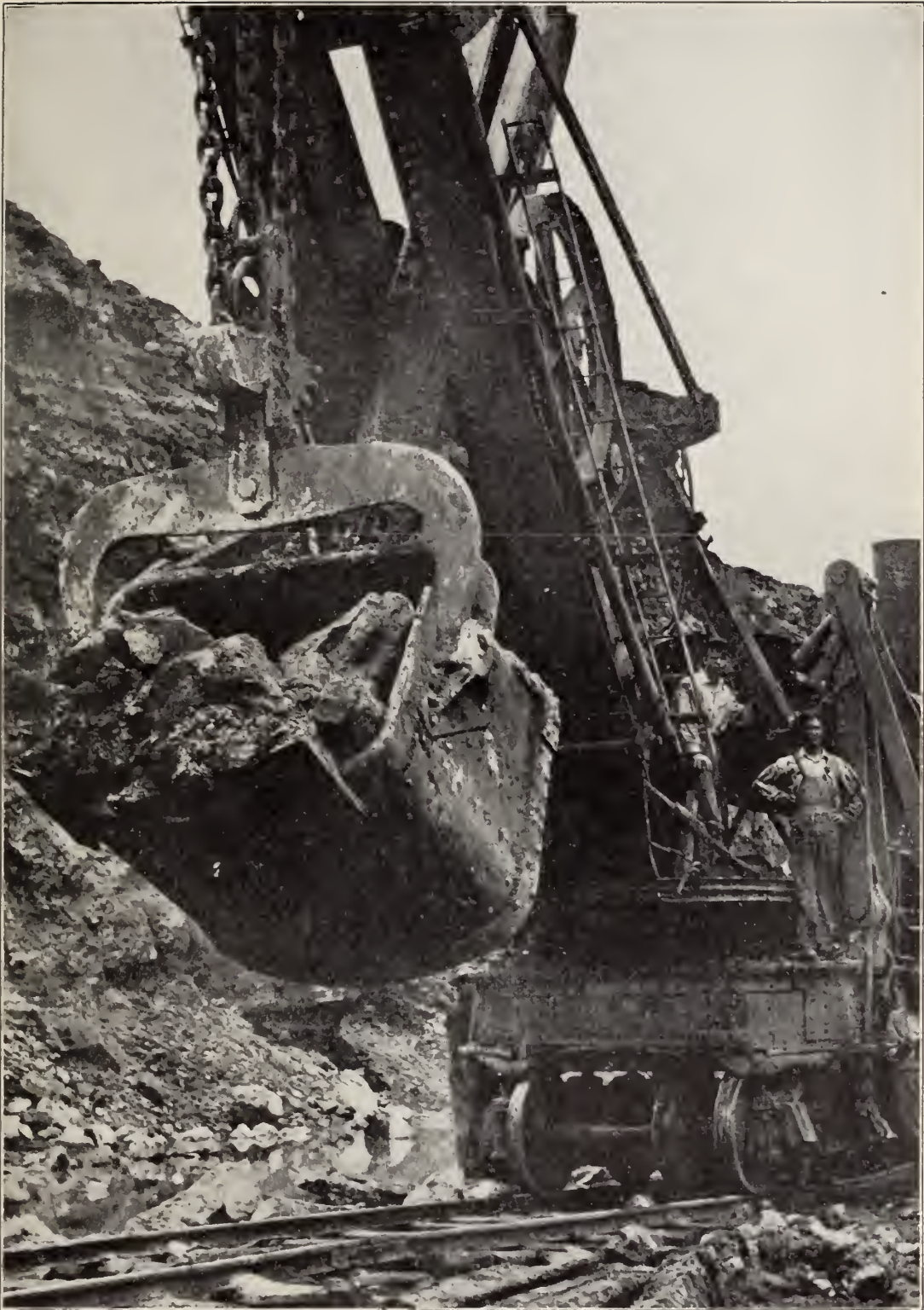
Last dipperful of dirt taken out of Culebra Cut by Steam Shovel No. 226.
