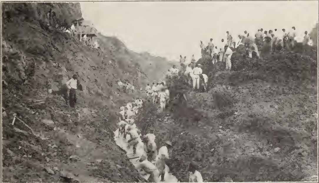
Closer view of trenching operations at the slide. Workmen engaged in trying to keep a trench open in the spongy mass to let the water from filled section through. This proved to be a most discouraging task, for the material moved about as fast as dug out. Two workmen were drowned while these operations were in progress.
