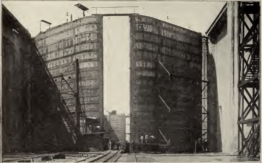
Close view of completed gates at Gatun Locks. There are 46 gates in the locks which aggregate 58,000 tons in weight, and if placed end on end would make a tower about one and one-fifth miles high. The author was standing on the lock floor between the partly closed gates when this photograph was taken.
