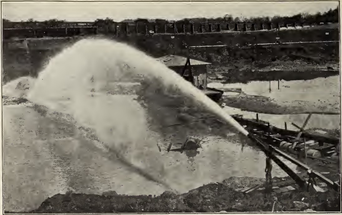
Part of Miraflores lock site and the Canal channel to the south of it were excavated hydraulically. This view shows one of the hydraulic pumps forcing the water through pipes, fitted with monitors, with a pressure of 130 pounds per square inch at the nozzle, which washes the material into pits or sumps.
