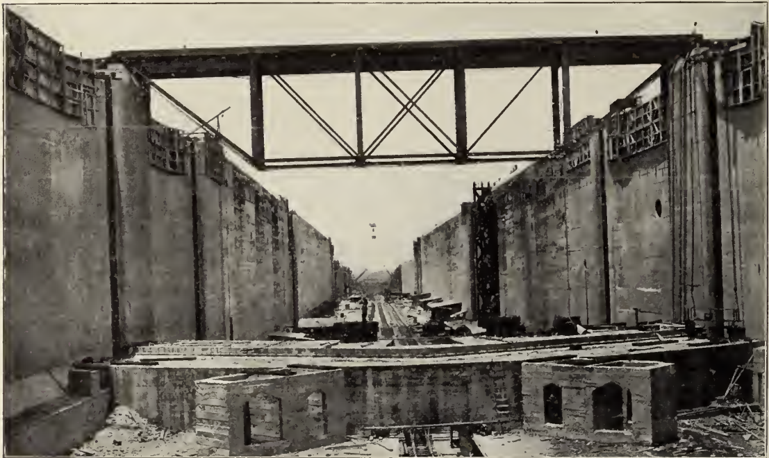
Completed sills from the lock gates. These sills, built of steel and concrete, form foundations on which the gates rest.
