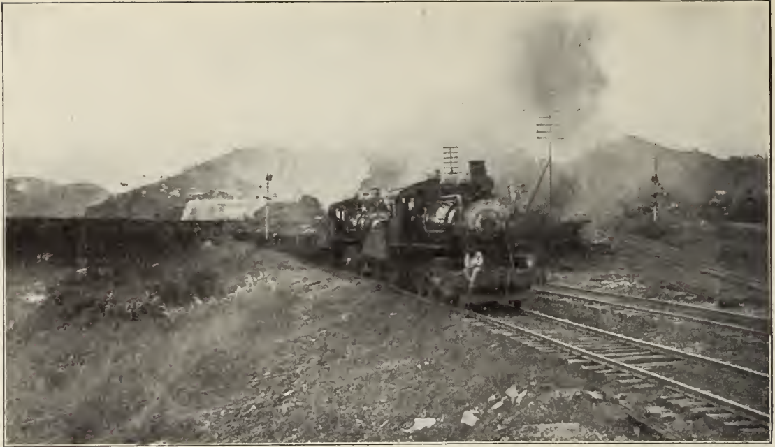
A loaded train of Lidgerwood flat cars coming out of the Cut at Pedro Miguel. During the latter part of the excavation, the Cut was at such a depth below the surrounding levels that long inclines had to be built, up which the dirt trains were pulled by two and three locomotives.
