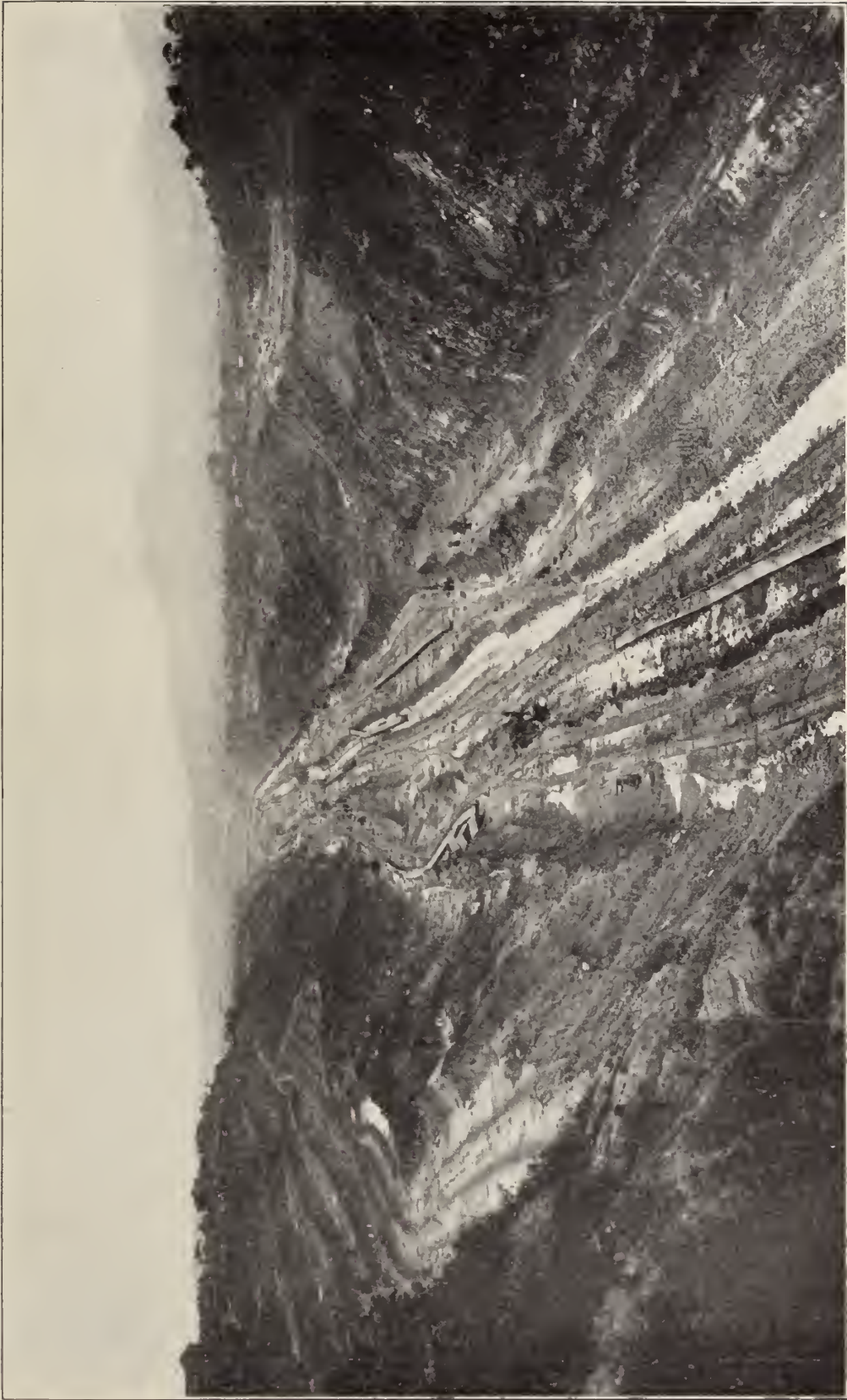
Culebra Cut near Culebra village, as it appeared October 1, 1912. You will note in the picture the manner of terracing the sides of the Cut. This was done as a preventive measure against the slides.
