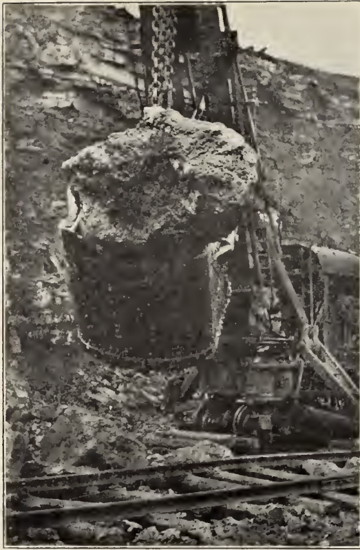
Next to the last large rock delivered by Steam Shovel No. 226, Engineer Geddes; Craneman Hudson.
