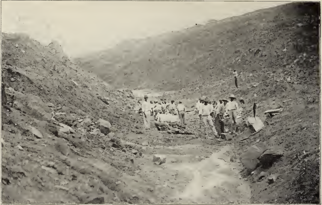
This shows where the slides on either bank have encroached upon the prism of the Canal to such an extent as to almost effect a closure.
