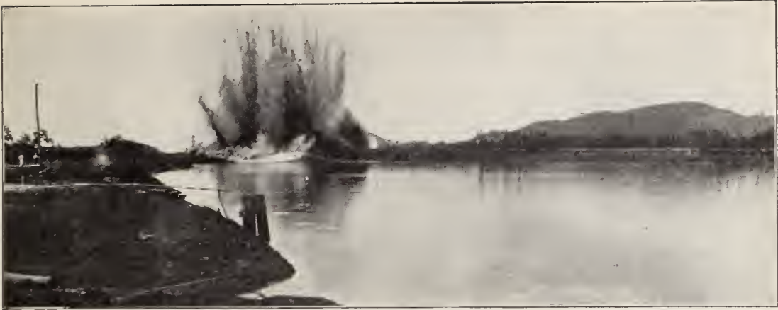
Blowing up the first dike at Miraflores on May 18, 1913. This let water into a completed section of the Canal about 1,000 feet long.
