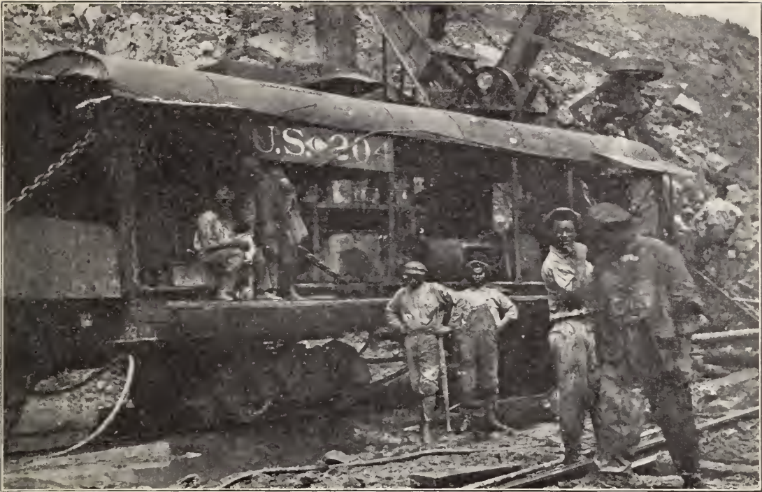
Steam Shovel No. 226, which loaded last dipperful of dirt on last train out of the Cut.
