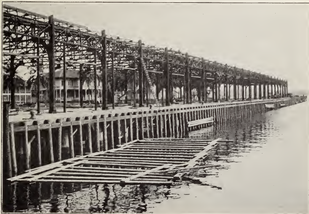
New dock No. 16 at Colon under construction. Part of the Cristobal terminal system.
