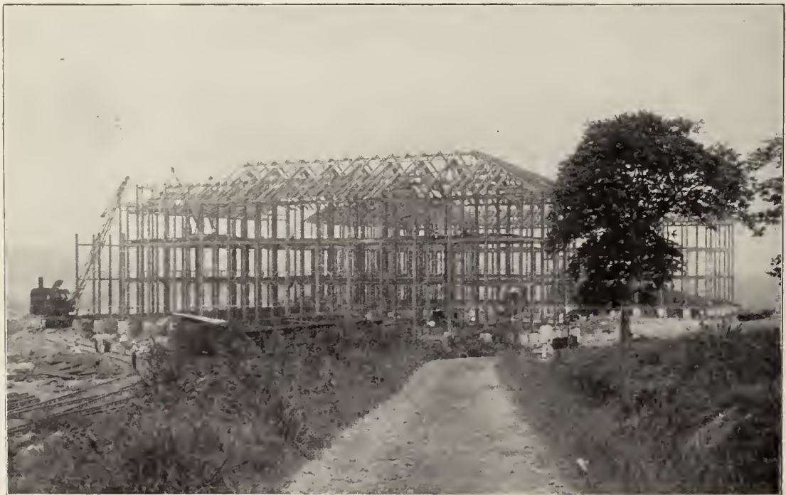
Permanent administration building on west side of Ancon Hill under construction. Overlooks the site on which the permanent town at Balboa will be laid out.
