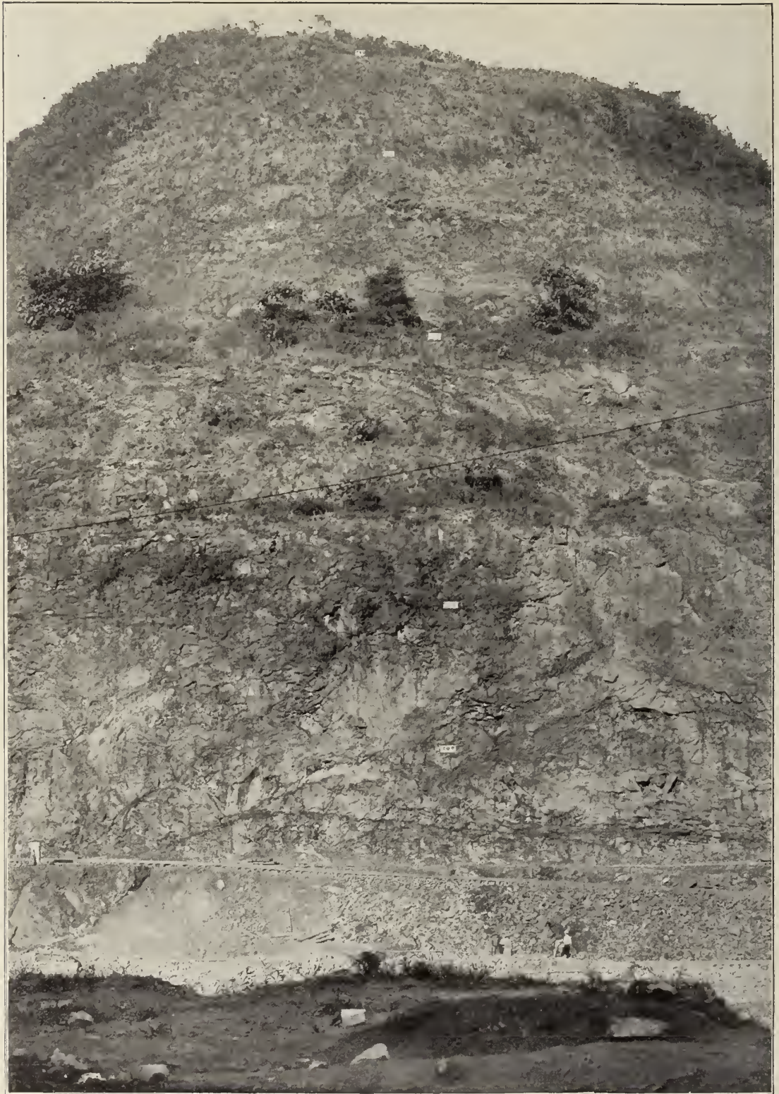
The side of the Cut at Gold Hill, where the deepest cutting was done. When this photograph was taken the steam shovels had 30 feet further to go at this point.
