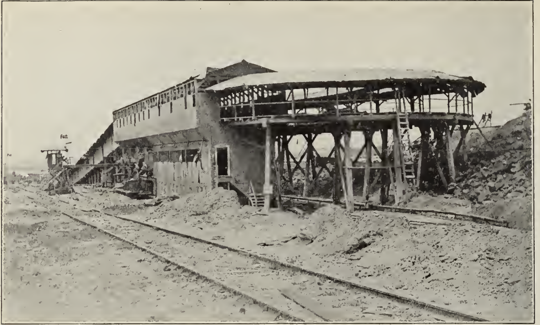
A general view of the main concrete mixing plant at Gatun Locks, which houses a battery of eight 2-cubic yard mixers. Rock and sand were carried to the mixers by an electric railroad running underground to a point beneath the storage piles. The finished product was carried to the lock site by a surface electric railroad.
