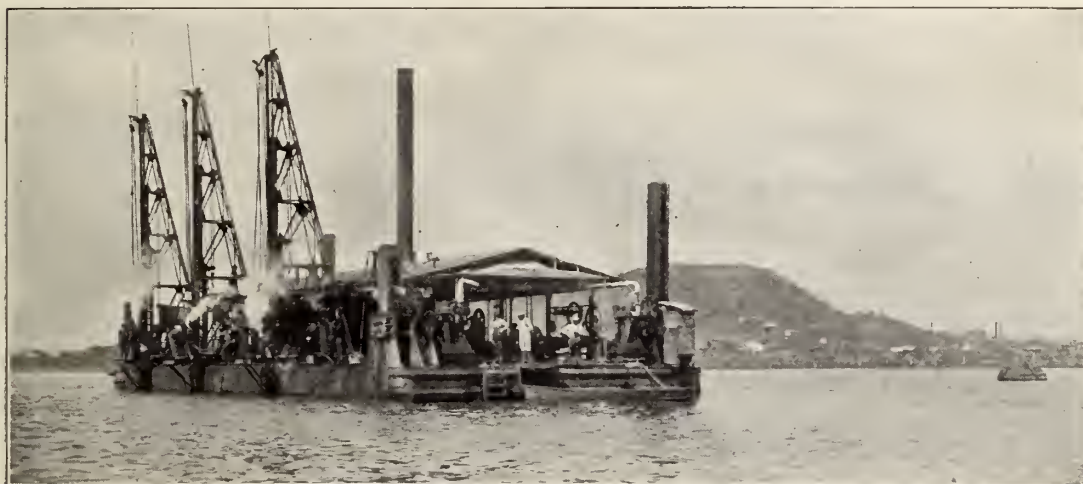
In dredging operations, subaqueous or under water blasting is employed. Drill boats, like the one in the picture, sink the holes in connection with this work.
