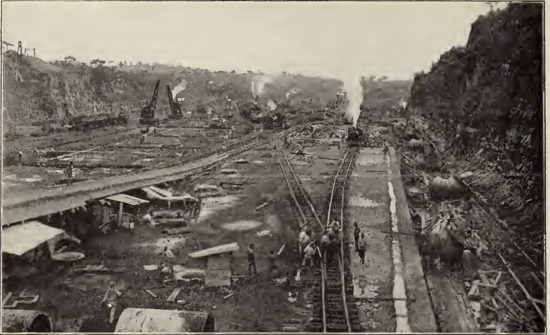
The beginning of concrete work at Gatun Locks. Laying the floor and installing the lateral culverts. The circular holes in the floor are to admit the water to the locks, and to empty them. The floor varies in thickness from 13 to 20 feet of solid concrete, according to the character of material underlying it, and is anchored by steel rail to a depth of 10 feet.
