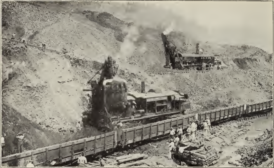
Steam shovels working in the slide at Cucaracha. This slide showed evidence of activity as far back as 1887, when the French were at work on the Canal, and has been a source of trouble ever since.
