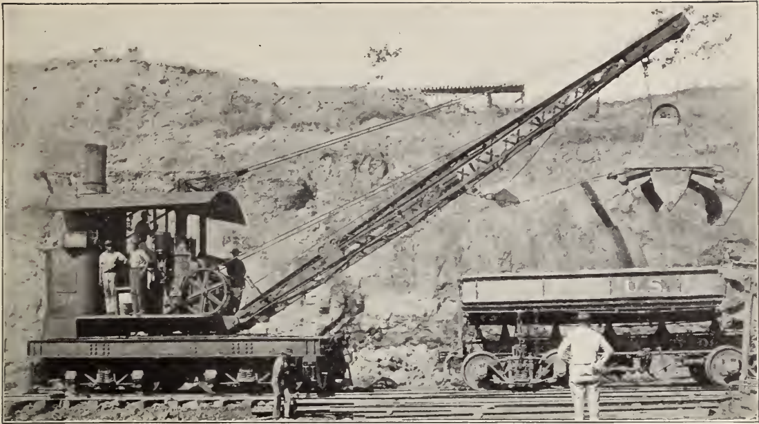
Locomotive cranes were a useful adjunct to the Canal work. This one is operating a clamshell bucket, so named from its resemblance to the bivalve.
