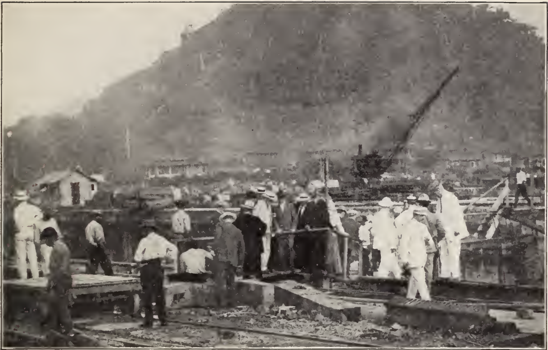
Visitors inspecting the work on the locks at Pedro Miguel. Thousands of tourists have visited the Canal during the last few years, including people in every walk of life from the States, as well as committees from almost every nation on the globe.
