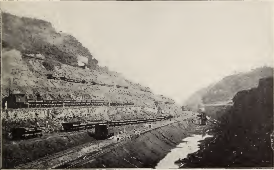
The Cut as it appeared in 1904 when the Americans began the work. Contractor's Hill on the right; Gold Hill on the left. Note the succession of benches, lying one above the other. The Americans have followed this same method in excavating.
