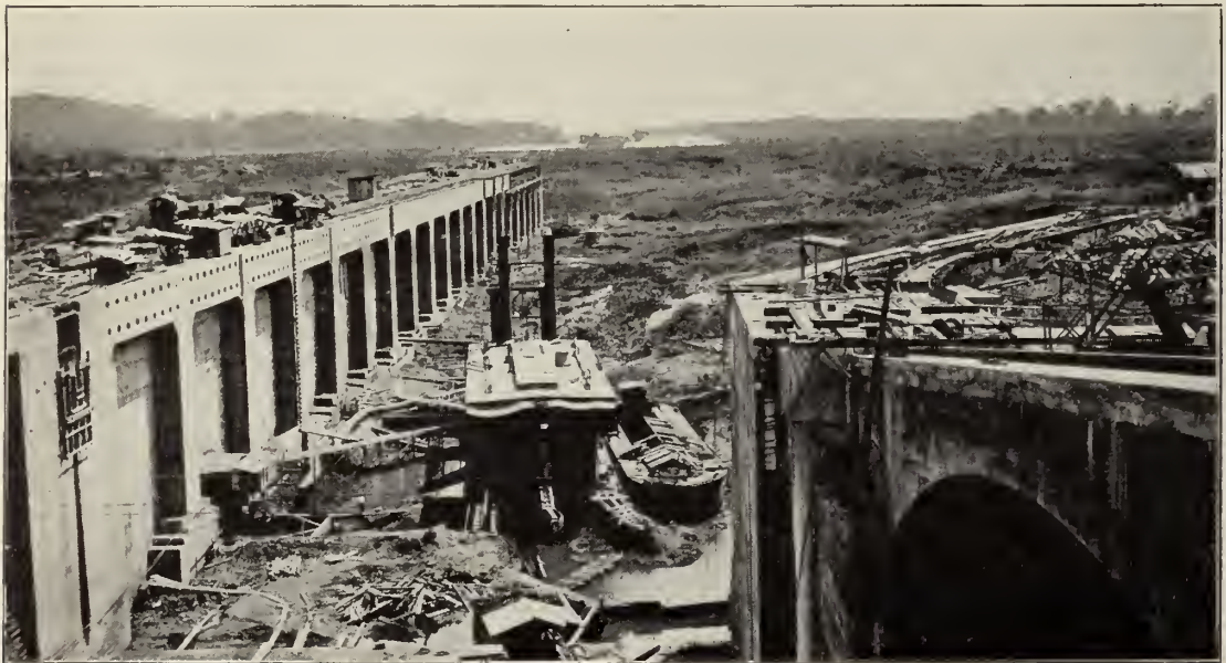
Section of the north guide wall at Gatun Locks under construction. This was one of the most difficult pieces of masonry work in the whole job. The greater part of its length of 1,000 feet rests upon piles driven to solid rock. To the right is seen the east wing wall of the locks.
