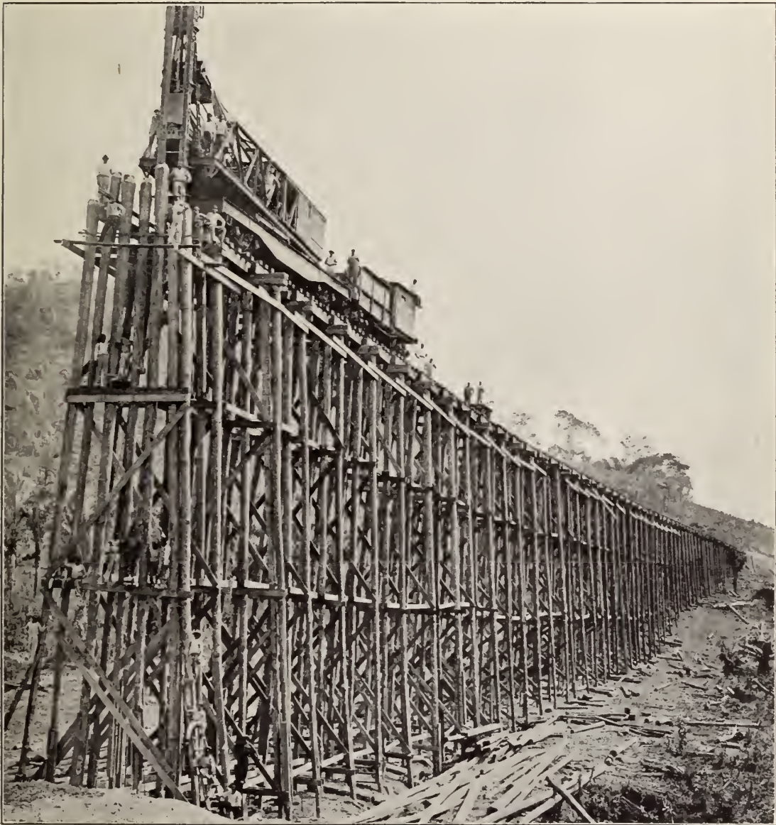
High trestle for embankment fill. The new line was built on a 95-foot level and across the lowlands of the Gatun Lake region a number of long and high trestles for embankment fills, some of them 90 feet high, had to be built.
