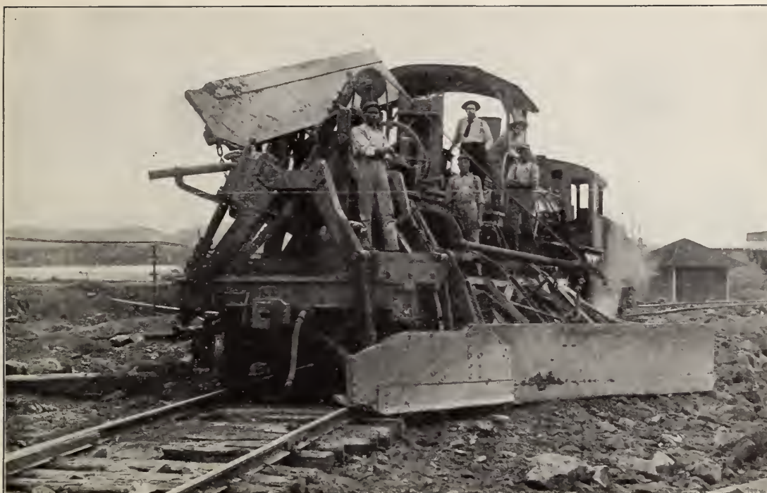
An earth spreader at work. After the cars have been unloaded, an earth spreader comes along and levels off the ground.
