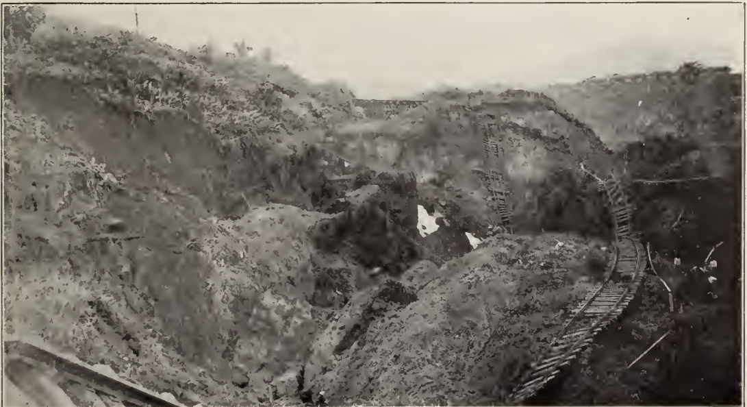
A break in the east bank of the Canal near Bas Obispo. This was caused by high water in the diversion channel, which broke through the separation wall, carrying into the Canal over 100,000 cubic yards of material, and flooding it for some distance. The disastrous effect on the railroad is clearly shown.
