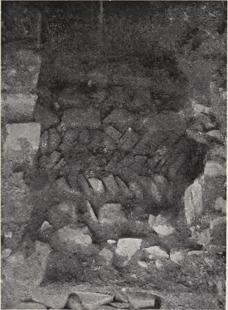
Glasfryn, Tremadoc : Arch in Room A, and Herring-bone Pattern of the Masonry
