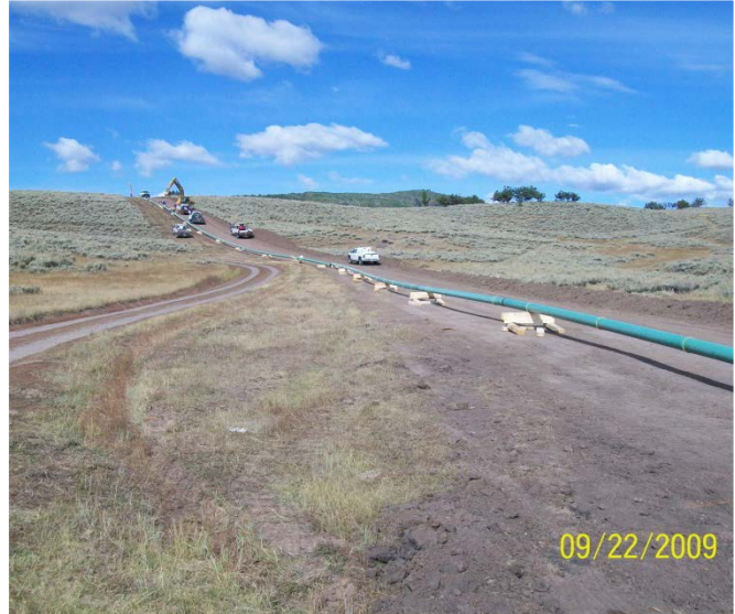
Photo 5: Typical corridor with steel gas-gathering pipe
