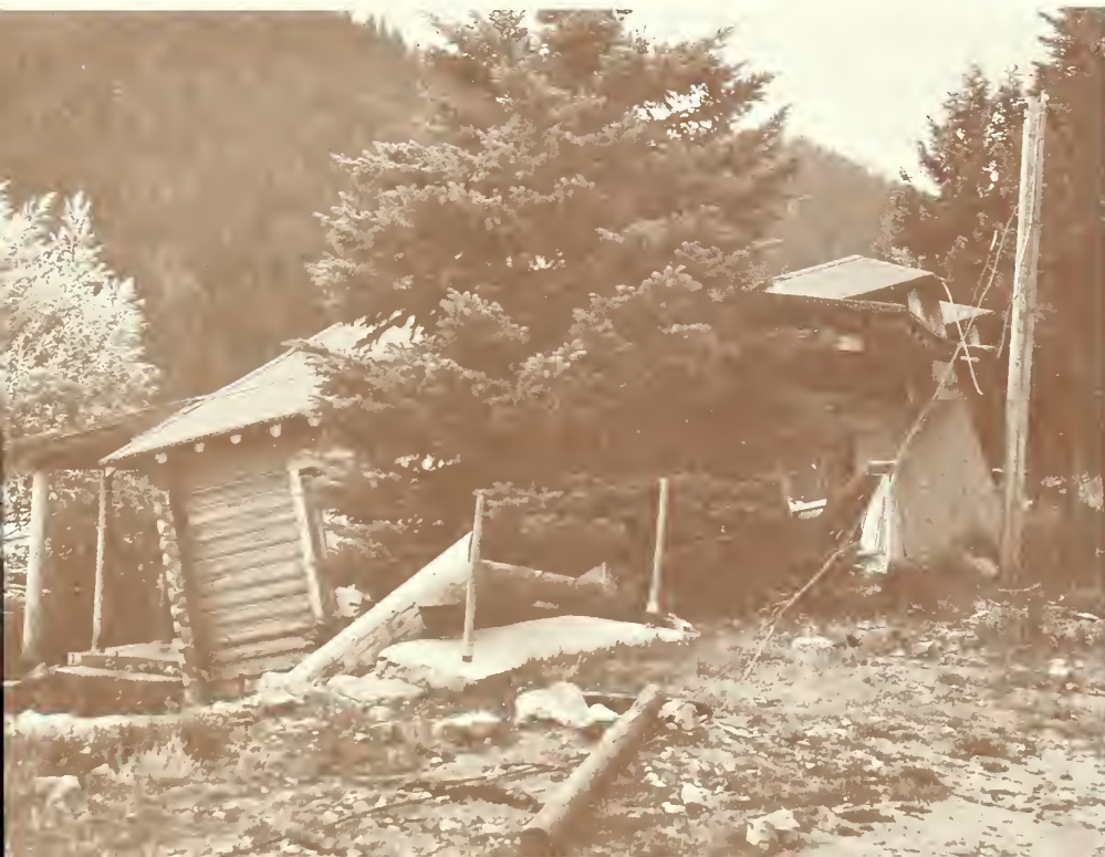
Bottom right: Interior of cabin at Hilgard Lodge showing the dark water lines of the seiche on the walls above the wood paneling. The water lines indicate degree of tilting of the cabin; this one was but slightly tilted.
