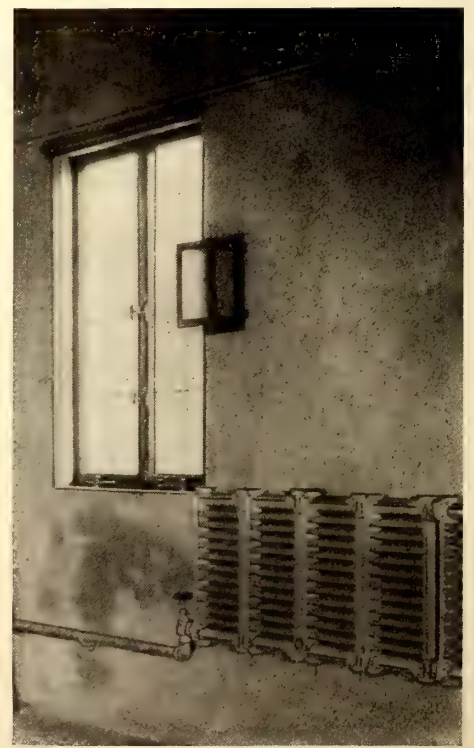
Steam Radiator and Inclosed Acetylene Light on the Wall
