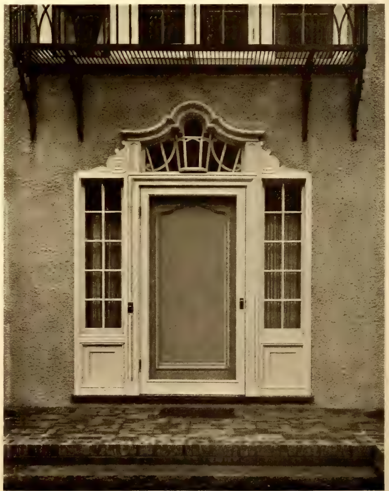
The Entrance Doorway, with Its Glazed and Curved Tympanum, Is the Most Striking Feature of the Exterior
