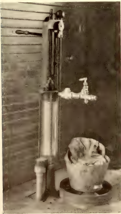
Gasoline Pump for Drawing Fuel from Tank in Ground Outside
