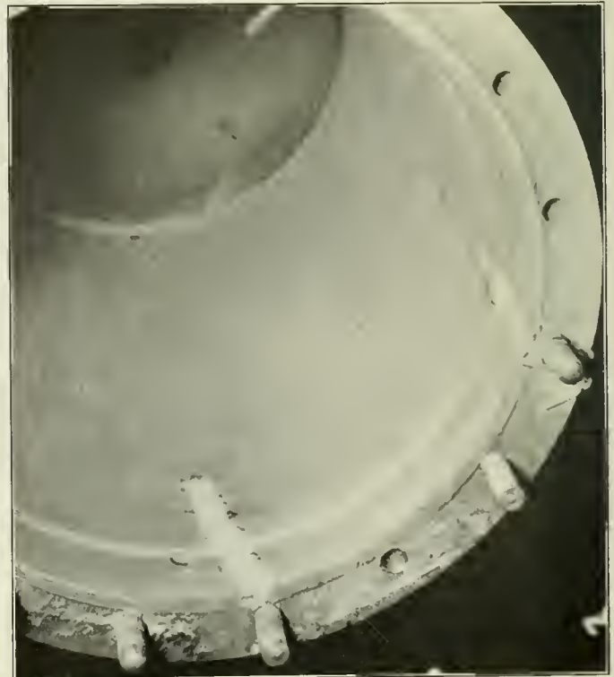
Fig. 19—Inside of Cracked Cylinder Which Had Been Repaired by Welding.
