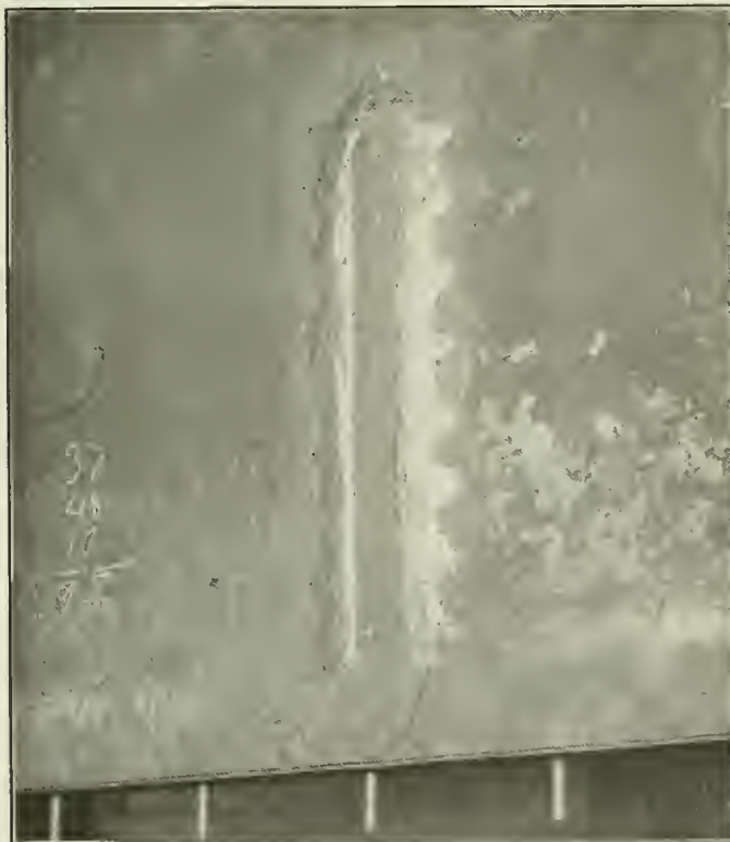
Fig. 10—Side Sheet Patch Welded to Firebox.
