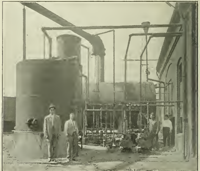
Boiler Washing and Refilling System.
