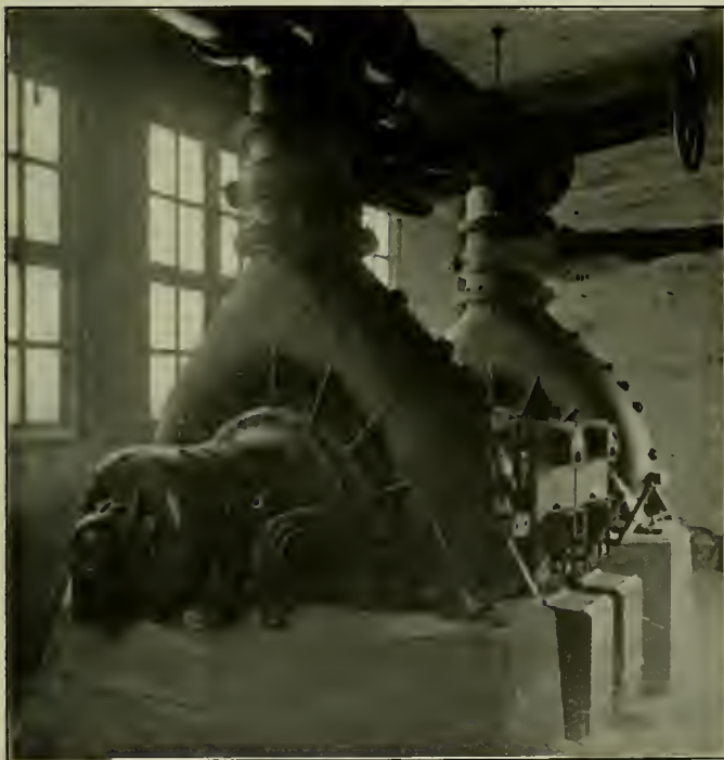
Blowers in Gas House.
