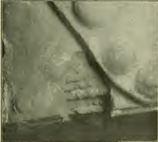
Fig. 1—Mud Ring Partially Welded After Being Drilled and Chipped Out.
