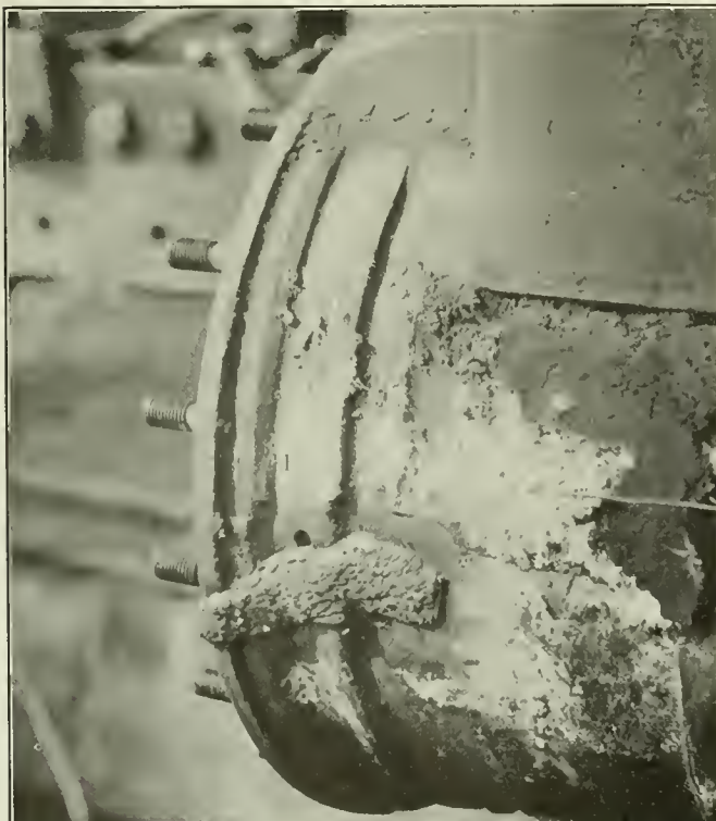
Fig. 18—Outside of Cracked Cylinder Which Had Been Repaired by Welding.
