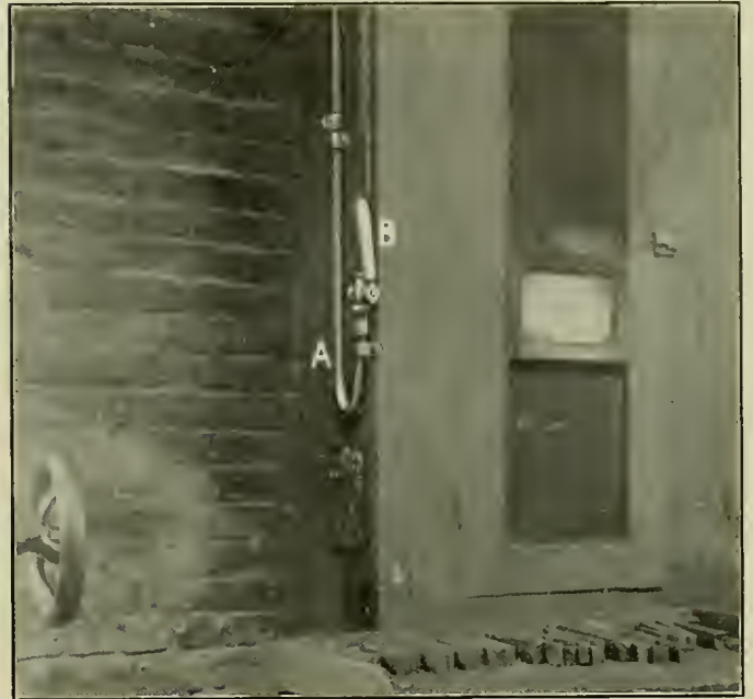
Fig. 6—One of the Air Valves in the Shop for Stopping the Engine in an Emergency.
