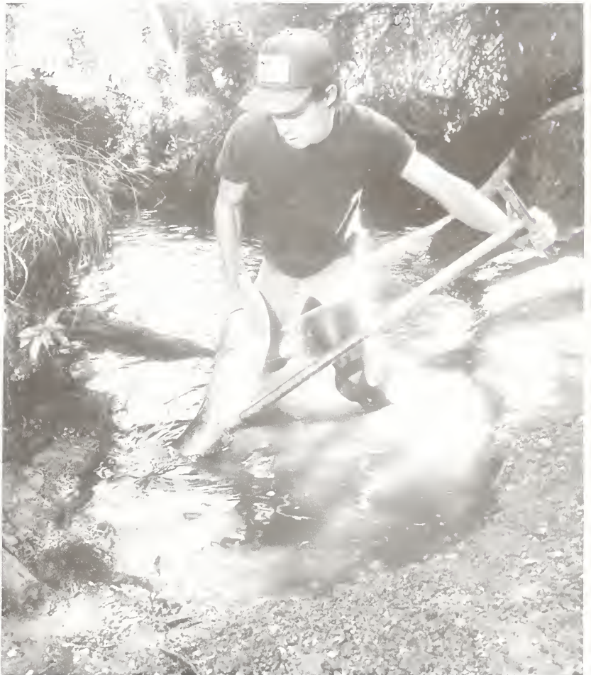
Randy Minnick, seasonal employee, removes sediment from Elk Creek with a suction machine. Photo by Shelly Hanks, Daily Idahonian, Moscow, Idaho.
