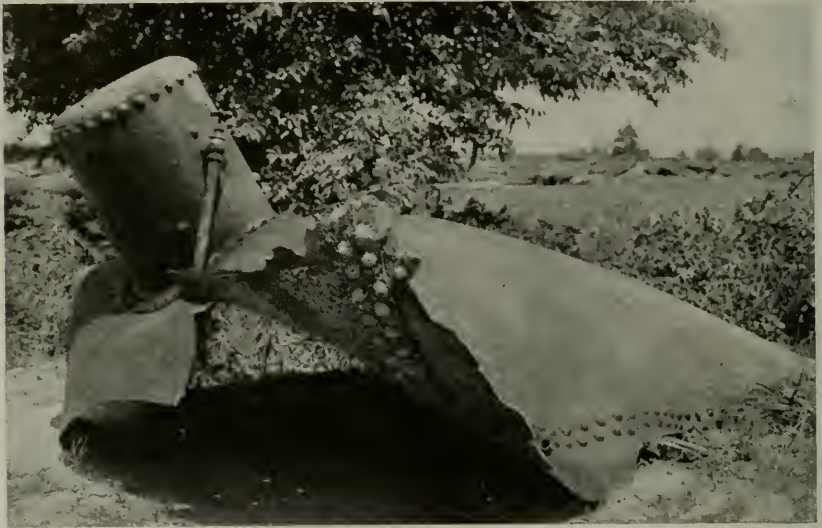
Figure 1—A crack in a longitudinal lap-seam caused the explosion of this boiler. Three men were killed and twelve others injured, eight of them seriously.
