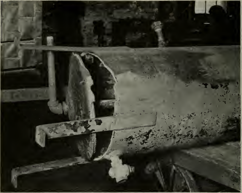
Figure 5—Broken shell of a hydro-pneumatic tank in which the shell had been crimped around the head and welded.
