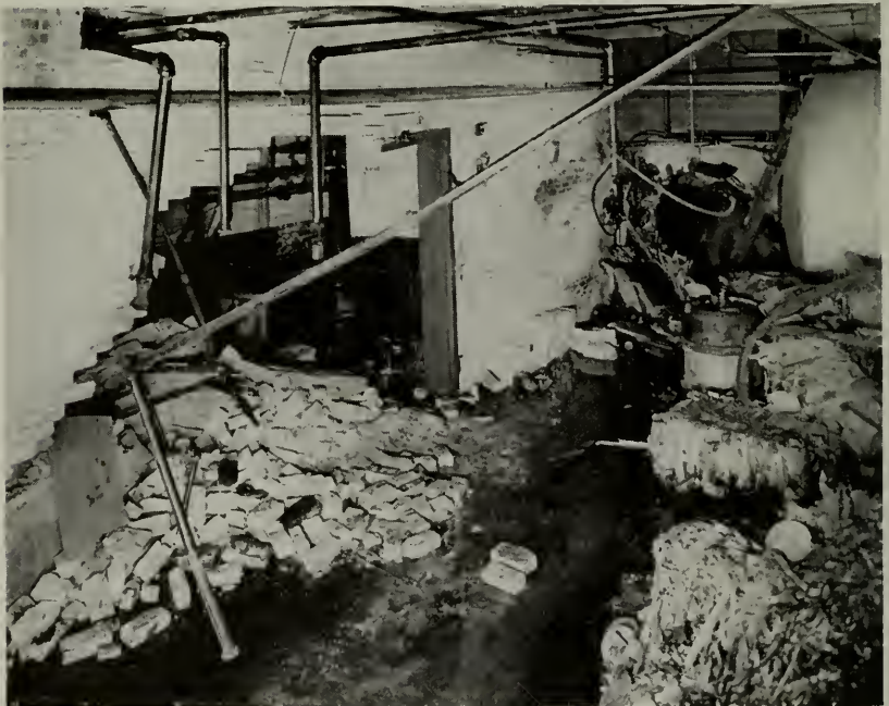
Part of the damage caused by the recent explosion of a condensate receiving tank.
