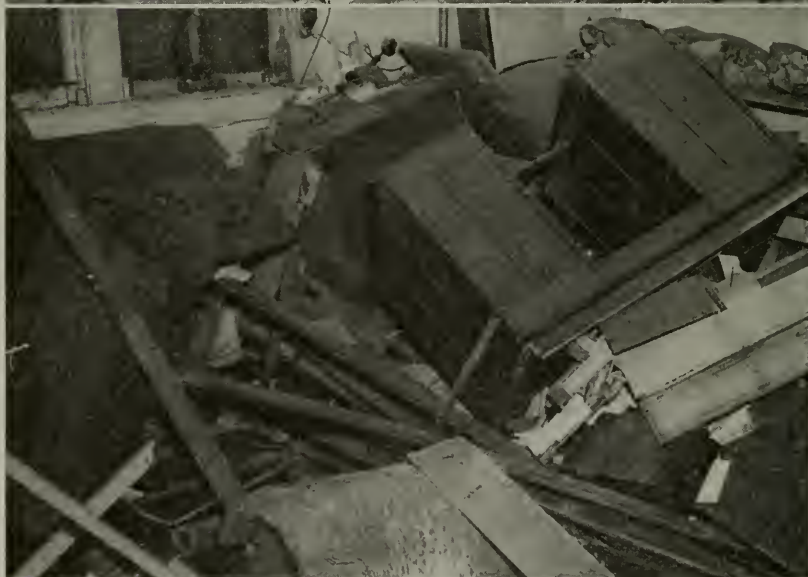
Figure 1 (Top)—An explosion of a cast iron sectional heating boiler caused this damage. A new boiler, it had been placed in service for the first time only a short while previously.
