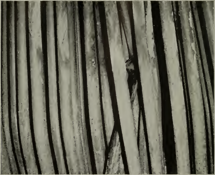
Figure 3—A bank of tubes in which magnetic oxide formed due to excessively high temperatures.
