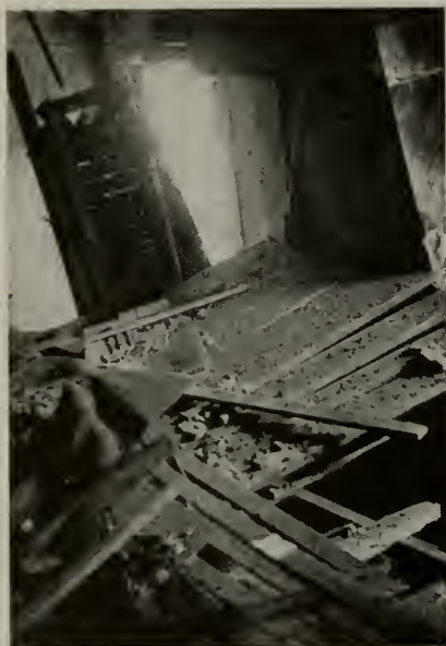
Figure 2—Part of the damage to the first floor of a residence from an explosion of a hot water tank.
