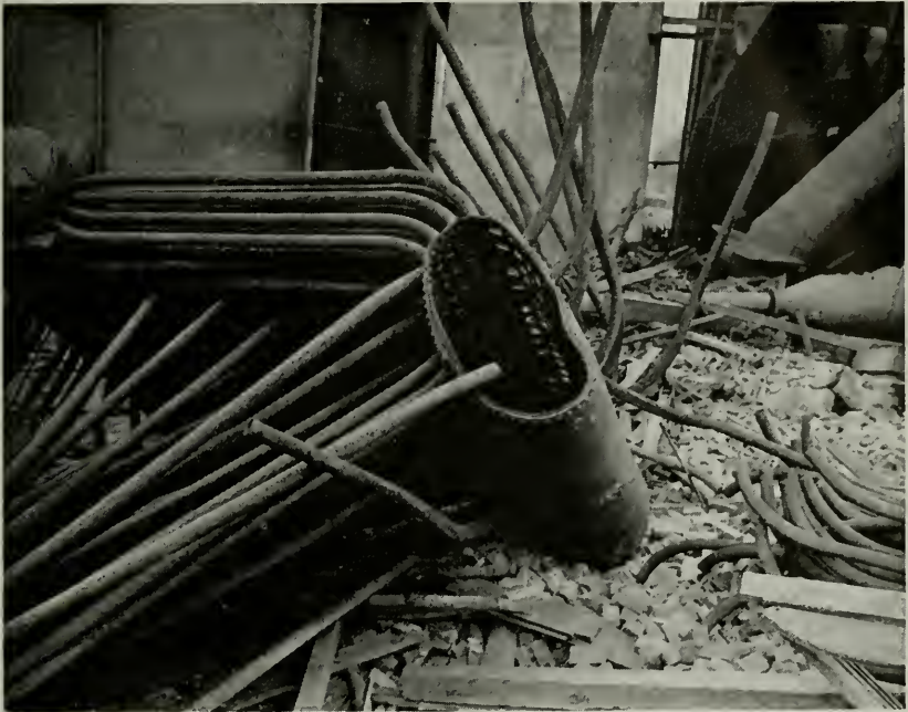
Figure 2—Weakened by corrosion, the blind head in the mud drum of this water tube boiler in a utility plant tore loose and caused the death of four people, injuries to six others and $100,000 property loss.
