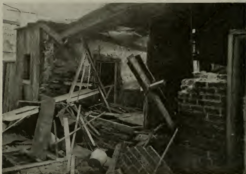
Figure 4—Part of the damage to a laundry building caused by an explosion of a small vertical flueless boiler.
