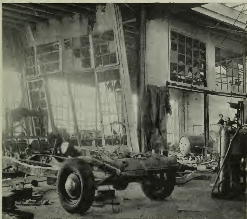
Figure 1—Typical damage as the result of an air tank explosion. This accident occurred in a paint spray room. A workman was injured.
