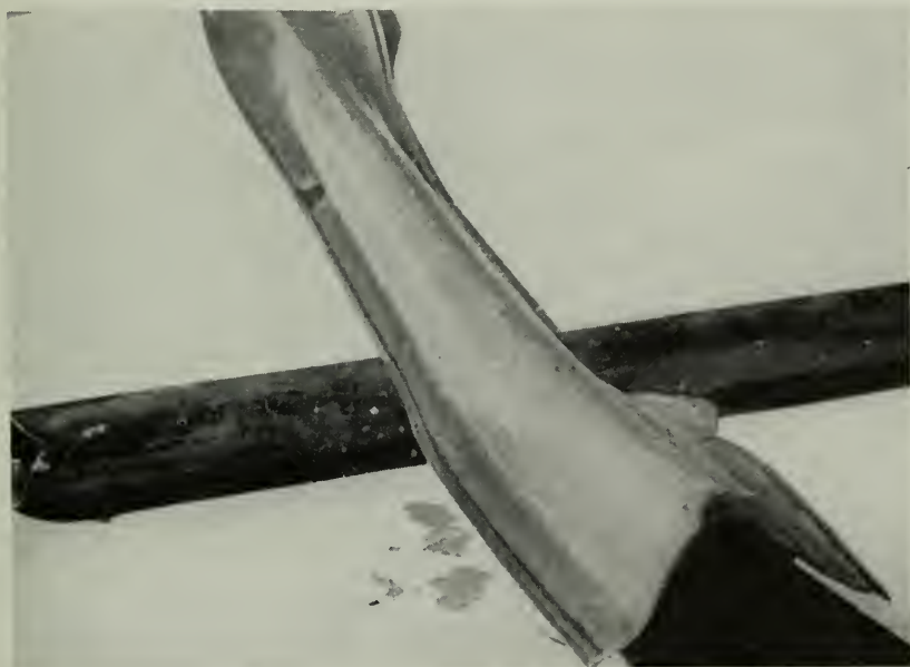
Figure 5—Stainless steel ammonia piping which tore open in a brewery.
