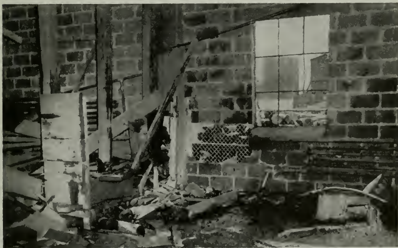
Figure 3—After an explosion of a cast iron hot water heating boiler in a garage. Originally located adjacent to the hole in the rear wall, the base of the boiler was hurled several feet to the right.
