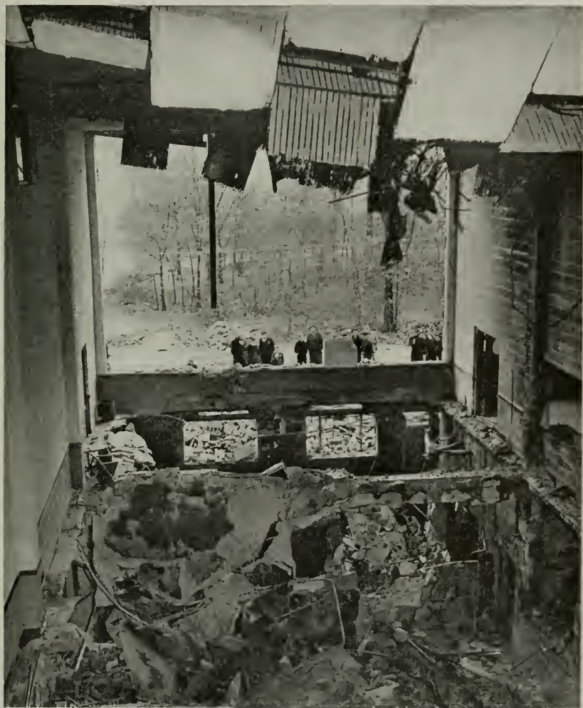
Pictured above are the ruins of a high-school study hall. An explosion of a hot water heating boiler caused this damage.
