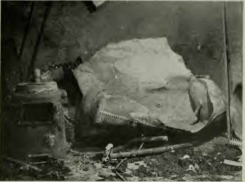
Figure 5—The damage resulting from the explosion of this hot water tank was estimated at $4,000. The cause was not determined.
