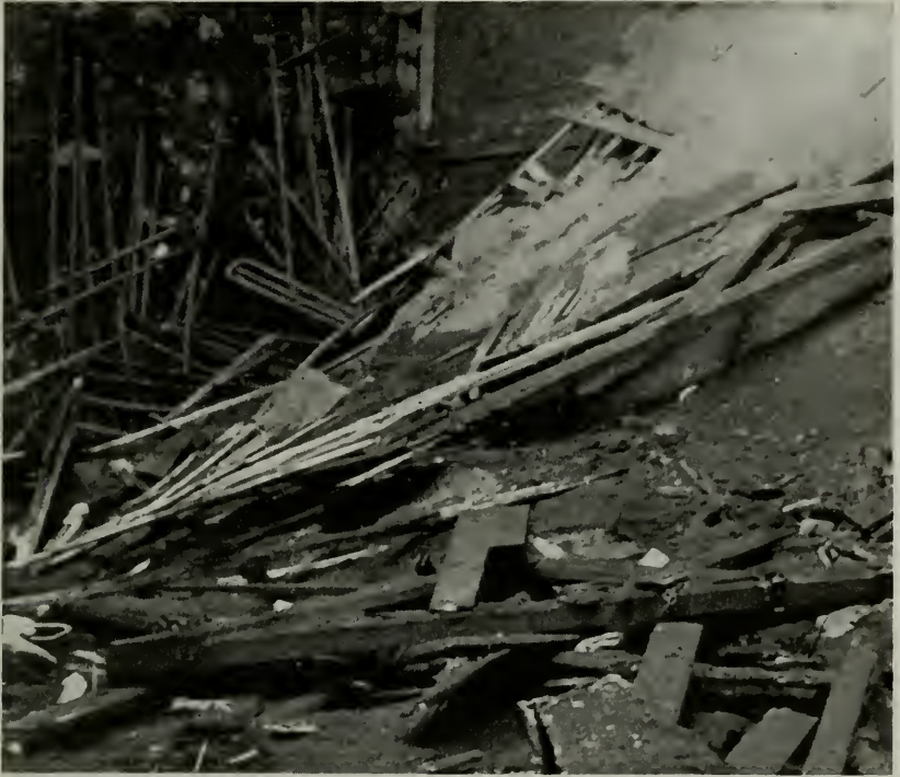
Figure 2—Some of the broken ammonia cooling coils and a section of the collapsed roof following an accident to a refrigerating system in an ice storage building.
