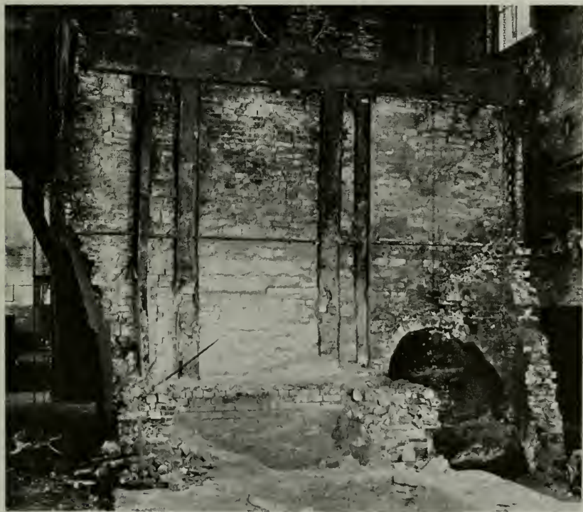
Figure 1—Boiler supporting columns, encased in intermediate brick-walls of a battery of boilers, almost entirely wasted away by oxidation from the high temperatures in the combustion chambers.
