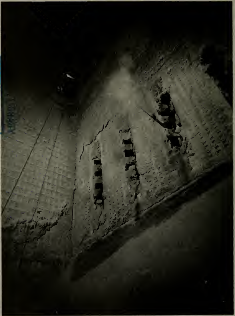
An inspector inside the combustion chamber of a 2000 hp Water Tube Boiler
