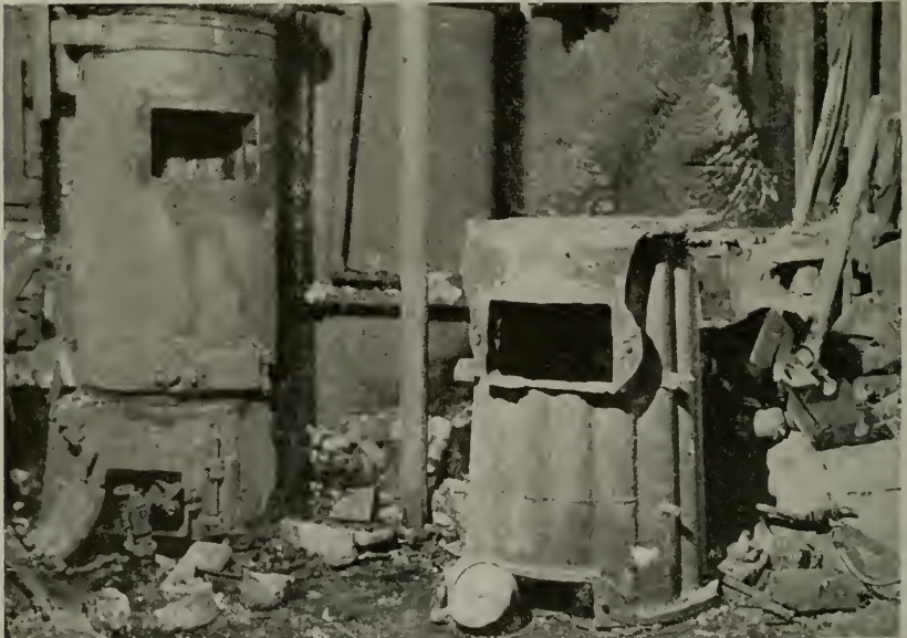
Figure 4—Through an operating mistake, a small hot water supply boiler was changed to a steam boiler. As its water relief valve did not afford suitable protection, the boiler exploded from overpressure.
