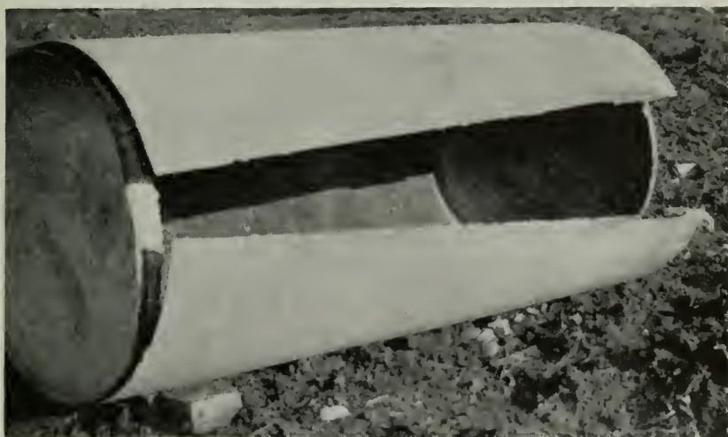
Figure 3—Failure of the longitudinal seam. Faulty welding was given as the cause of this accident.
