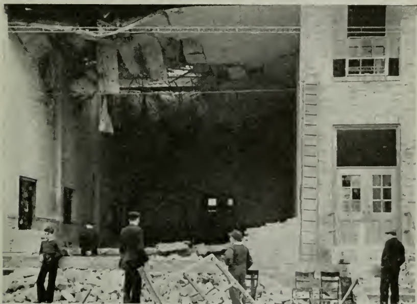
Figure 1—An explosion of a steel hot water heating boiler was responsible for the damage to this Ohio school. Excessive pressure was believed to have been the cause.
