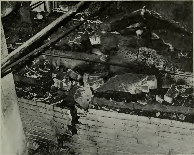
View of another watertube boiler—oil fired—showing damage from a furnace explosion.
