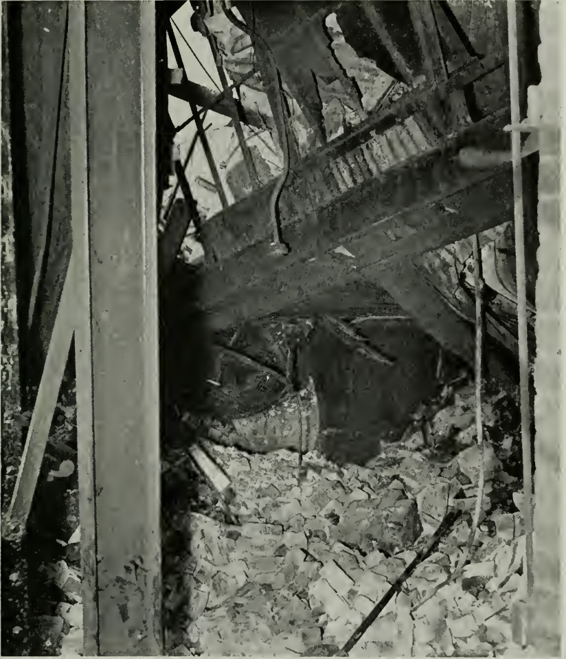
Figure 1—Top page 226—Damage after the explosions of a creosote tank and a water tube boiler at a southern plant.
