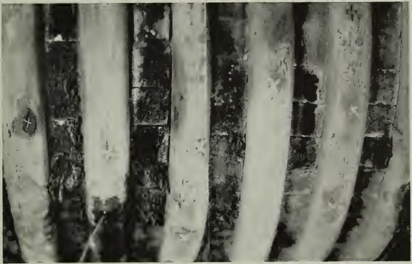
Figure 1—Deposits of scale at the bends in these tubes permitted general over-heating of an entire row. Finally one of the tubes burst (second from the left in the picture), but the warning came too late.
