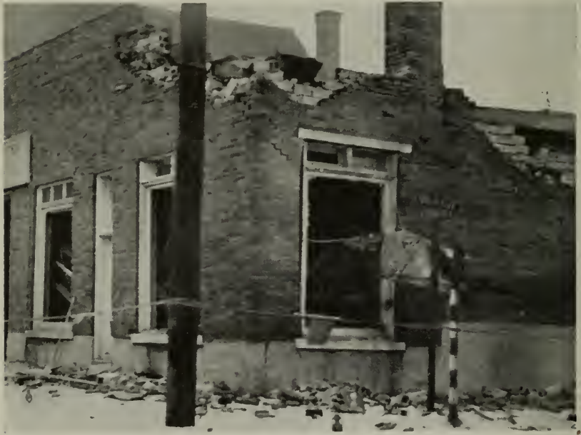
Figure 1—Damage to the exterior of a large garage because of a hot water tank explosion.
