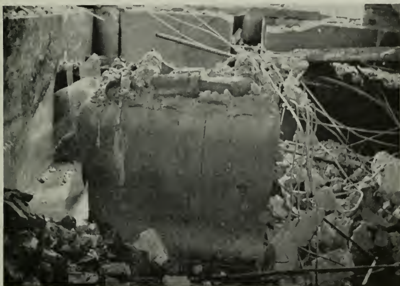
Figure 2—Basement of an automobile showroom after the explosion of hot water equipment. Three automobiles fell through into the basement when the floor was destroyed by the blast.
