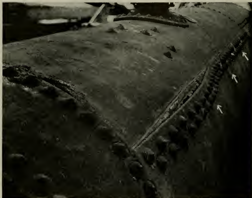
Figure 3—Failure in the longitudinal seam of No. 1 boiler during the hydrostatic test. A few of the paths of embrittlement defects are exposed and clearly show the progress from rivet hole to rivet hole. This boiler has been slotted as a means of detecting a lap seam crack. The slots are indicated by the arrows. See also Figure 4.
