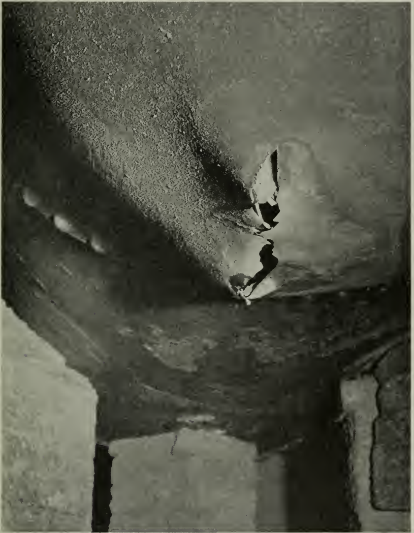
Figure 1. A serious rupture caused by over-heating.
