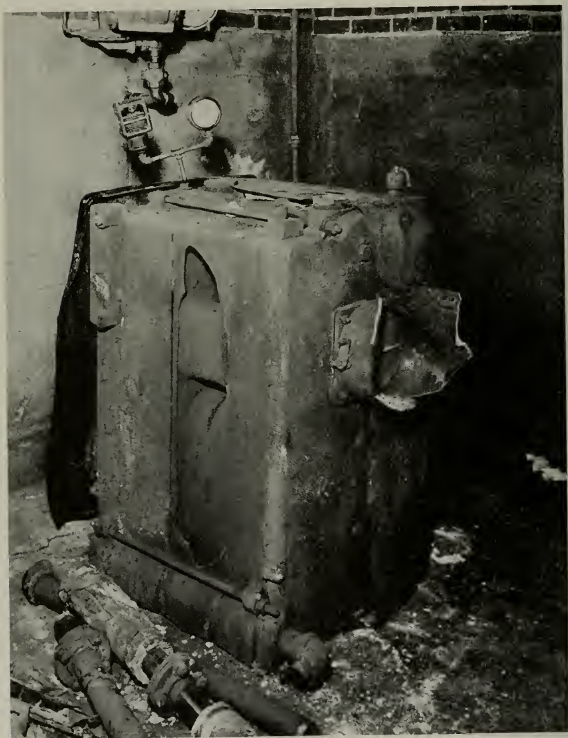
Figure 4—Failure of a pressure control device plus an inoperative safety valve caused the explosion of this cast iron steam heating boiler in a Kansas residence.
