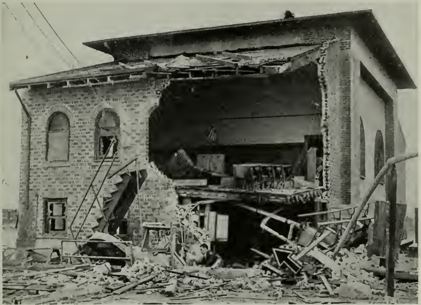
The damage to this school was caused by an explosion of a hot water tank.
