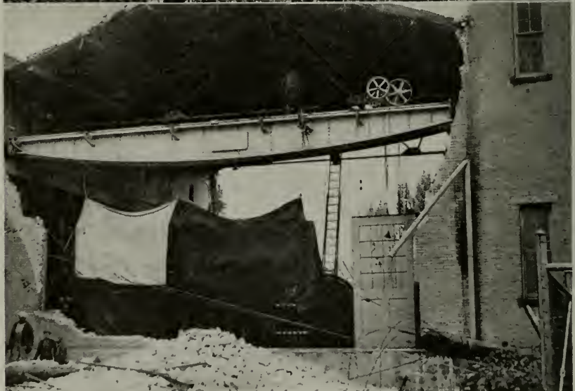
Two views of a utility sub-station after an explosion, caused by a direct stroke of lightning, blew out the end-walls.
