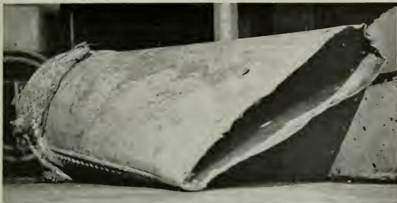
Figure 1—Over-pressure caused explosion of this hot water tank in a laundry. The property loss was over $5,800.
