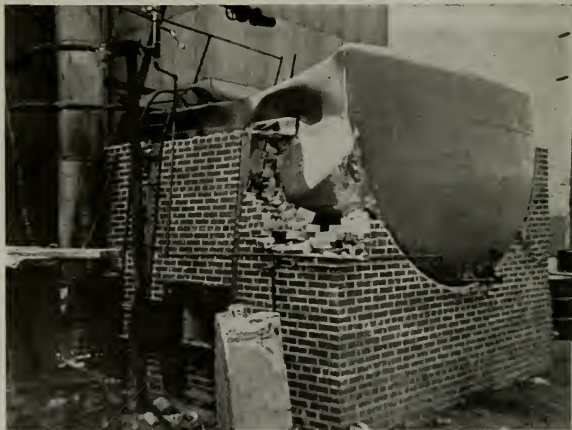
View of a large tank after it had collapsed while being given a vacuum test.
