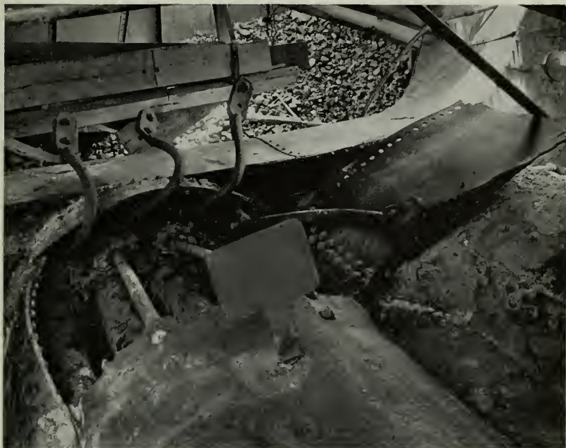
Figure 1—The failure in Boiler No. 2. The break along the rivet holes near the caulking edge of the seam at the left is clearly evident.
