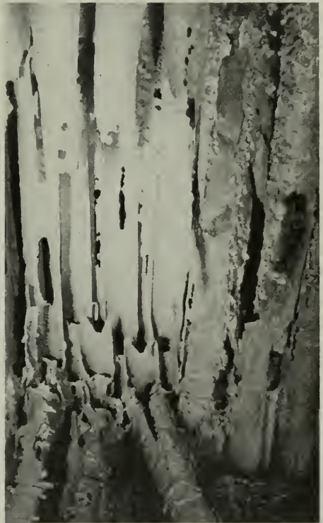
Figure 5—Rear wall of the furnace after forgotten open blow-off valves had drained the tubes.
