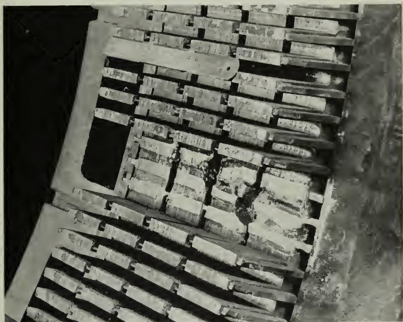
Figure 1—Failure of 450 hp hoist motor showing the iron burns after three laminated teeth had been cut away.
