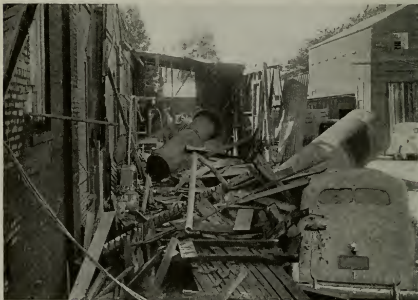
Damage at a creamery and cold storage plant caused by a boiler explosion as a result of low water which, in turn, was attributed to failure of automatic controls. The furnace in the boiler overheated, collapsed and ruptured. Property loss was nearly $5,900.
