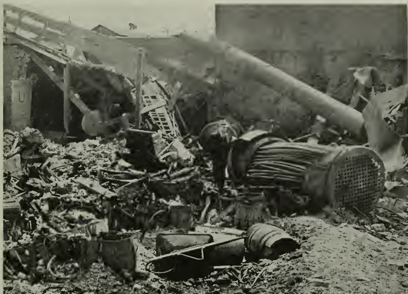
Figure 4—A building demolished by an explosion of a vertical tubular boiler which had been poorly patched by welding.
