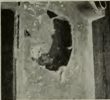
Figure 4—Failing section of a hot water heating boiler in a theater.
