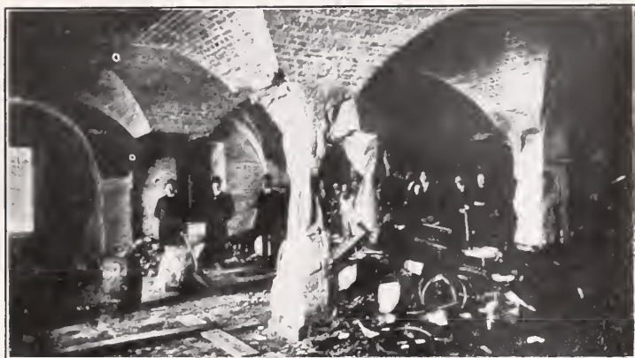
Fig. 1 Showing damage to granite pillars in United States Public Store House No. 1 at Baltimore Md. 1904
