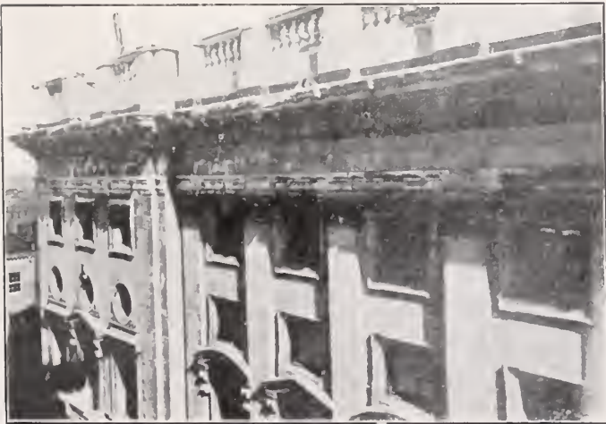
Fig. 2 City Courthouse at Baltimore Md., showing the damage to the marble facing. 1904
