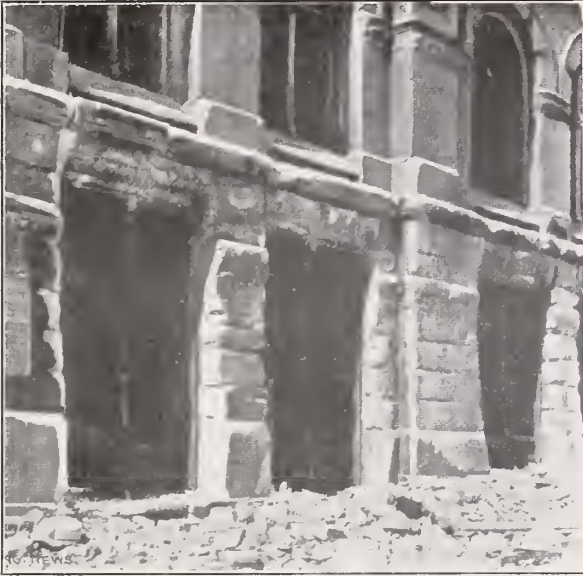
Fig. 1 Bluestone front of the Baltimore & Ohio Railroad Co.'s building at Baltimore Md., damaged by fire. 1904
