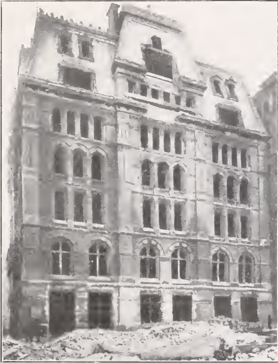
Baltimore & Ohio Railroad Co.'s building at Baltimore Md., showing the effect of the fire on the stonework and the slate roof. 1904
