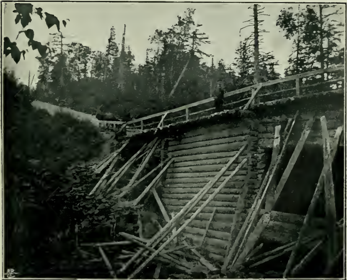
AN ATTACK ON THE POST. REPAIRING THE BRIDGE CUT BY THE "PRODYAGI."
