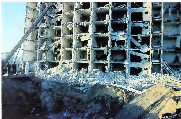
Fig. 24-1. Remains of Khobar Towers in Dhahran, Saudi Arabia. On 25 June 1996, terrorists bombed this complex, which was used as a barracks for US Air Force personnel. Note the large crater in front of the building and the loss of the building closest to where the truck bomb was parked. This bombing caused 19 deaths and 500 injuries.
