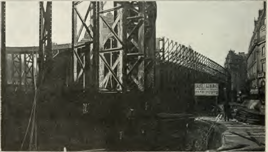
The St. Michel Station, Under Construction, Showing One of the End Caissons; Paris Metropolitan Railway.
