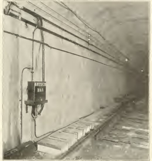
Fig. 5—Fire-Proof Fixtures at Switches.
