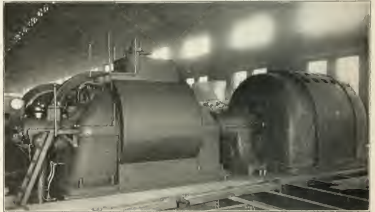
Double-Flow Turbine Direct Connected to Generator.
