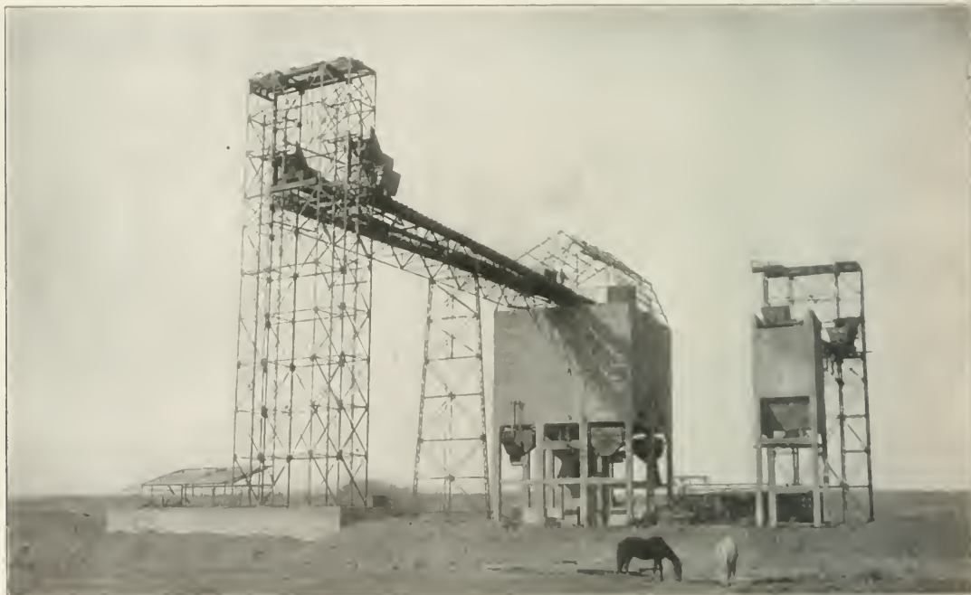
Coaling and Cinder Plant at Belen, N. Mex., Under Construction; Atchison, Topeka & Santa Fe.
