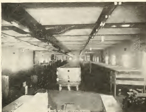
Fig. 3—Battery Floor, Looking West; Yonkers Power House.
