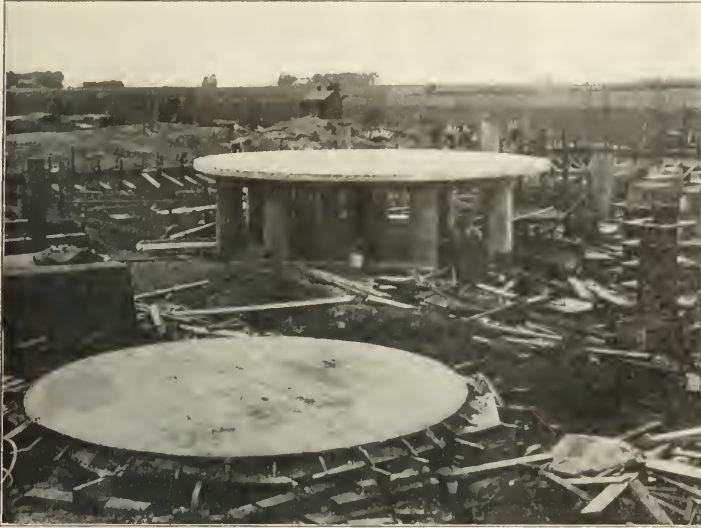
Reinforced Concrete Foundation for Tank; Galesburg Timber Preserving Plant. Table for second foundation in form in foreground.
