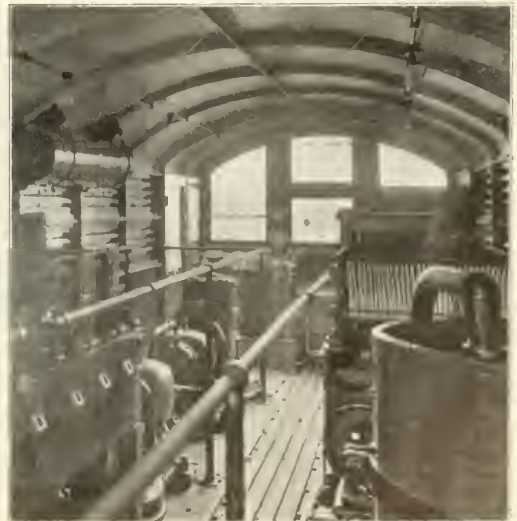
Interior Arrangement of Electrical Apparatus.
