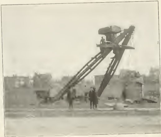
Anchor for Cable Conveyor.
