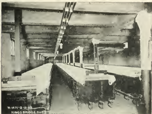
Fig. 1—Battery Floor; Kings Bridge Sub-Station.
