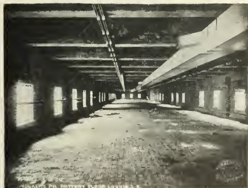
Fig. 2—Battery Floor, Looking East; Yonkers Power House.
