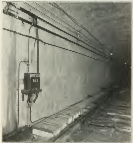
Fig. 5—Fire-Proof Fixtures at Switches.
