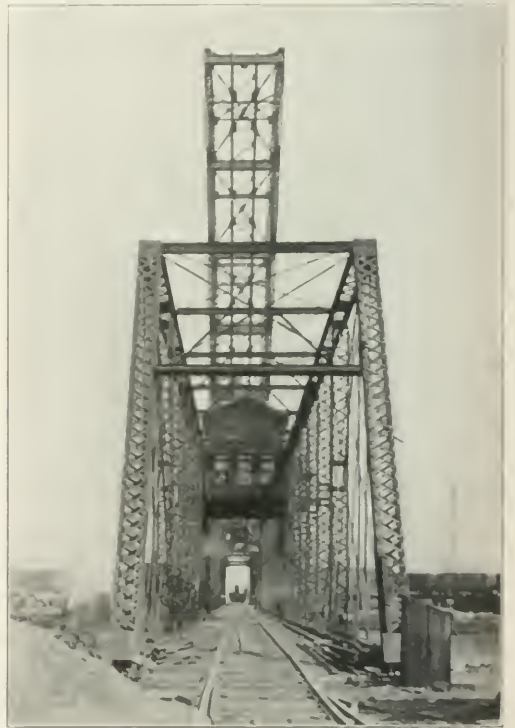
End View, 230-ft. Scherzer Bridge, Showing Method of Construction Without Interference with Traffic.
