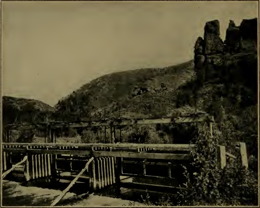
FIG. 94. Headgate of a canal.
