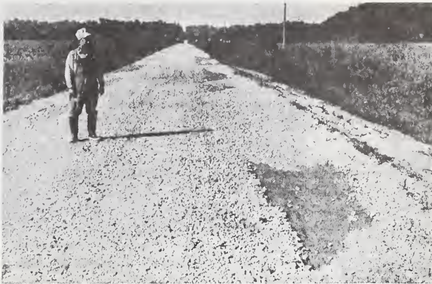
ROAD DAMAGE ALMOST $1 PER ACRE —Clyde Hamilton inspects damages inflicted to the county road adjacent to his farm, 4 miles south of New Lancaster. That damage is high is shown in the report of R. H. Eckhoff, Miami county engineer, who estimated that flood damage to the 1091 miles of county roads amounts to $310,000. Miami county, with an area of 378,240 acres of which 361,026 acres are agricultural land, is serviced by 88 miles of surfaced state and federal roads, 29 miles surfaced, 922 miles gravelled and 140 miles graded dirt county roads. Flood control on the streams would greatly reduce road damages caused by these deluging storms. (Courtesy Soil Conservation Service)
