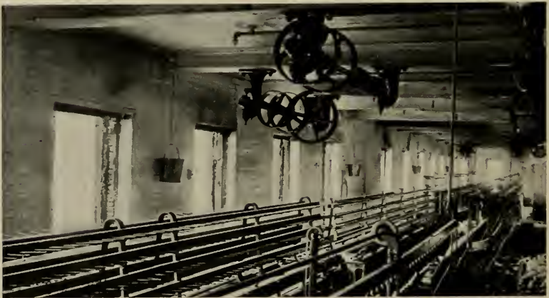
INTERIOR OF FOURTH FLOOR OF PICKER HOUSE, SHOWING WINDOW CASINGS DESTROYED WHILE THE FRAMES JUST INSIDE AND PILE OF BOBBINS AT THE RIGHT WERE UNHARMED
