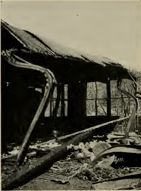
DETAIL OF STEEL WORK, SHOWING RESULT OF FIRE. WASHBURN & MOEN MFG. CO.
