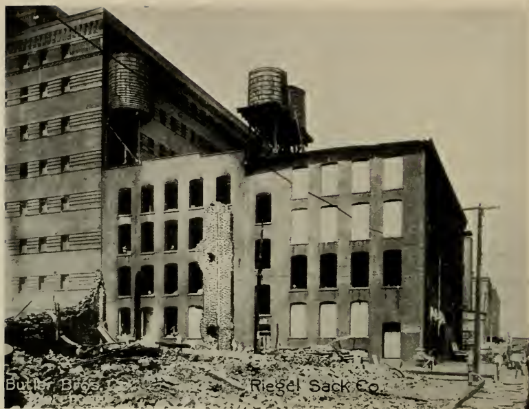
RIEGEL SACK COMPANY BUILDING, SHOWING BURNED-OUT WINDOWS, ALSO THE TANKS CHARRED BY THE FIRE
