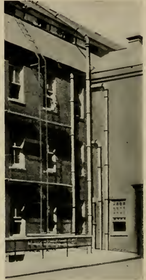
PERFORATED PIPE SPRINKLER FEEDERS
