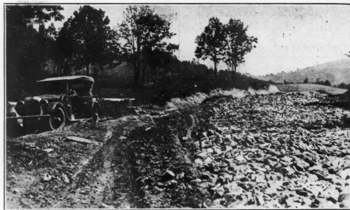
Building a road of iron ore. Native rock is often used as a subsurface in highway construction and much of the rock in the Western part of the state is not far removed from the pig-iron stage
