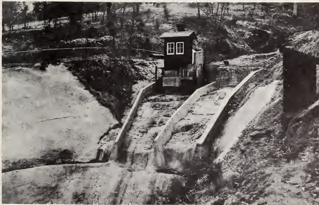
Stream gaging station at head reservoir provides continuous record of runoff. Consists of 90° V-notch weir under instrument house for low flows and 24-inch San Dimas flume at right for moderate and peak flows. Right channel built to divert mud and boulder flows.
