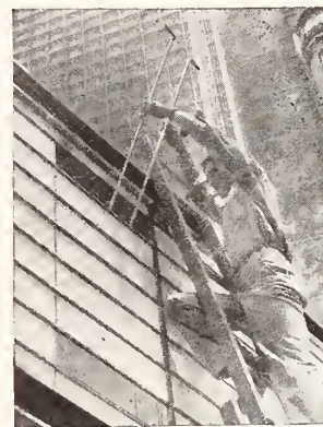
Showing Marquee illuminated with Fluorescent Tubing. Note how easily the tubing is handled in or out, through the "Remova-Panels."
