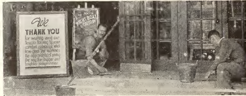
Temporary inconvenience to patrons of the Reo Cinema, Fazakerley, Liverpool, England, when new flooring was installed in the lobby, was overcome by this clever announcement posted by manager W. Roberts, thanking patrons for wearing away the terrazzo through constant patronage.
