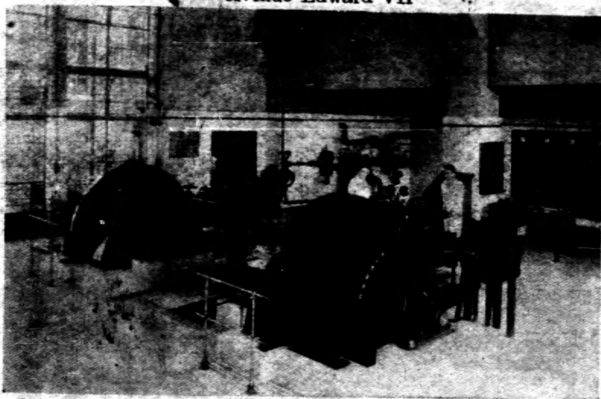
Sulzer Refrigerating Plant (2X270000 cal./h. at -13°+40°C) Installed at the Union Brewery in Shanghai
