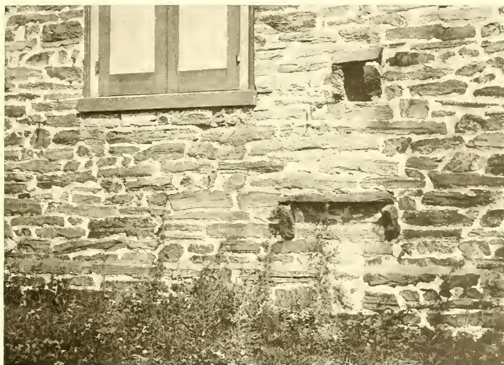
SMOKE HOLE IN WALL OF HAVERFORD MEETING HOUSE, 1700 The oldest church building in Delaware County
