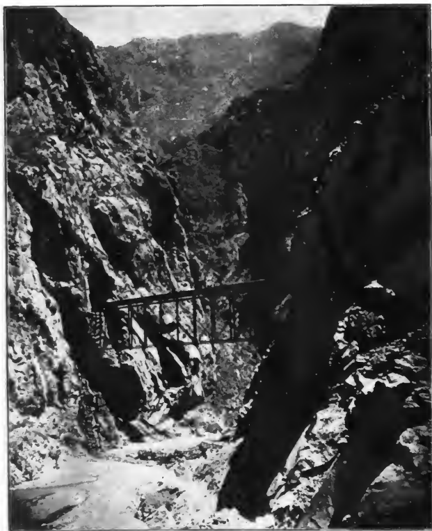
THE FAMOUS "INFERNILLO" BRIDGE ON THE OROYA RAILROAD, PERU, 2 MILES ABOVE THE SEA.
