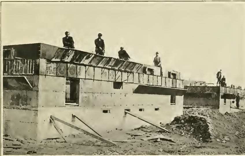
NOTE THE STEEL FORMS AND SWING-UP. (Forty Buildings, D. L. & W. R. R.)
