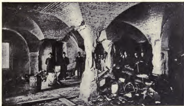
Fig. 2. — Effect of fire on granite columns, U. S. Public Storehouse, Baltimore, Md.
