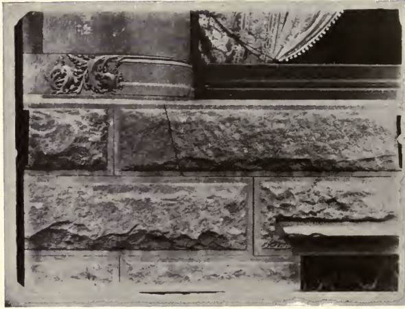
Fig. 1. — Sandstone broken by transverse strain-caused by settling of the building.
