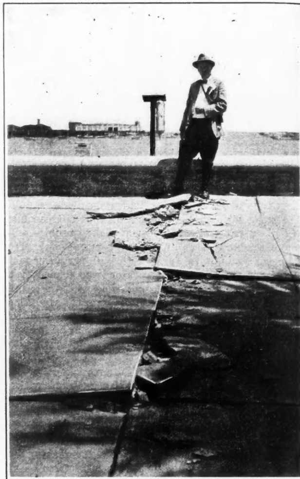
How the earthquake spoiled a cement sidewalk
