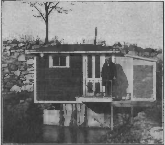
FIGURE 5.—Compact turbine plant in Massachusetts, built over the tailrace of an old rubble-face earth dam 18 feet wide on top (at tree). Drainage area 8 square miles, head 10 feet. Plant supplied current for lighting five rural houses
