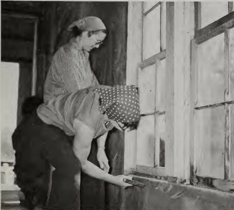
Before nailing on the paneling, workshop participants line the walls with polyethylene.
