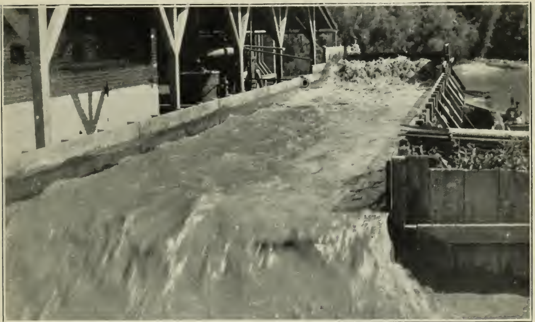
FIG. 2.—PUMPING PLANT FOR RICE IRRIGATION.
