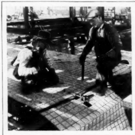
Applying the Wire Carpet as Reinforcing for Concrete Floor; It Also Serves as Insulating Material
