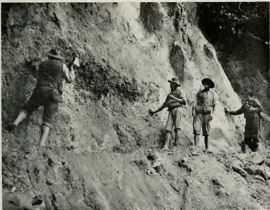
Cutting out a new trail five hundred feet up the face of a cliff where a slide had obliterated the path. This point in the trail is known as "Sal-si-puede" ("Get out if you can")
