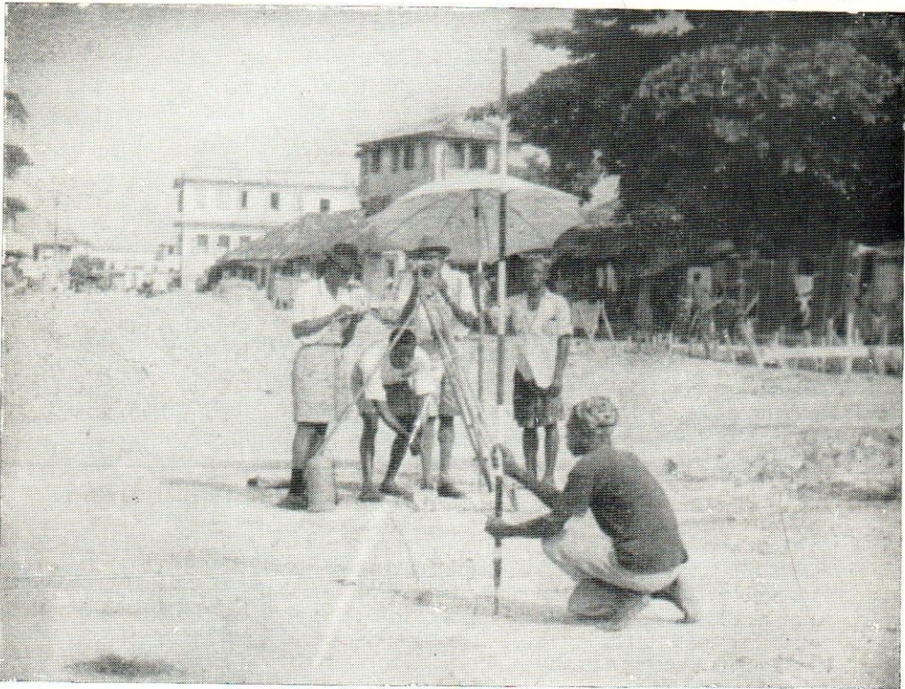
Setting out for re-development of cleared areas under the direction of the Board's Chief Surveyor, Mr. L. A. Akande Smith.
