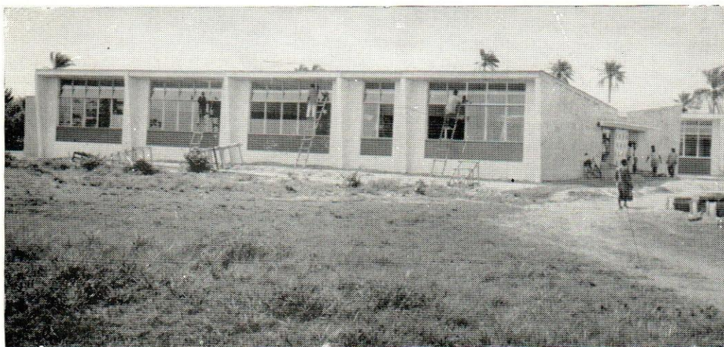
One of a number of schools to serve the Suru-Lere Estates, nears completion.
