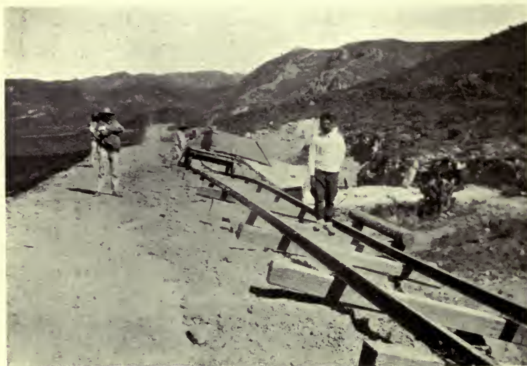
Building a Railway in Hidalgo. The man between the rails is a murderer and a good workman.
