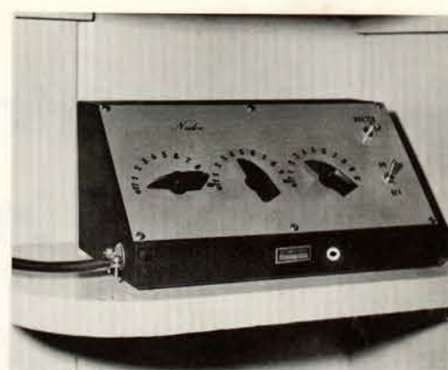
Pharmacy technicians update visual display through selector switches on remote control panel.
