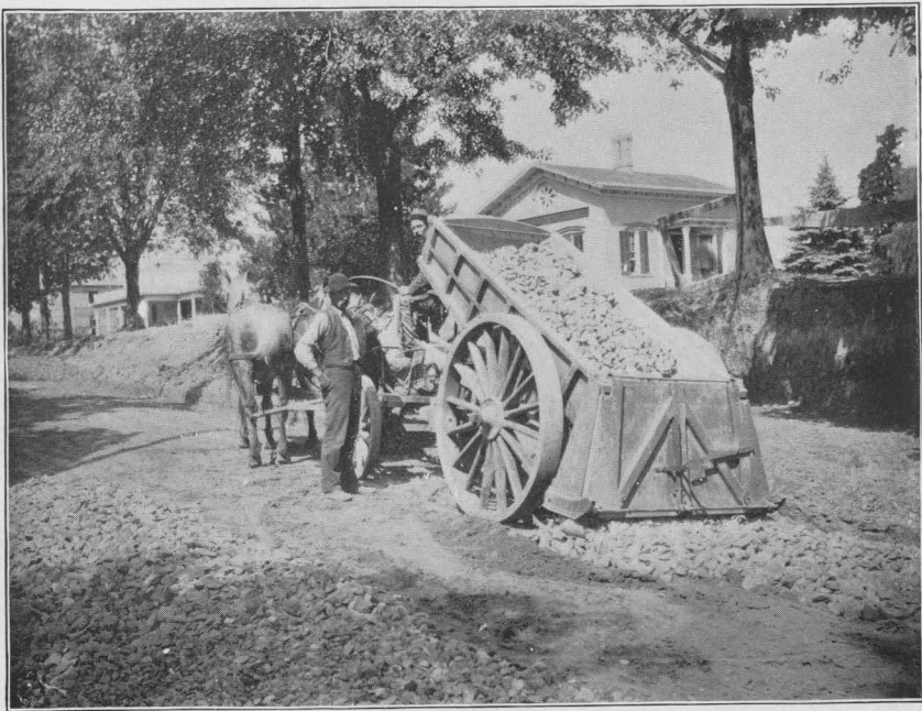
FIG. 2.—UNITED STATES OBJECT-LESSON ROAD AT GENEVA, N. Y. (PLACING THE MACADAM FOUNDATION.)
