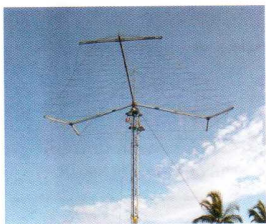
HF Antenna AK451 as backup system
