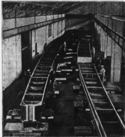
View Showing Manner of Assembling the Arch Ribs at the Works of Chatillon & Commentry; Alexander III. Bridge, Paris, France.
