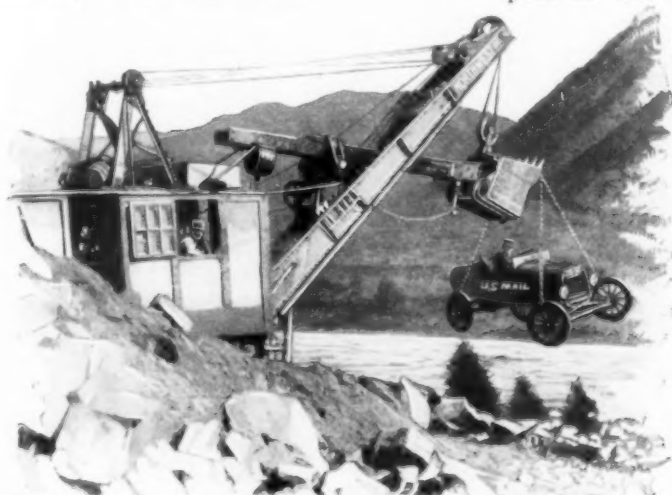
Where the Mail Goes Around with the Steam Shovel; Swinging Carrier's Car Past Repair Obstruction
