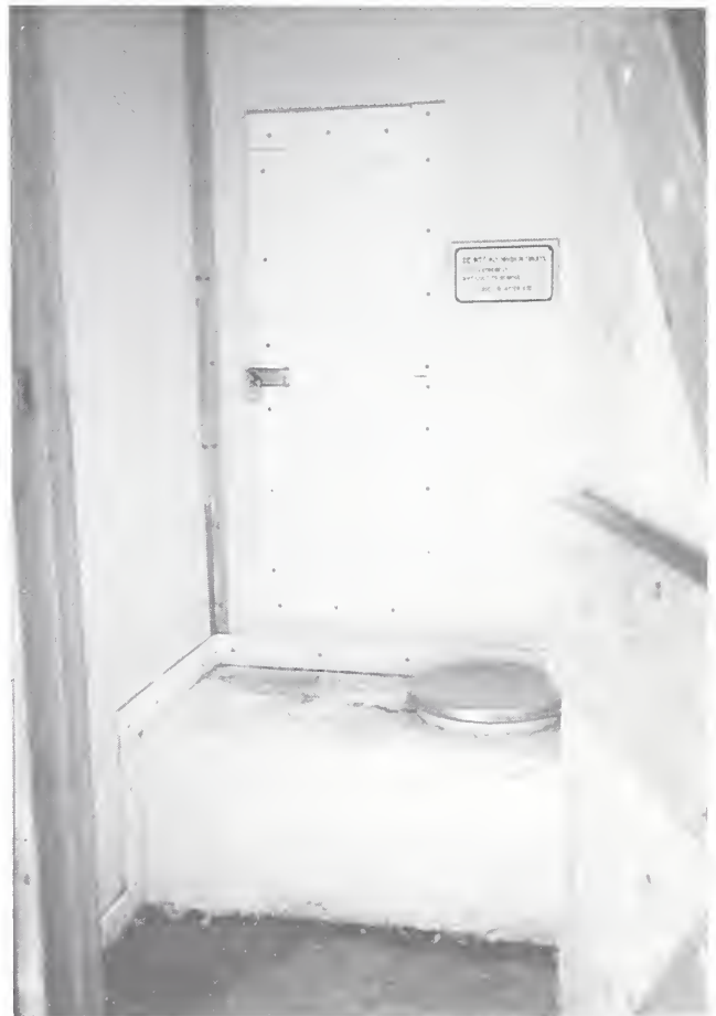
Figure 1. Bench seat. Footprints and scuff marks from people standing on the bench seat in toilet at Nevada Falls, Yosemite National Park (NP).
