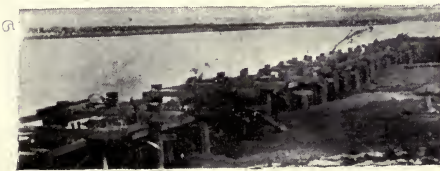
FIG. 129.—Revetment in the Missouri River to prevent undercutting. The river is flowing from left to right.
