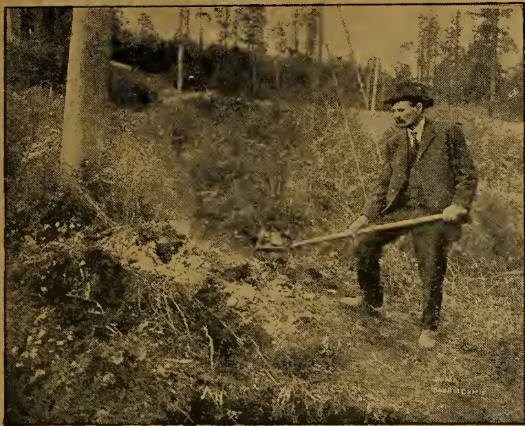
The smouldering fire is here being covered with clay to force it to burn to the roots' ends, for when the stumps are burned off at the top of the ground the job is but partly finished
