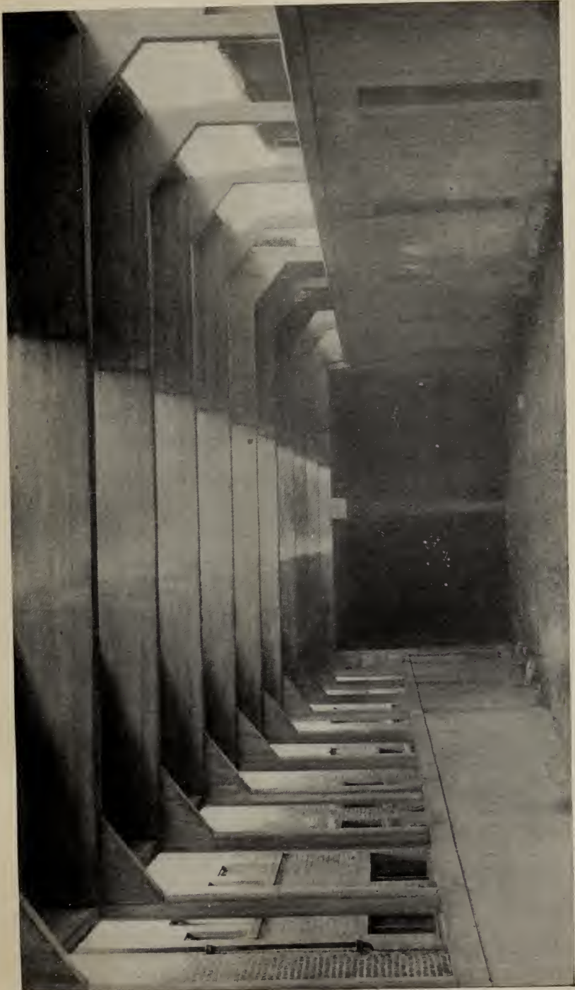
Incline of Section 1 of the Washington Street Tunnel, near Ash Street, looking northerly. Walls and covering are of reinforced concrete.
