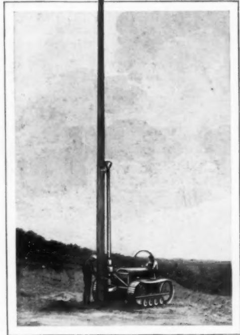
Setting a Pole After the Hole Is Dug; the Endless-Tread Tractor Is Fitted for Rough Travel
