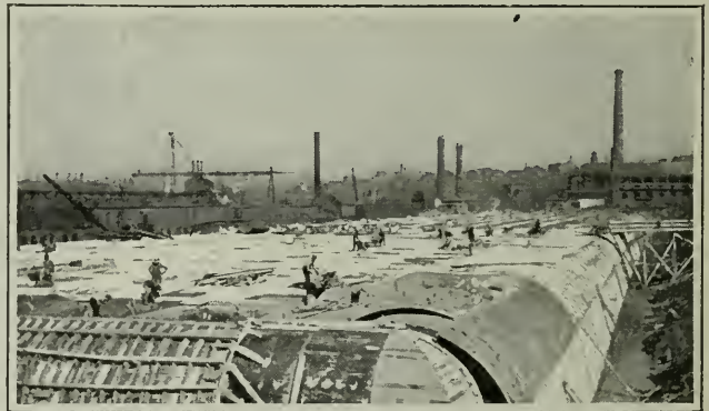
The top of this one hundred and fifty million gallon tank will be a fifteen-acre park
