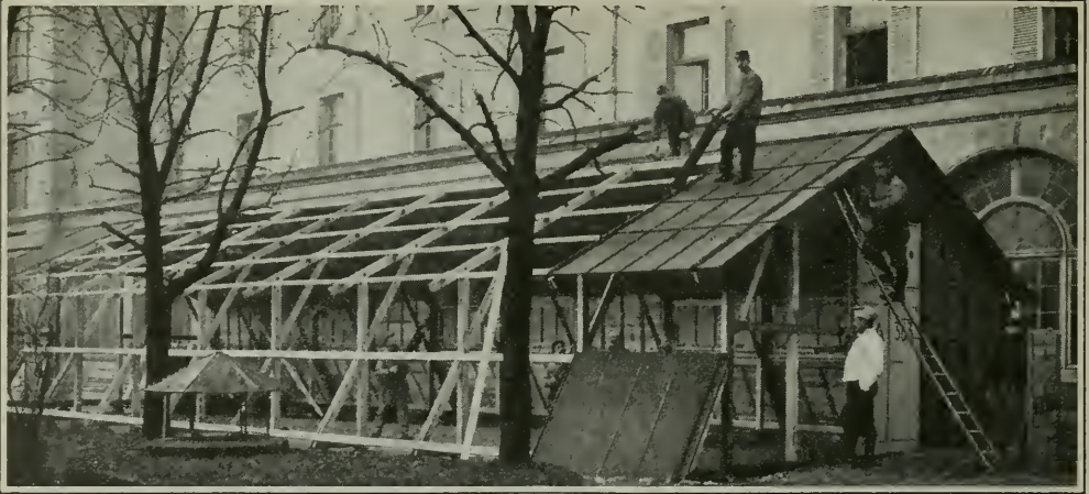
Constructing portable barracks for French troops. These houses may be quickly set up immediately behind the firing line, and form an admirable shelter for soldiers who are taking their three days' rest from the trenches
