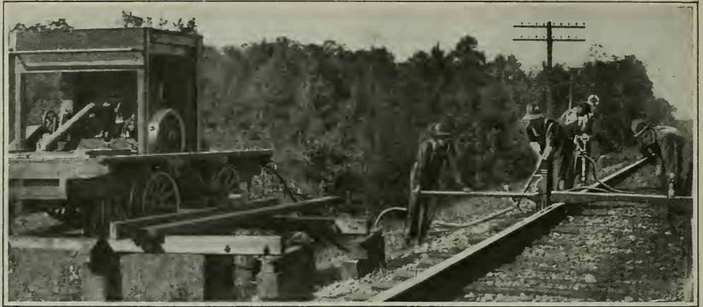
A track surfacing and tamping gang on the New York Central. The compressor car is mounted beside the track to furnish compressed air to the tampers
