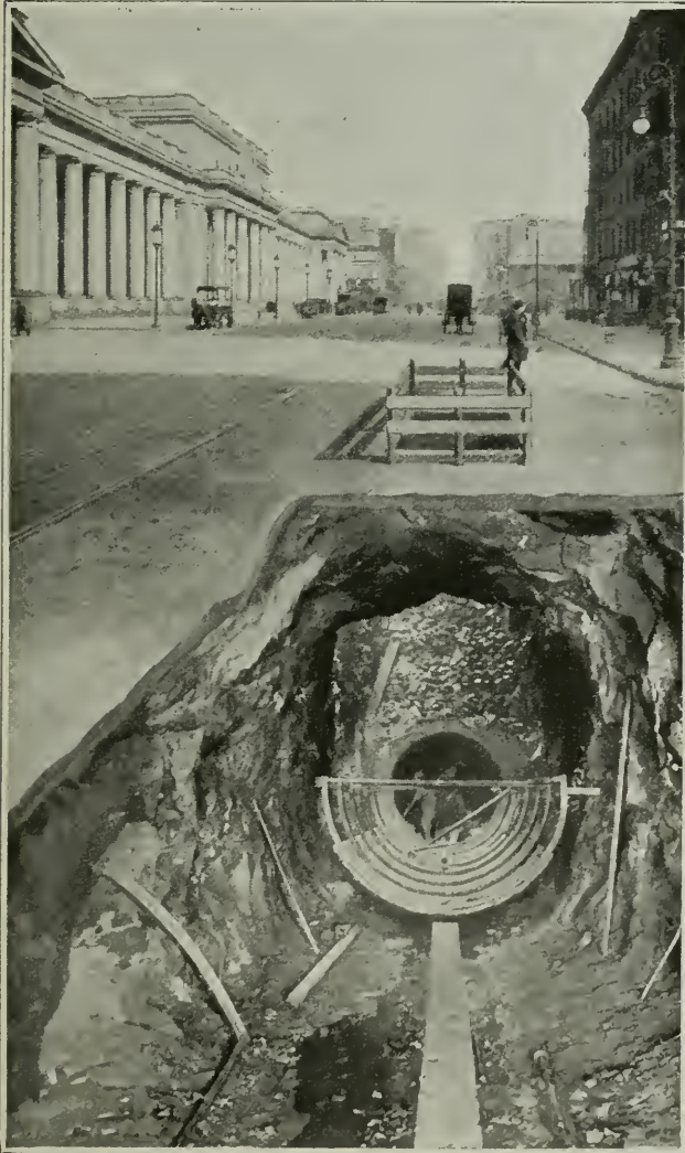
Rebuilding and moving sewers to vacate space required for the new subways. The sewers alone mean an expenditure of from six to seven million dollars. The illustration shows a large tube making a new outlet for the sewer system emptying into the Hudson River. This outlet will cost the city half a million dollars. To the left of the picture is the magnificent new Pennsylvania Terminal
