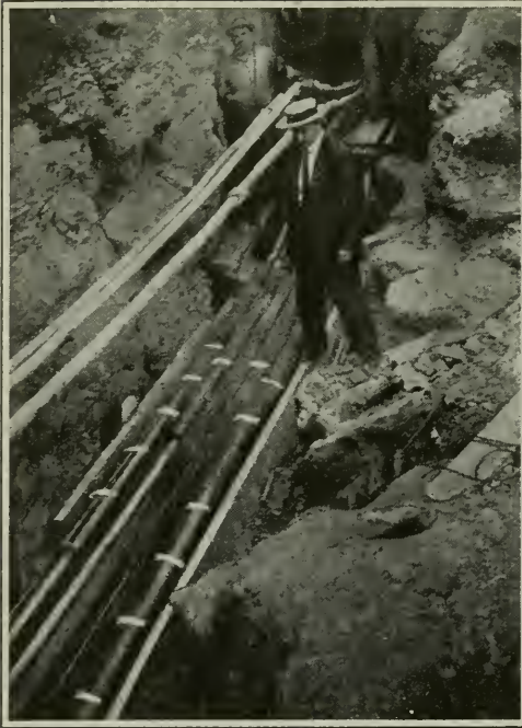
Laying the cables into split ducts without cutting or drawing through conduits as usual. The ducts used were the usual vitrified clay, but before baking they were scored inside and out, and easily split open by the brick-layer
