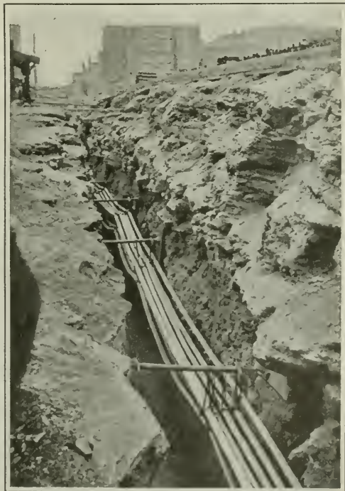
Cables systematically arranged and hung in the trench preparatory to being lowered into the split ducts
