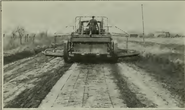
Two treatments of the roadway during the season keep it in excellent condition
