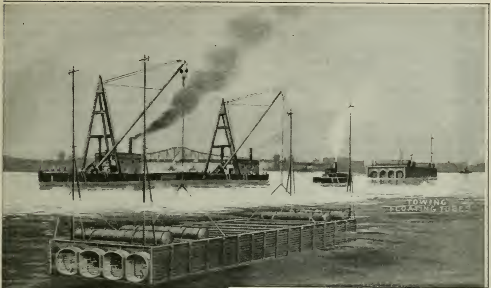
The great tunnel sections seem to float in the water as easily as though they were of wood. Four sections, when floated to their positions, weighed seven hundred and fifty tons
