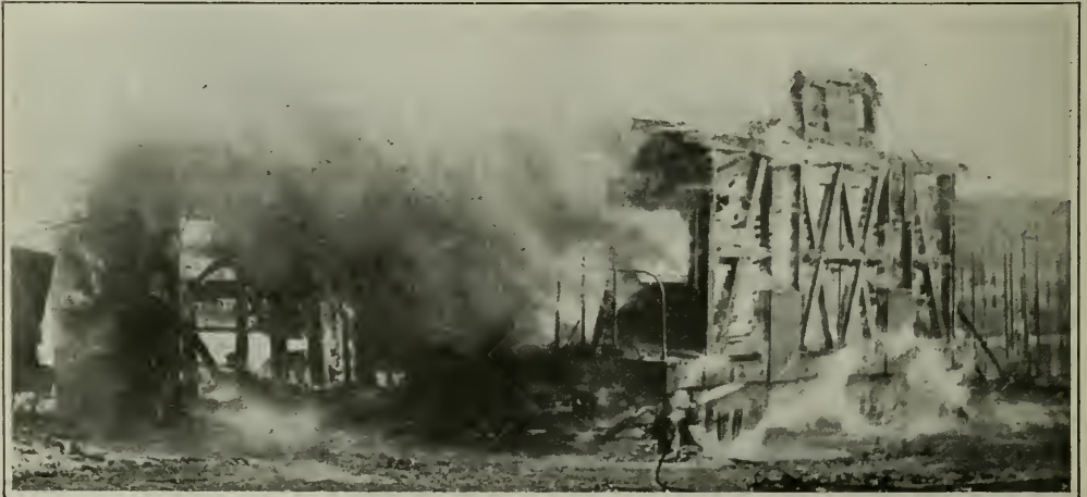
By burning its old wooden cars a railroad company saves $2,000,000 a year in labor formerly spent to repair the cars. Before setting fire to the cars, all usable fixtures are removed. After the fire, the remaining scrap iron is sold
