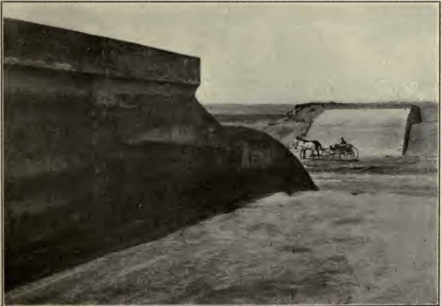
FIG. B.—Concrete inverted siphon carrying water of main canal under side drainage line instead of over it. North Platte Project, Wyo.-Nebr.
