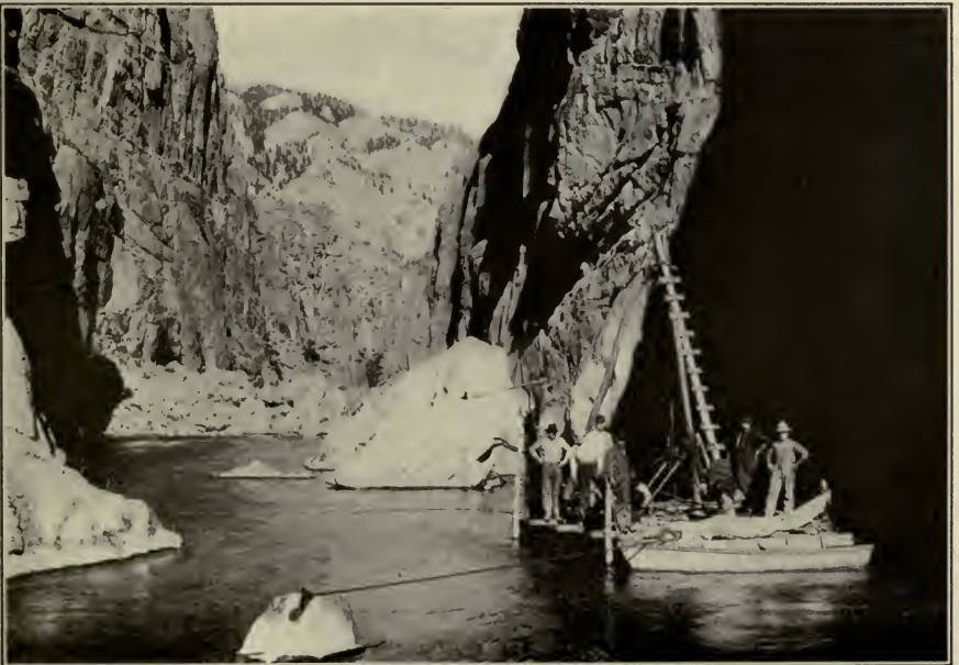
FIG. B.—Drilling for bed rock at storage dam site. Shoshone Project, Wyo. (Facing Page 192)
