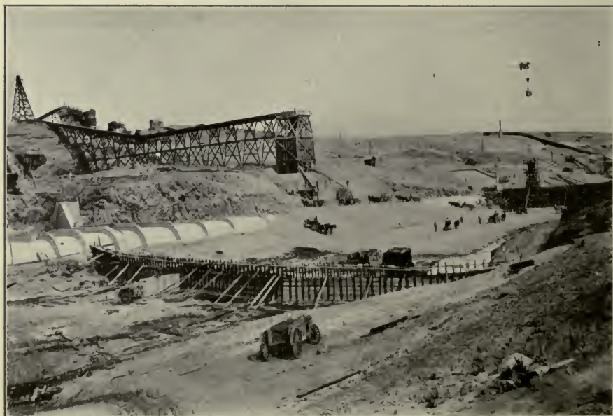
FIG. D.—Foundations for Lahontan Dam, Nev.; showing concrete conduit, conveying water through lower part of dam, with conveying plant in background.
