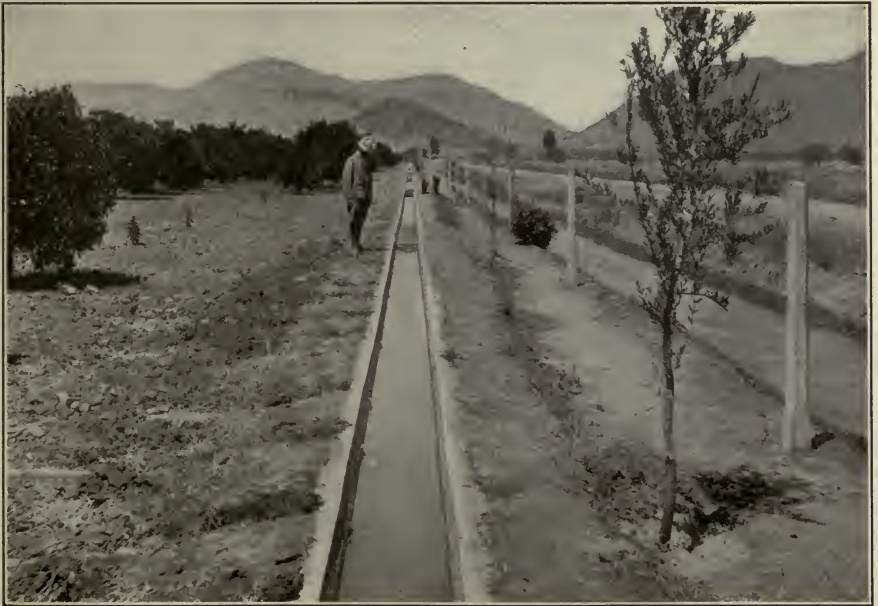
FIG. B.—Distributary lined with concrete to reduce loss of water and prevent development of alkali.
