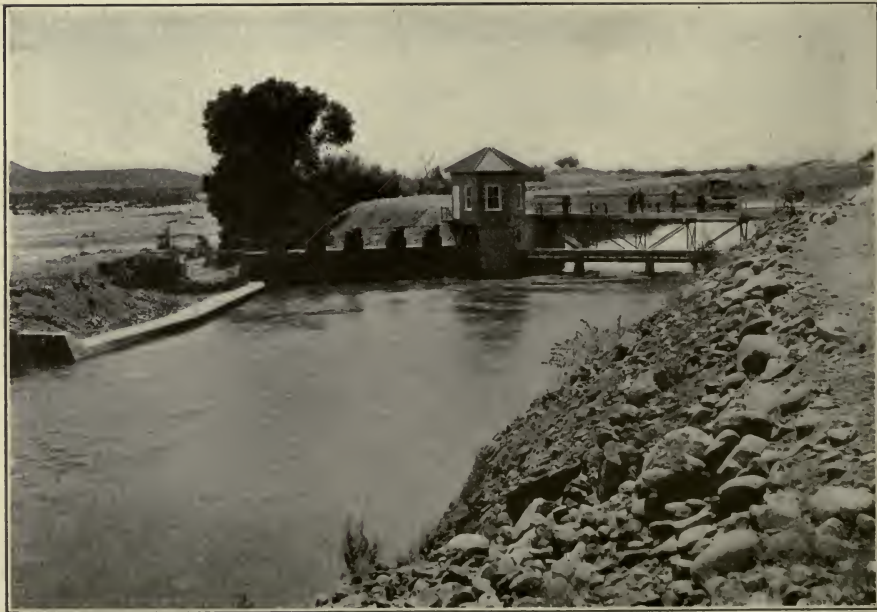
FIG. D.—Spillway lip to automatically permit escape of excess water from canal back into river and sluice gates provided to facilitate scouring out of materials deposited in upper portion of canal. Salt River Project, Ariz.
