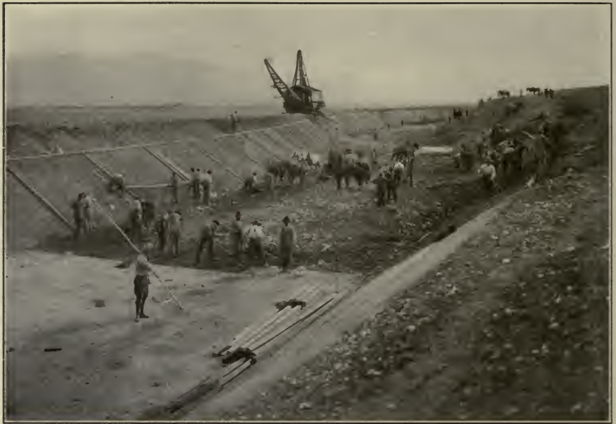
FIG. C.—Lining canal with concrete to increase the capacity, and reduce the seepage. Boise Project, Idaho.
