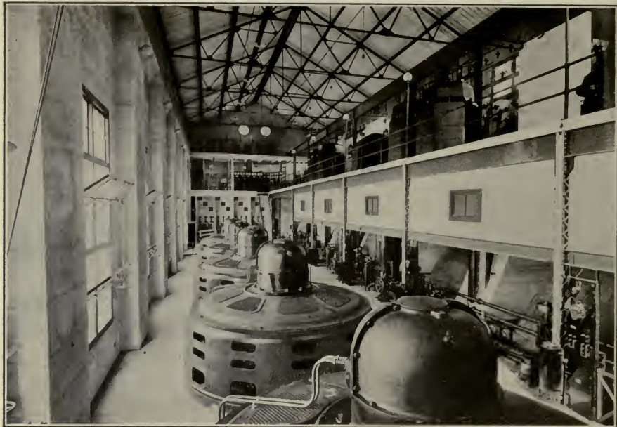
FIG. C.—Generators driven by water power furnishing electrical energy for pumps. Minidoka Project, Idaho.
