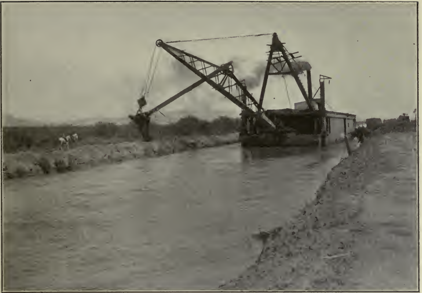
FIG. A.—Enlarging canal by means of floating dipper dredge. Salt River Project, Ariz.
