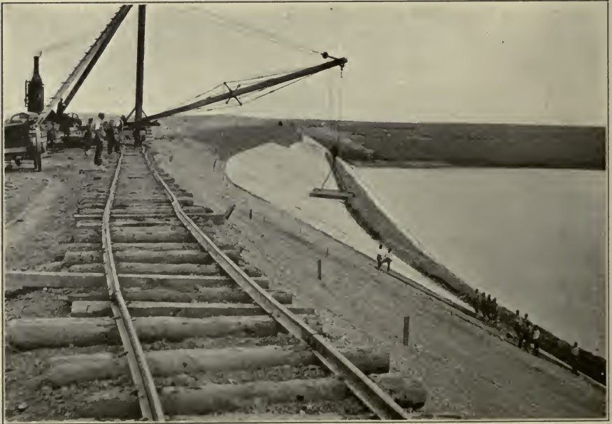
FIG. D.—Concrete block protection against wave action on earth dam. Belle Fourche Project, So. Dak.
