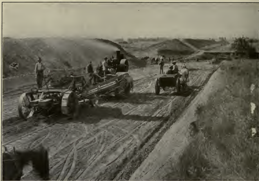
FIG. C.—Excavating canal by use of excavator with belt conveyor, drawn by traction engine. Belle Fourche Project, So. Dak.
