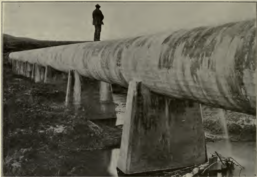
FIG. C.—Concrete pressure pipe used in place of flume. Sun River Project, Mont.
