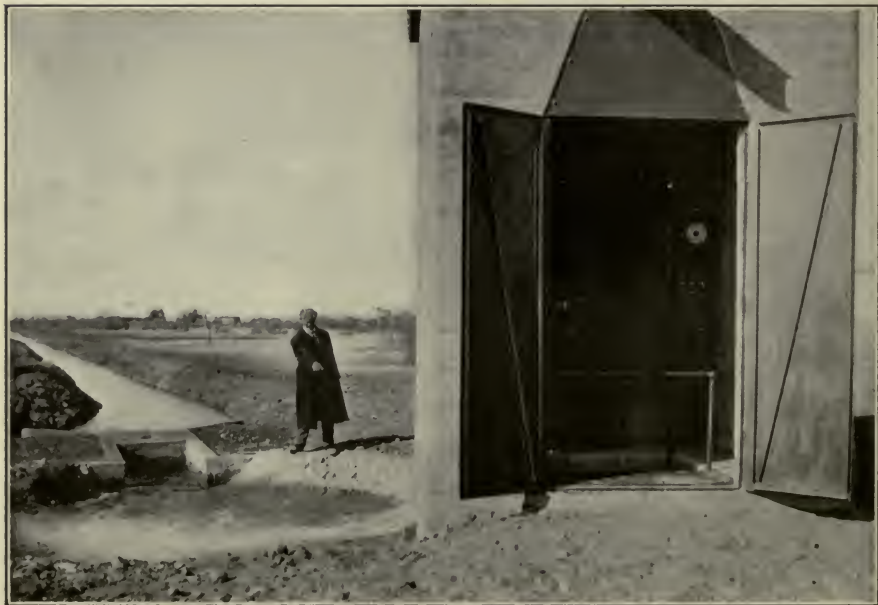
FIG. D.—Electrically operated centrifugal pumps delivering water to laterals on Gila River Indian Reservation, Ariz.
