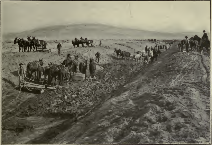
FIG. A.—Constructing canal in earth by means of four-horse Fresno scrapers. Minidoka Project, Idaho.
