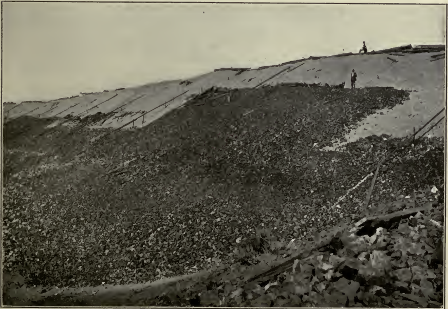
FIG. B.—Loose rock protection of earth dam on water side. Umatilla Project, Ore.
