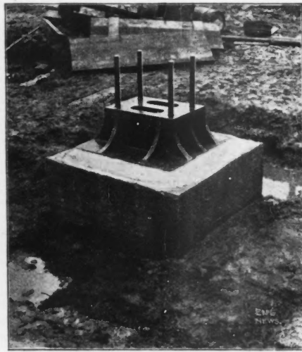
Fig. 3.—Column Foundation, Boston Elevated Railway, Showing Shoe and Holding-Down Bolts in Place.
