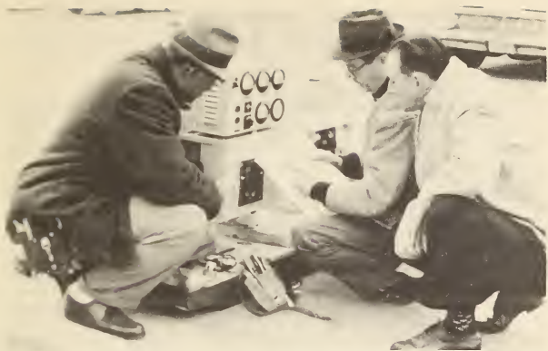
The Chief Building Engineer and two helpers of the PDH operating site carefully examine wiring and operating plan for hospital's generator during Packaged Disaster Hospital training exercise.
