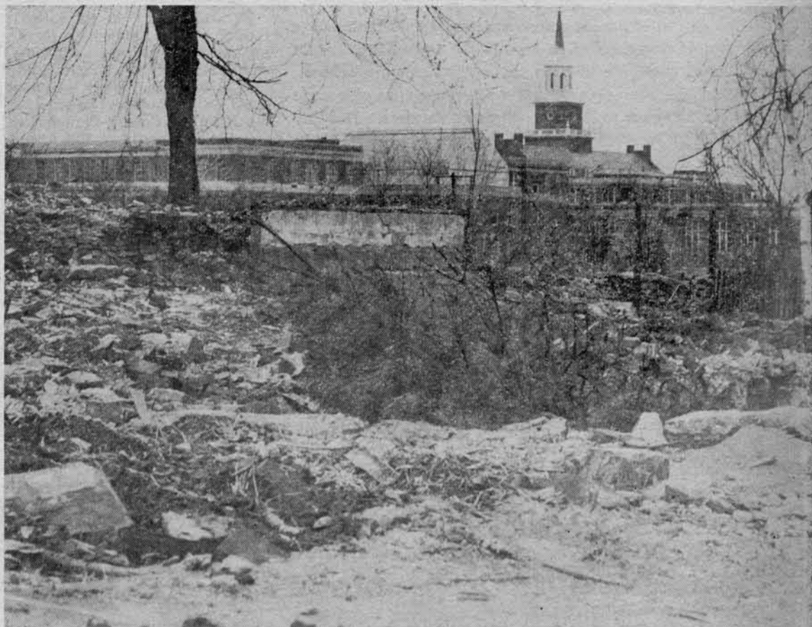
Buildings begin coming down on Calhoun Street as the University's construction plans proceed.
