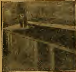
Spraying roof deck of box car with Carbosota Creosote Oil (no paint used).
