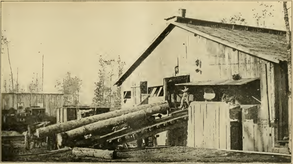
SNAGING BIG LOGS, THREE AT A TIME, IN A BIG SAWMILL OPERATED BY THE AMERICAN FORESTRY ENGINEERS AT ST. DOZIER ON THE MARNE
