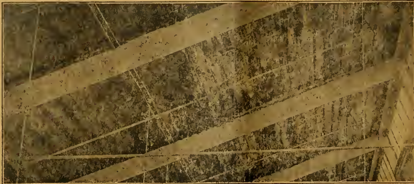
Roof planks of weave shed of textile-mill destroyed by decay in nine years. (Courtesy F. J. Hoxie, eng., Associated Factory Mutual Fire Insurance Cos., Boston.)
