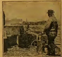
Spraying: Applying Carbosota to ends, mortises, and tenons (points of contact) of ceps and stringers for trestle.
