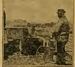
Spraying: Applying Carbosota to ends, mortises, and tenons (points of contact) of logs and stringers for track.
