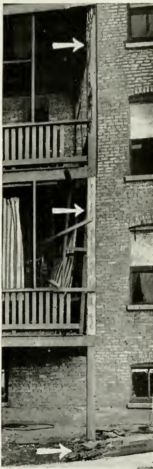
Replacement of porch columns and joists in framing of three floors is an annual occurrence at most apartment houses of this type.
