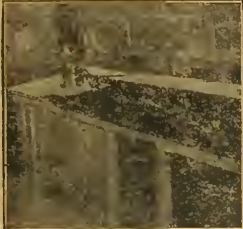
Spraying roof deck of box car with Carbosota Creosote Oil (no paint used).
