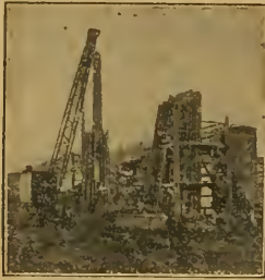
Commercial Plant for Creosoting Poles by The Open-Tank System. Western Wood Preservers, Sandpoint, Idaho. (W. C. Assoc.)
