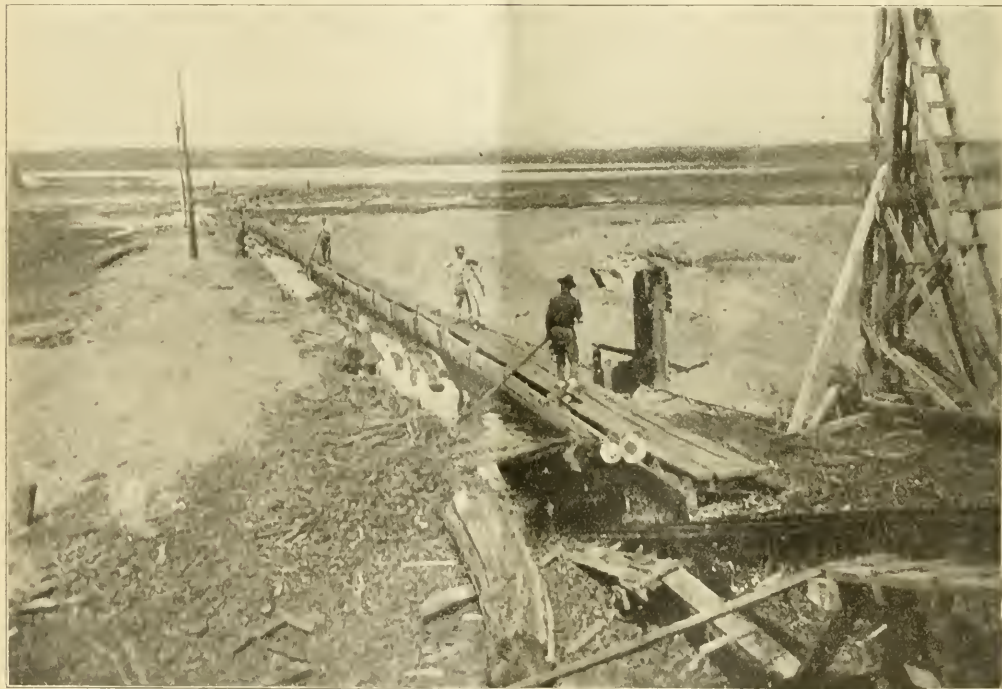
CANAL AND CAR BRINGING LOGS UP TO THE HOIST INTO THE AUREILLIAN MILL OF THE 20th ENGINEERS NEAR PONTENX, LANDES, FRANCE
