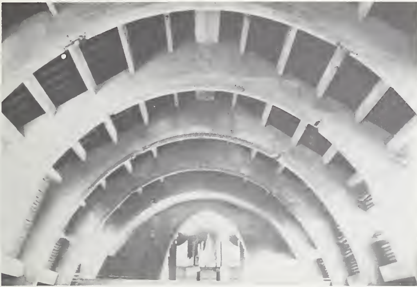
Figure 46-5 Cracking in arches of chapel, Instituto Pedagógico.
