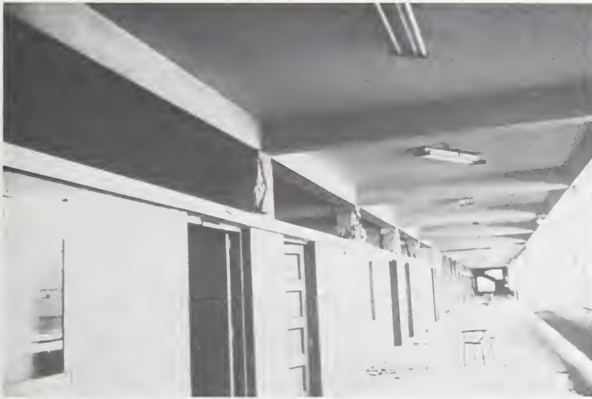
Figure 38-1 Sheared columns above partial height wall, Instituto Nacional Ramirez Goyena.
