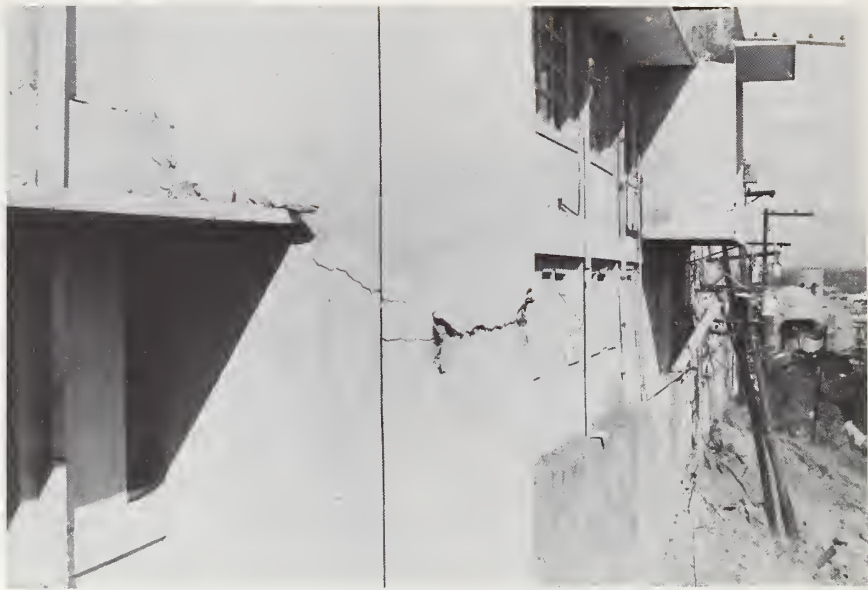
Figure 60-5 Cracking of walls at rear of building, Casa Presidencial.
