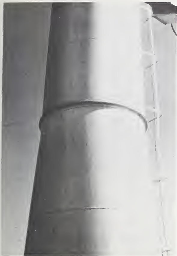
Figure 22-3 Cracked weld in stack, Planta Electrica ENALUF.
