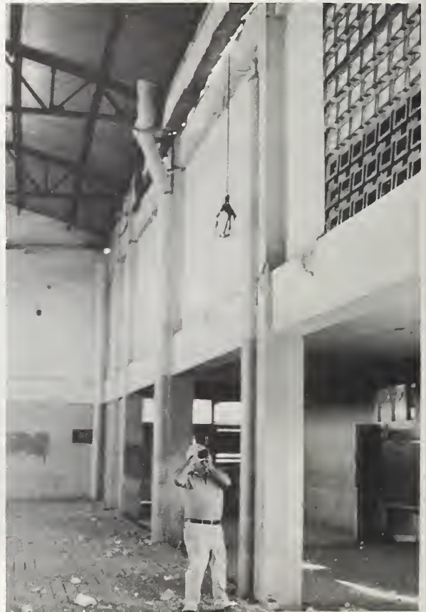
Figure 38-4 Broken wall on south side of gymnasium where school wing connects, Instituto Nacional Ramirez Goyena.
