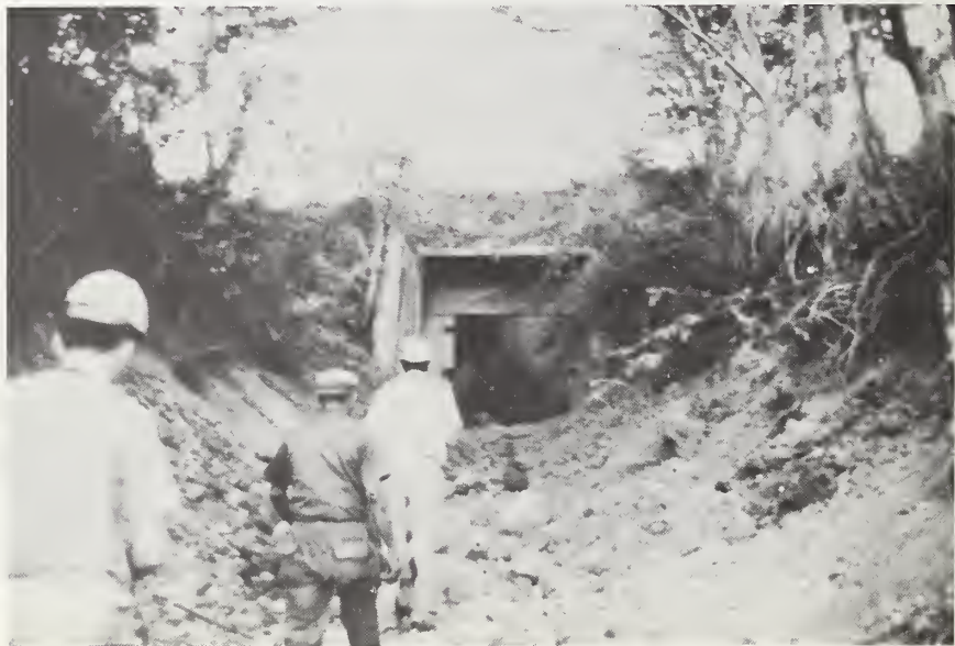
Figure 57-3 Wing wall collapsed at right of entrance, Bodegas de Almacenamiento de y Morocon.
