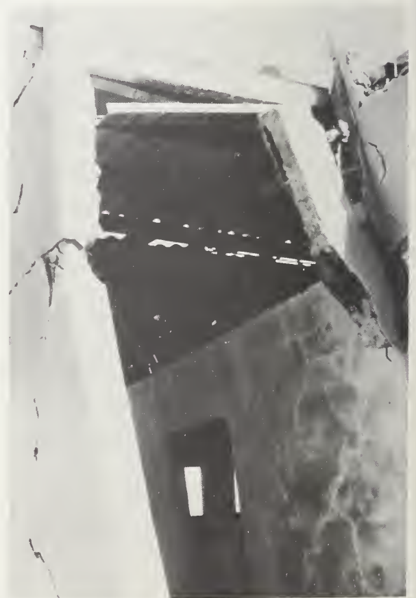
Figure 16-2 Damage from movement of inadequately braced roof, INCEI laboratory.
