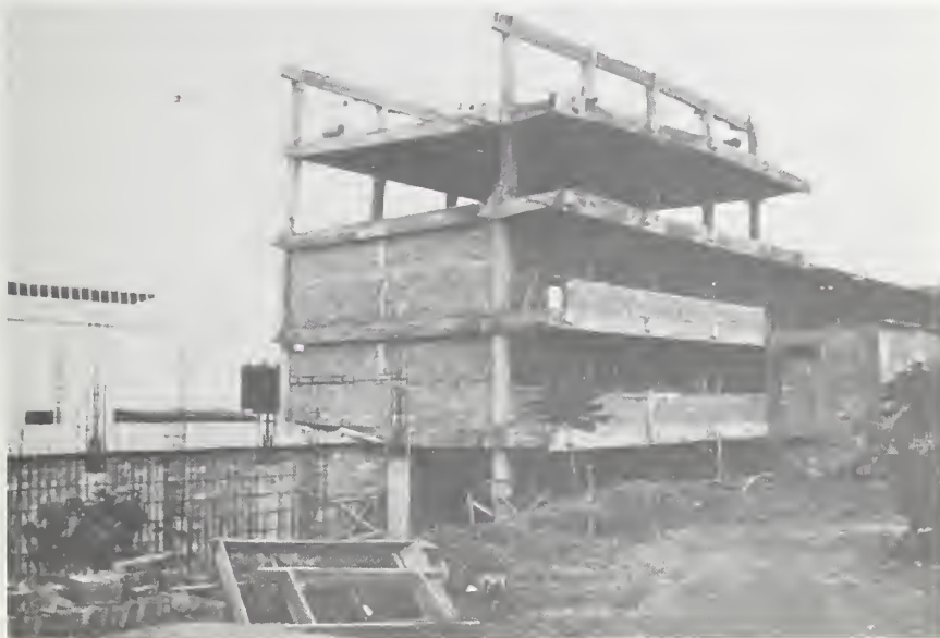
Figure 53-4 Frame failures in building under construction, Seminario Catolico.
