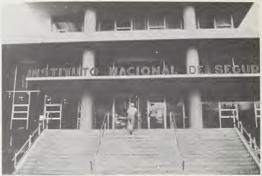
Figure 44-1 Main entrance to nine story frame showing absence of structural damage, Edificio Administrativo INSS.
