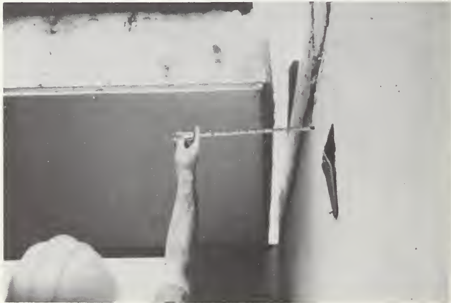
Figure 24-4 Unfastened roof channel in duplex unit, Bello Horizonte.
