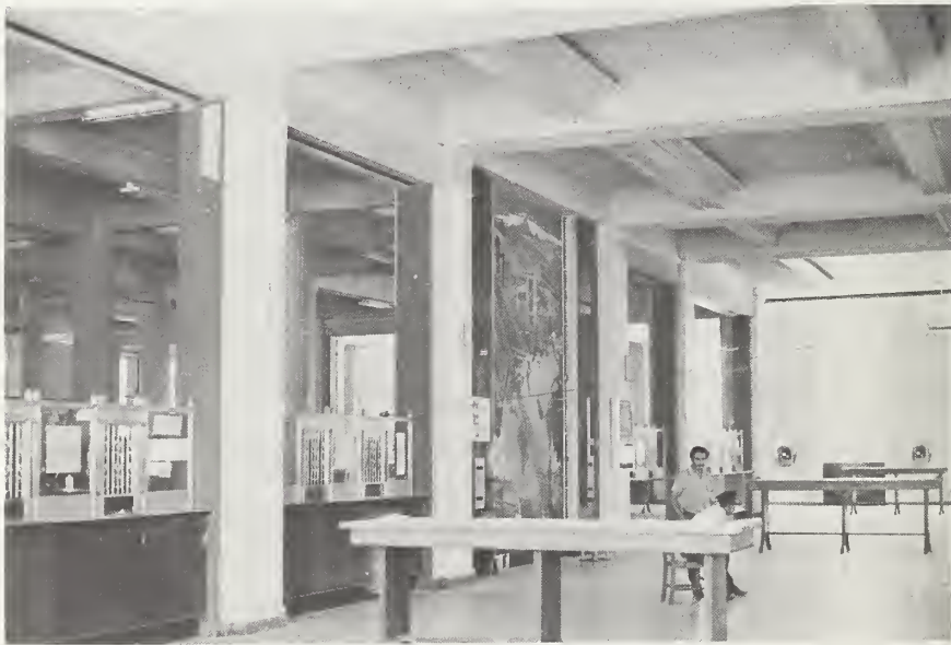
Figure 5-2 Main floor with light cracking of columns and damage to infilled mural, Palacio de Comunicaciones.
