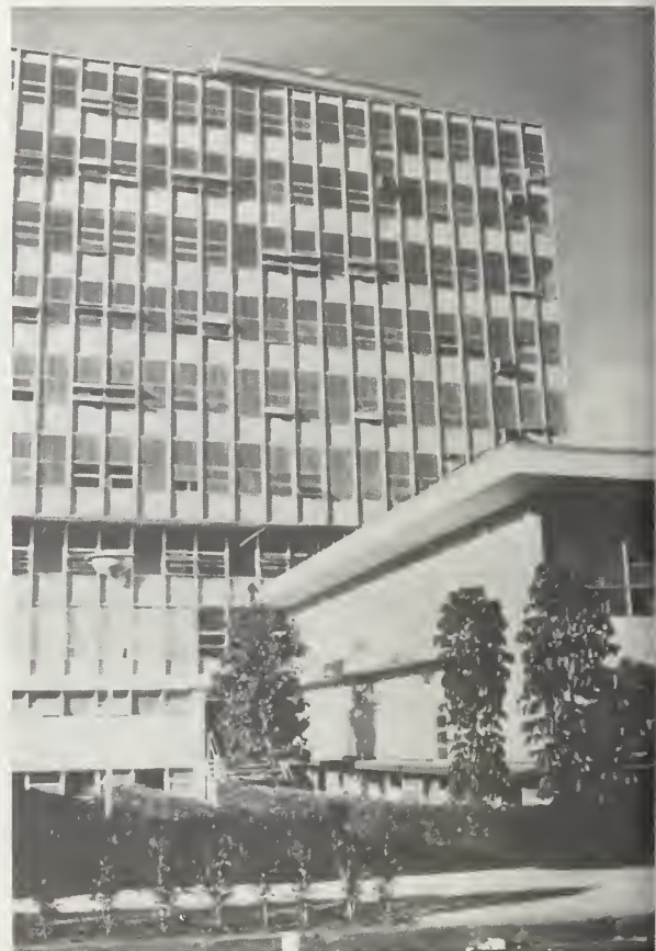
Figure 44-2 Facade shows limited nonstructural damage and collapsed mechanical penthouse, Edificio Administrativo INSS.
