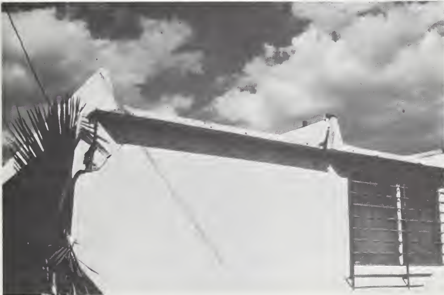
Figure 24-2 Cracking in walls at attachment of roof channel, Bello Horizonte.
