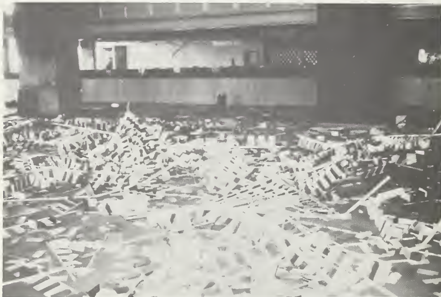
Figure 52-4 Suspended ceiling fallen to floor of main lobby, Banco Central.
