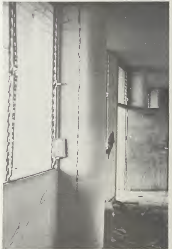
Figure 46-4 Cracking of columns, Instituto Pedagogico.
