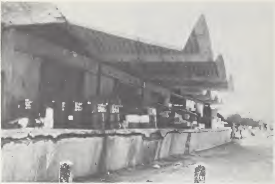
Figure 68-3 General view of damaged barrel shed, Aduana General de Managua.
