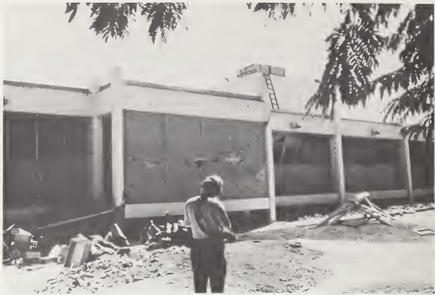
Figure 16-1 Severely damaged modern reinforced concrete frame building, INCEI administration building.
