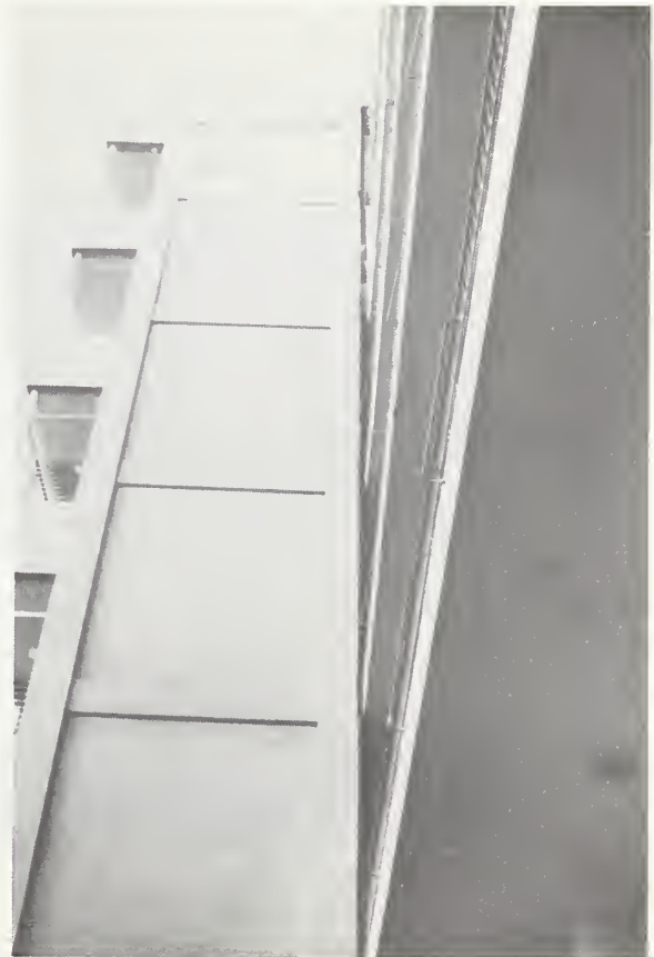
Figure 46-2 Displacement of building and cracking of slabs, Instituto Pedagógico.
