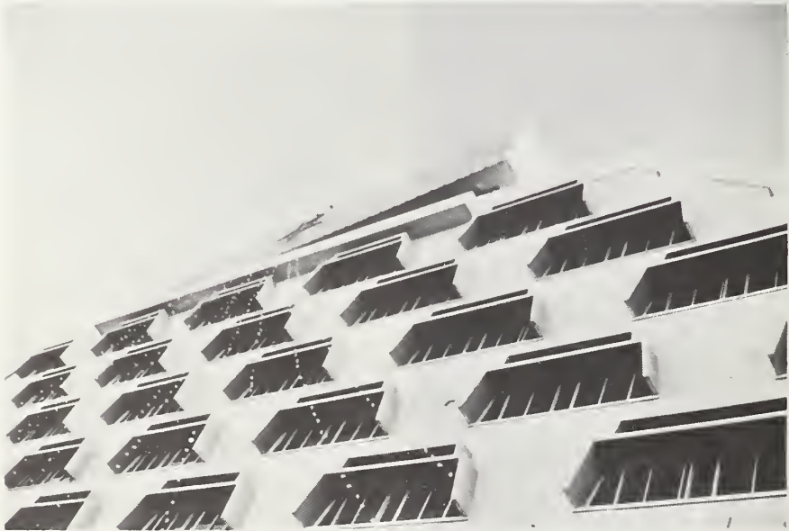
Figure 42-2 Minor facade cracking and displacement of mechanical penthouse, Hotel Intercontinental.
