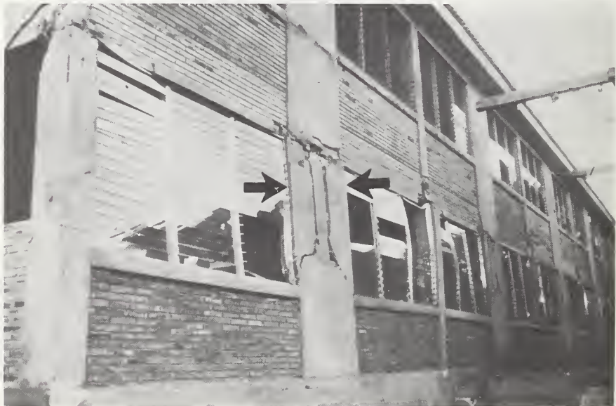
Figure 35-5 Arrows show masonry piers on either side of reinforced concrete columns were ineffective, Centro Escolar Simon Bolivar.
