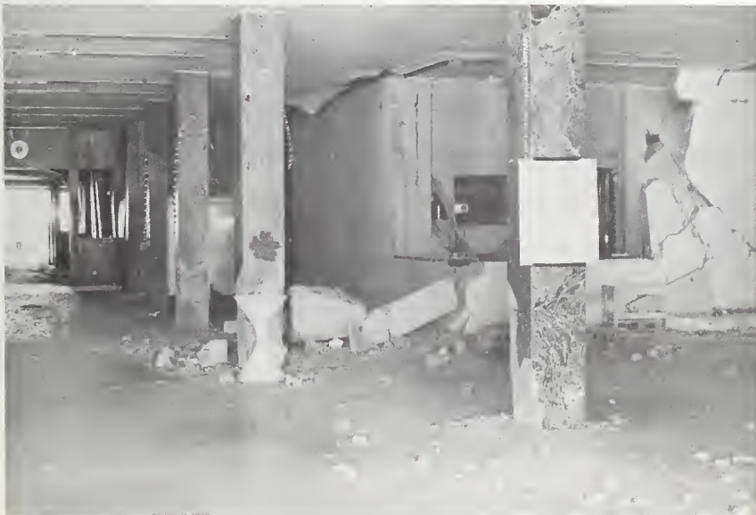
Figure 55-6 Interior view at main entrance, only nonstructural damage apparent, Hospital General El Retiro.
