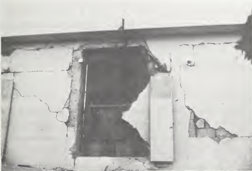
Figure 4-4 Wall and column damage in market building, Mercado Periferico Oriental.
