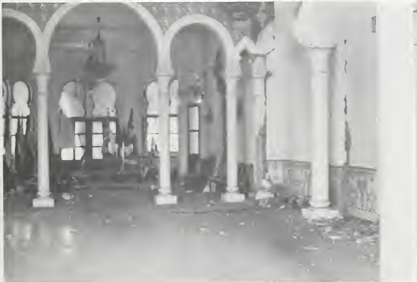
Figure 60-4 Interior damage in main lobby, Casa Presidencial.
