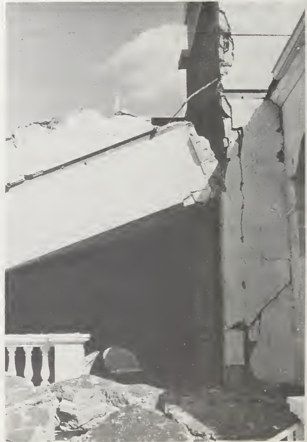
Figure 60-2 Detail of collapsed terrace roof, Casa Presidencial.
