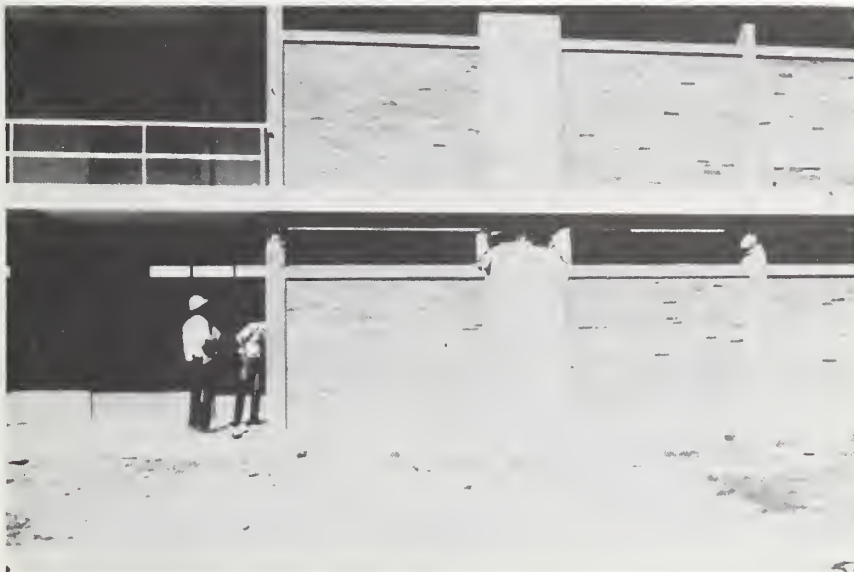
Figure 35-3 Sheared columns above infill wall, Centro Escolar Simon Bolivar.
