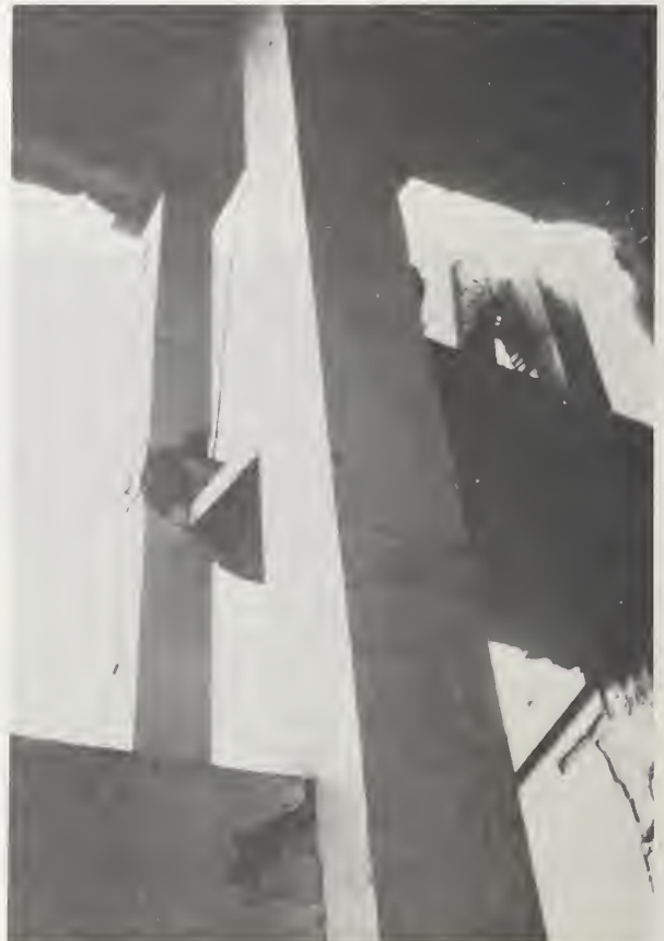
Figure 53-2 Damaged framing of gymnasium, Seminario Catolico.
