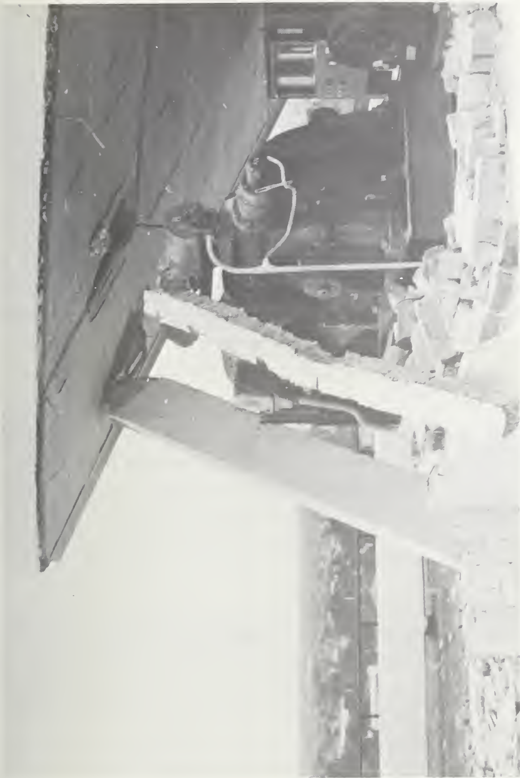
Figure 44-3 Collapsed mechanical penthouse, Edificio Administrativo INSS.
