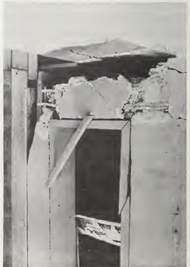
Figure 25-2 Failure of bond beam and column near aperture, note inadequacy of anchorage of reinforcement at corner.
