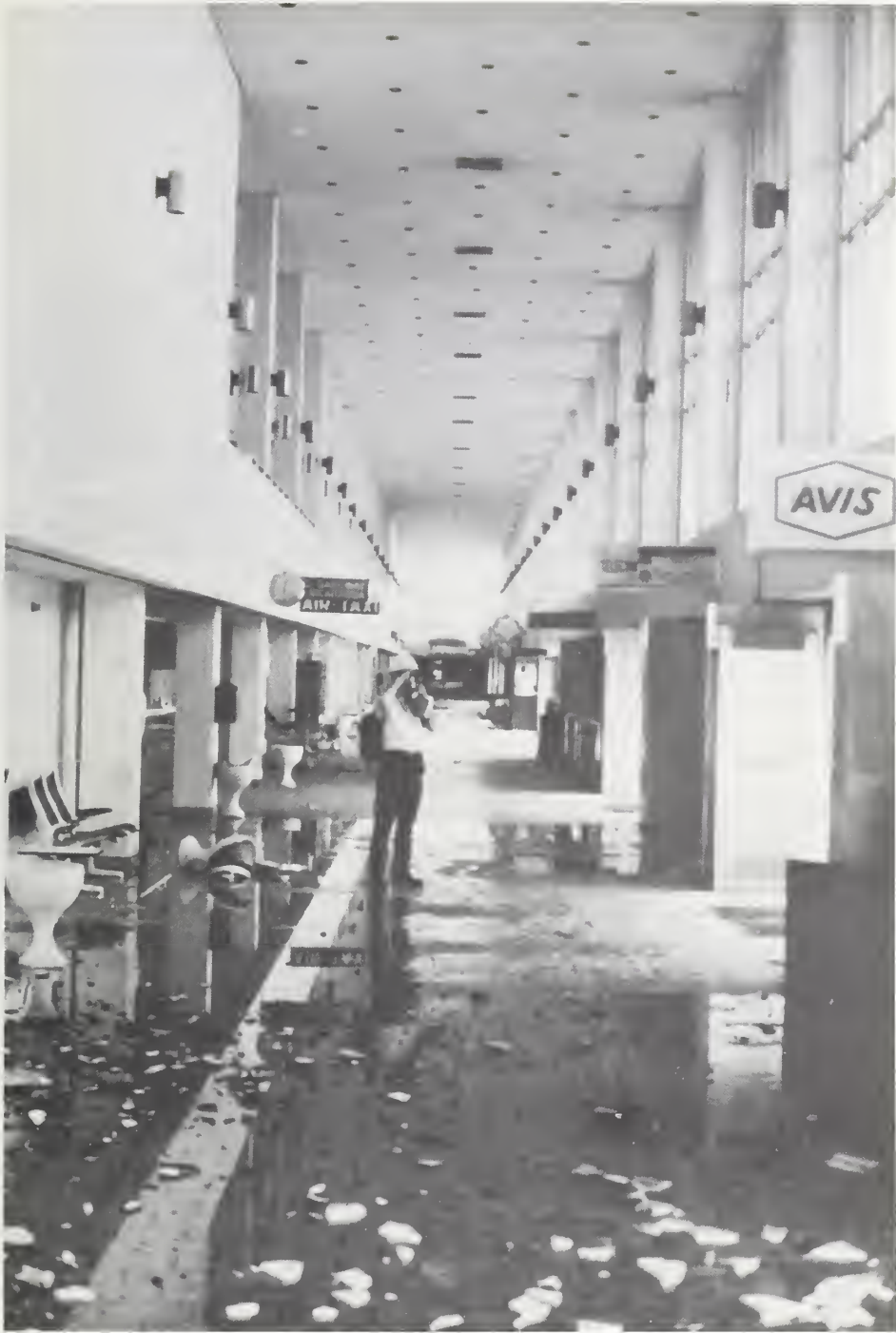
Figure 13-1 Aisle on the ground transportation side showing superficial damages, Terminal de Pasajeros Aeropuerto Internacional.
