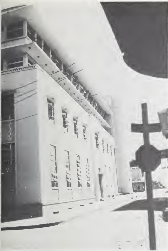
Figure 5-3 Side of the Palacio de Comunicaciones, note the tottering fourth floor walls and roof.
