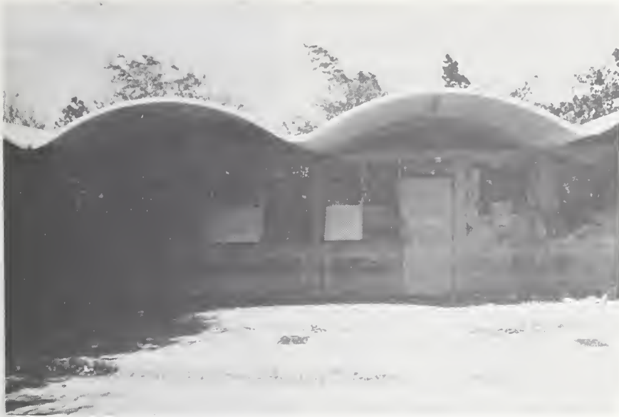
Figure 53-3 Severely damaged columns supporting shell roof, Seminario Catolico.
