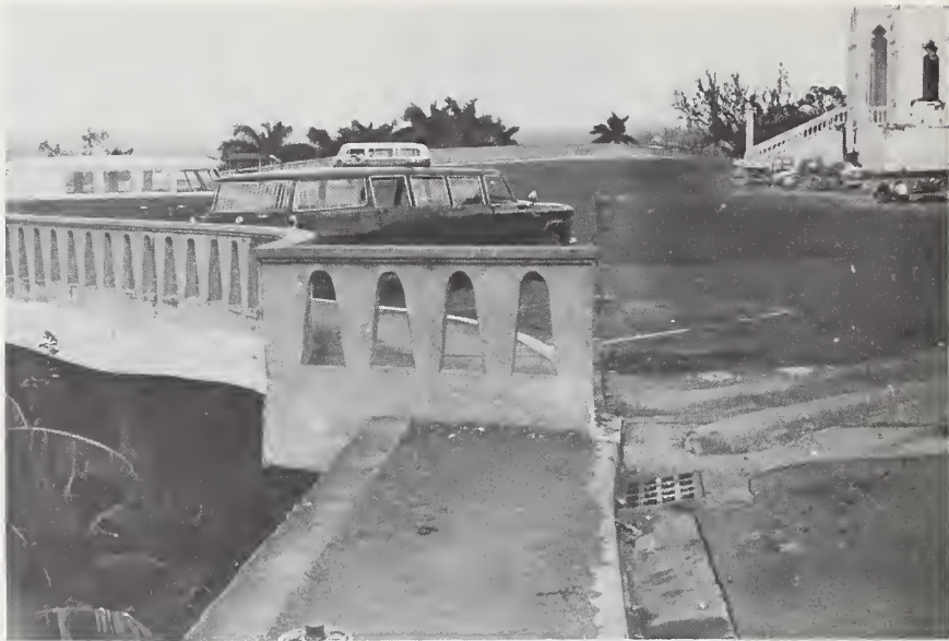
Figure 57-2 Cracking in road in front of house above retaining wall of the Storeroom of the Pines, Casa Presidencial.
