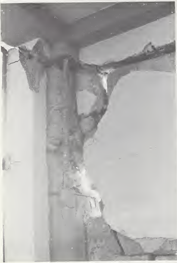
Figure 4-1 Column failure at construction join in nursery building, Mercado Periferico Oriental.
