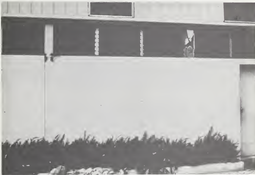
Figure 72-4 Column damage caused by partial height infill wall, IBM building.
