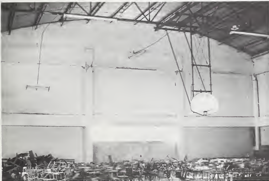
Figure 38-6 Shear of columns at west wall of gymnasium, Instituto Nacional Ramirez Goyena.
