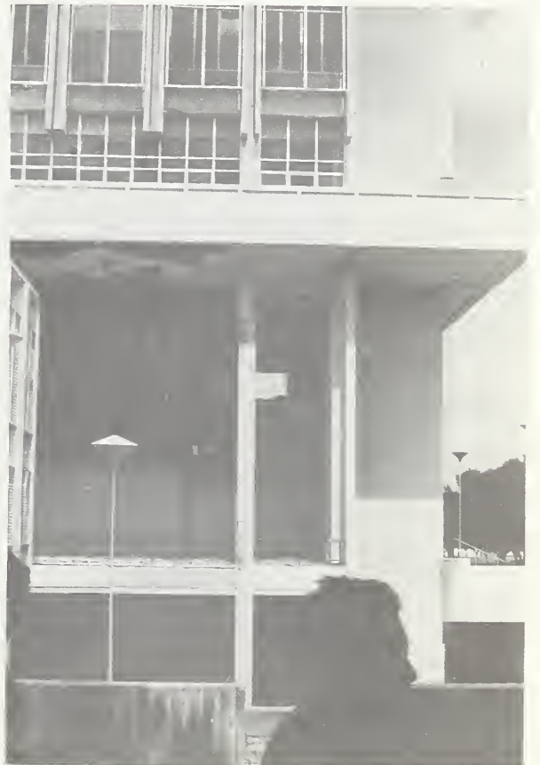
Figure 43-3 Nonstructural damage on 6 story wing, Corte Suprema de Justicia.
