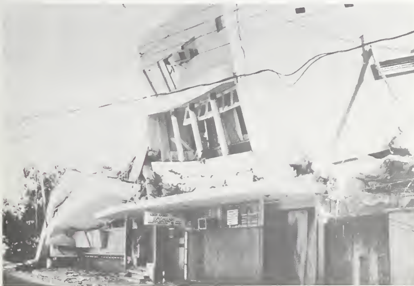
Figure 74-2 Three of five stories of the Edificio Guerrero Pineda standing at this end.
