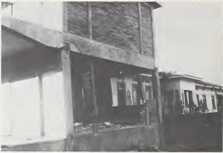
Figure 35-4 Fallen end wall and sheared columns, Centro Escolar Simon Bolivar.
