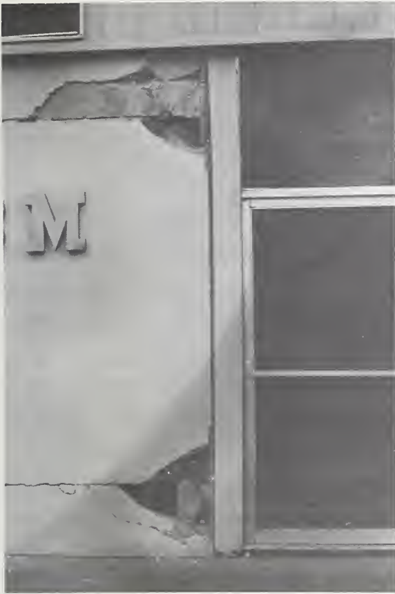
Figure 72-3 Column deformation at IBM building caused by cracked infill panel.
