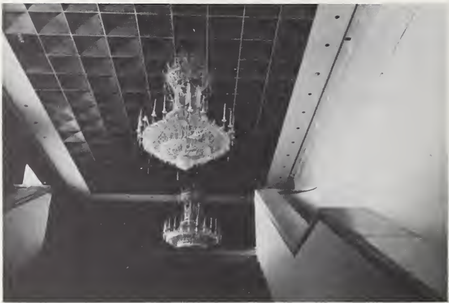
Figure 41-3 Minor finish damage amounted to fallen ceiling panels and some chips from the chandeliers, Teatro Ruben Dario.
