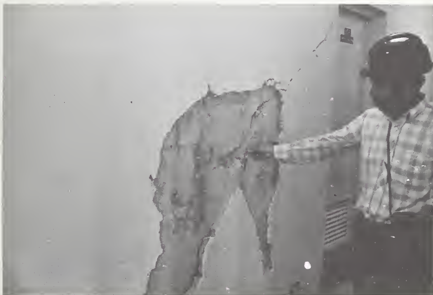
Figure 23-5 Cracking in shear wall on third floor, Edificio Administrativo ENALUF.
