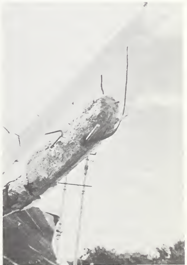
Figure 68-2 Close up of columns showing undeformed, lightly tied reinforcement, Aduana General de Managua.
