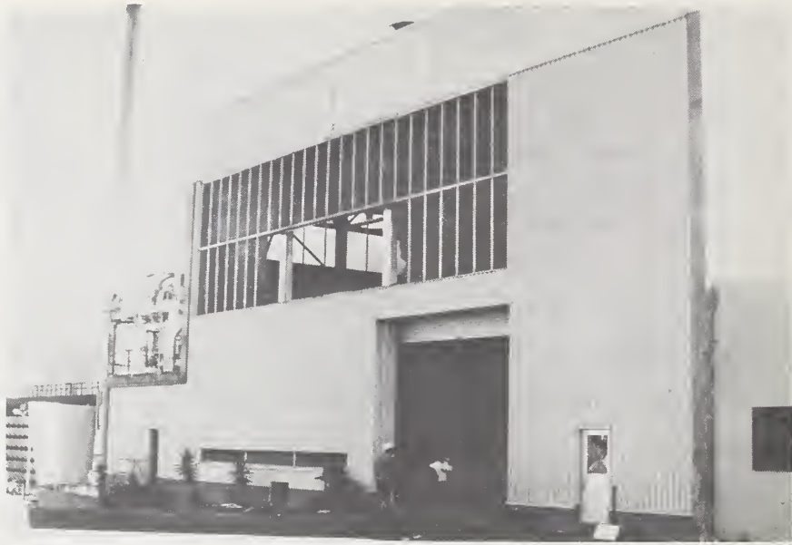
Figure 22-1 Only window damage notable in the main turbine building, Planta Eléctrica ENALUF
