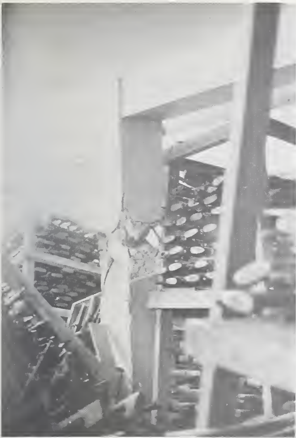
Figure 61-3 Column crushed in basement, Residencia Jefe Director.
