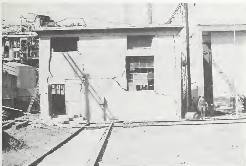
Figure 22-4 Severely damaged concrete block bearing walls of switch gear house at Planta Electrica ENALUF.
