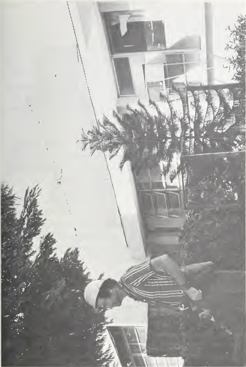
Figure 71-1 Cracked parapet walls, Policlínica Central del INSS.
