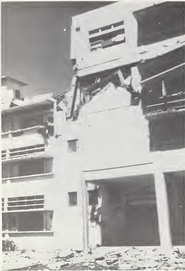
Figure 55-7 Third floor of the Hospital General El Retiro near collapse at rear.
