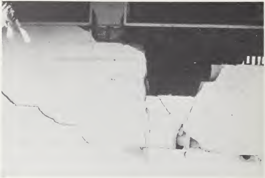
Figure 25-1 New damage over repaired cracks from the 1968 earthquake, Centro Escolar Salvador Mendieta.
