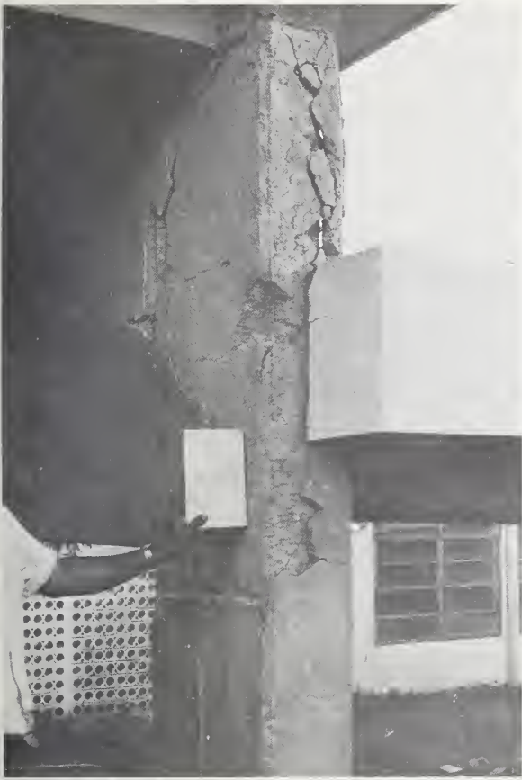
Figure 4-3 Damaged canopy columns at change of canopy elevation, Mercado Periferico Oriental.
