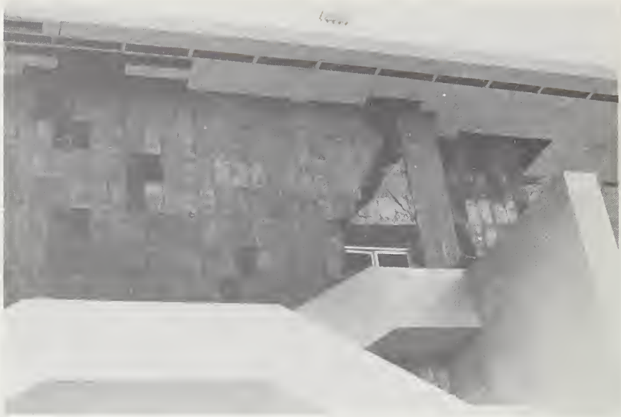
Figure 43-4 Extensive loss of exterior finish panels on 6 story wing, Corte Suprema de Justicia.
