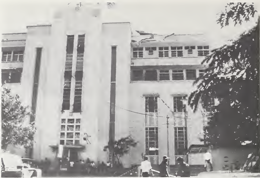
Figure 5-1 Front of the Palacio de Comunicaciones, limited damage except at fourth floor.
