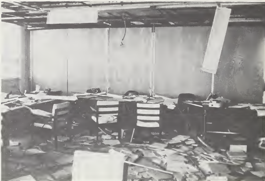
Figure 52-3 Nonstructural damage in an office, Banco Central.
