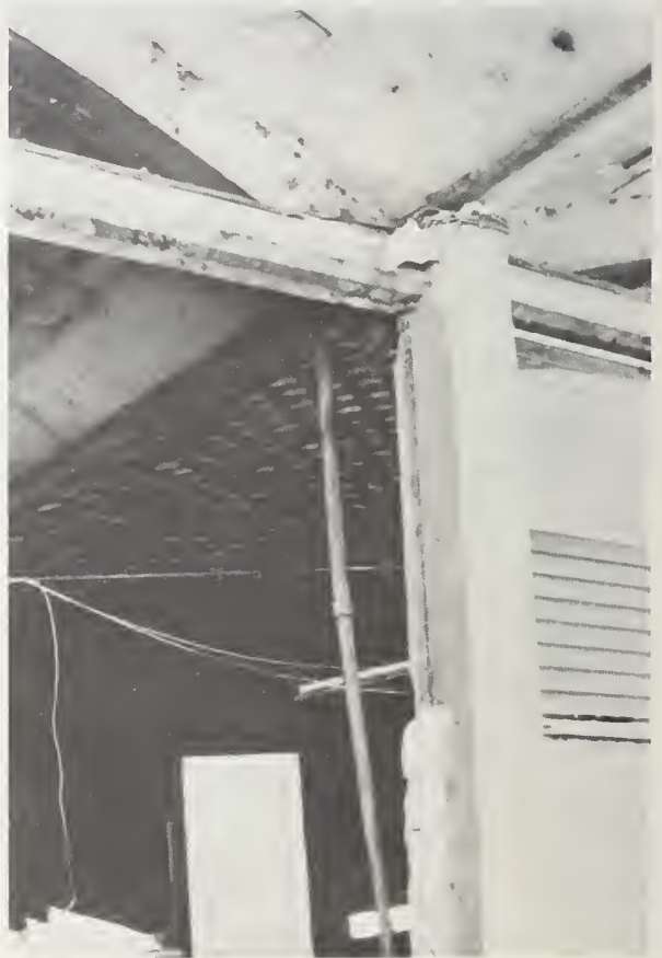
Figure 68-4 Close up of sheared exterior columns, Aduana General de Managua.
