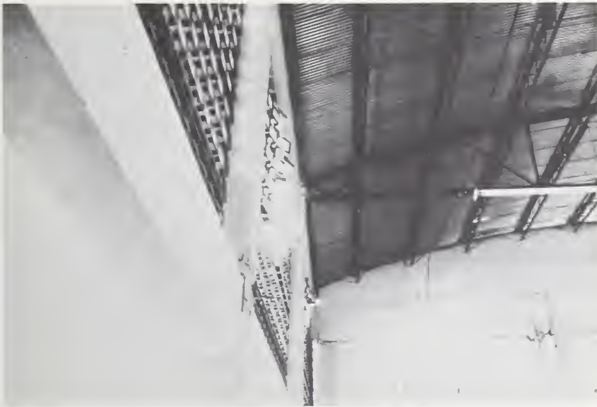
Figure 38-5 Lesser damage of south wall of gymnasium at more flexible west end, Instituto Nacional Ramirez Goyena.
