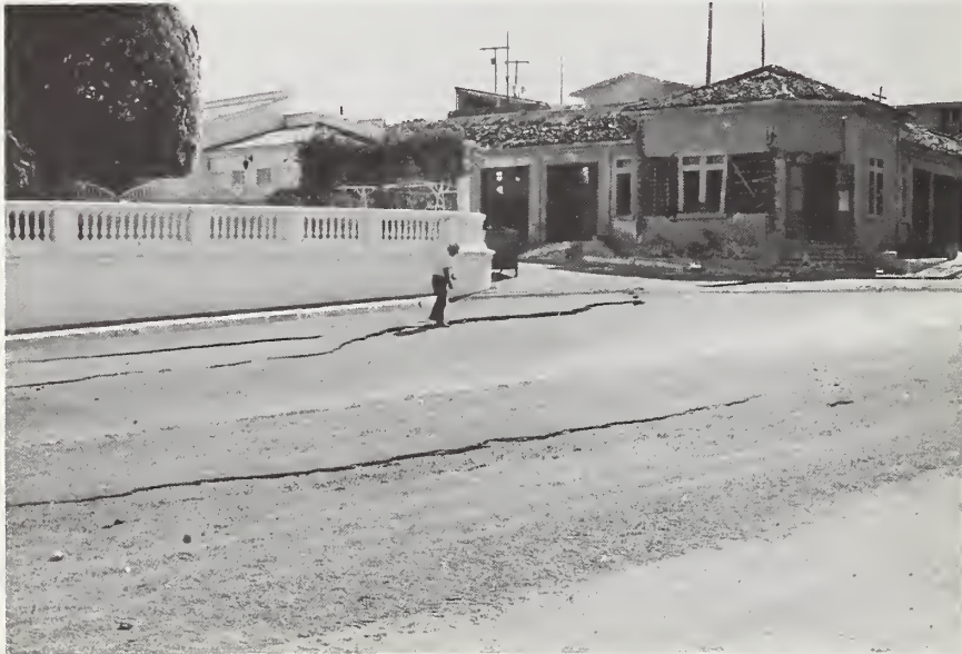
Figure 60-6 Subsidence cracking in road at northwest of Casa Presidencial.
