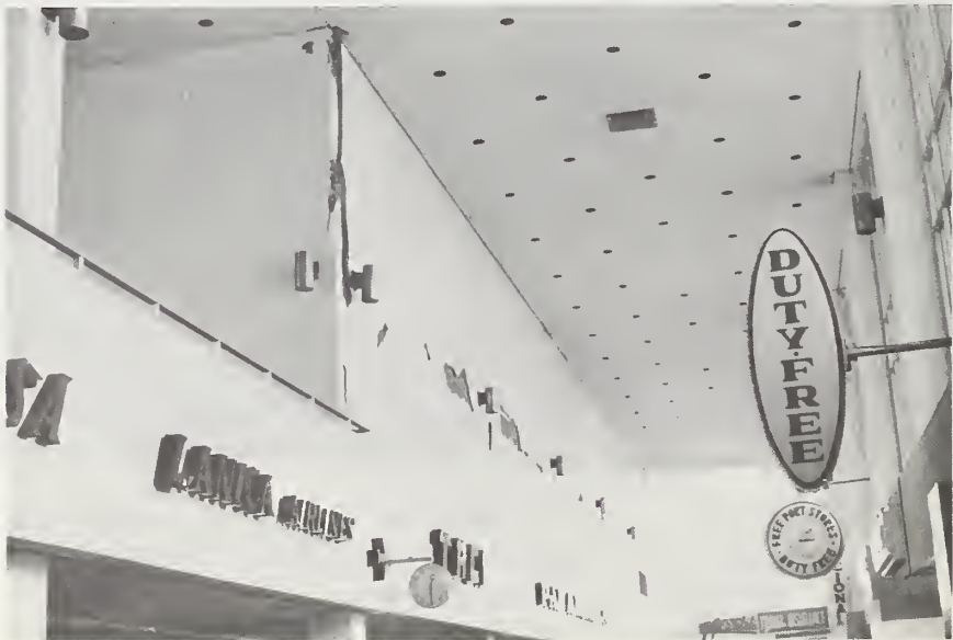
Figure 13-3 Overlaid curtain wall cracked at anchorage to frame, Aeropuerto Internacional.
