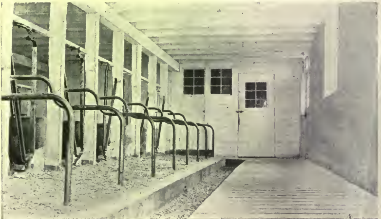
Fig. 97.—Side aisle of certified milk dairy transformed from old barn at small expense.
